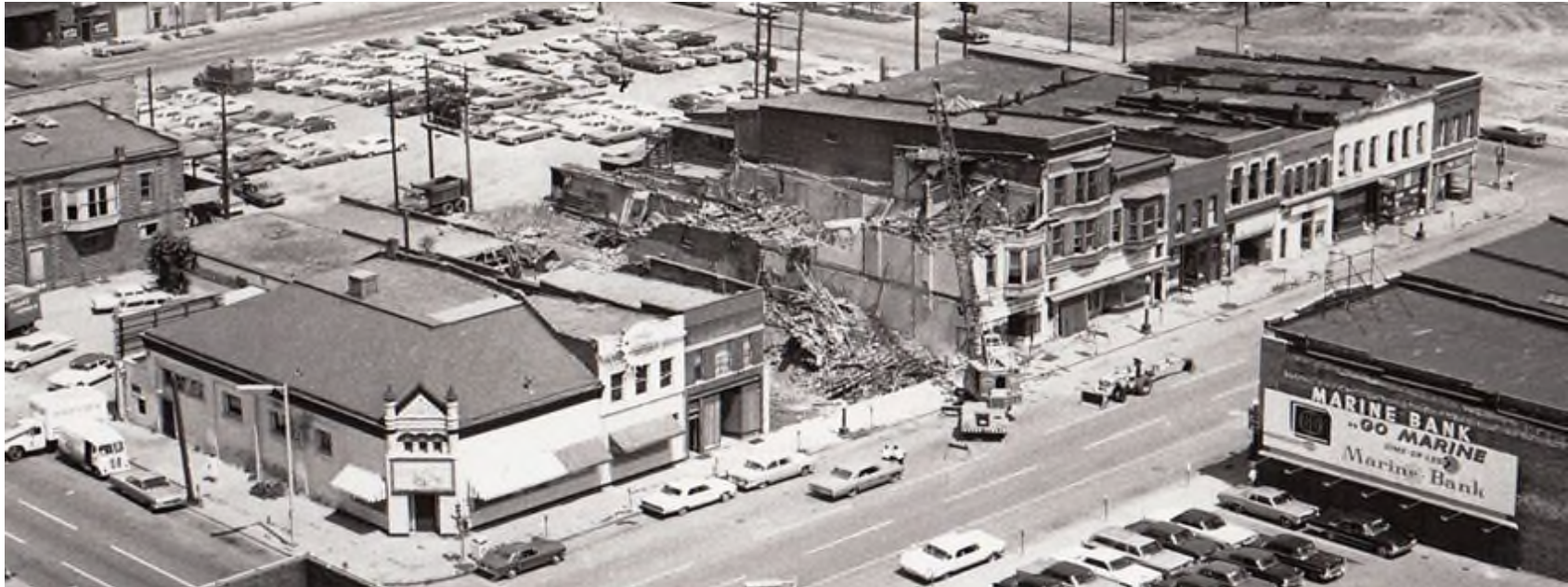
Figure 85. On May 18, 1966, the Illinois State Journal reported on the Springfield City Council’s award of a contract to Bartolo Excavating and Trucking Company for the demolition of 58 buildings in the “commercial urban renewal area” bounded by Washington Street on the south, Seventh Street on the west, Madison Street on the north, and Ninth Street on the east. In essence, this was the heart of the commercial district and social center for the black community—an area often referred to as the Levee. This picture, taken sometime shortly thereafter in the Spring of 1966, illustrates the work proceeding along the north side of Washington Street.
