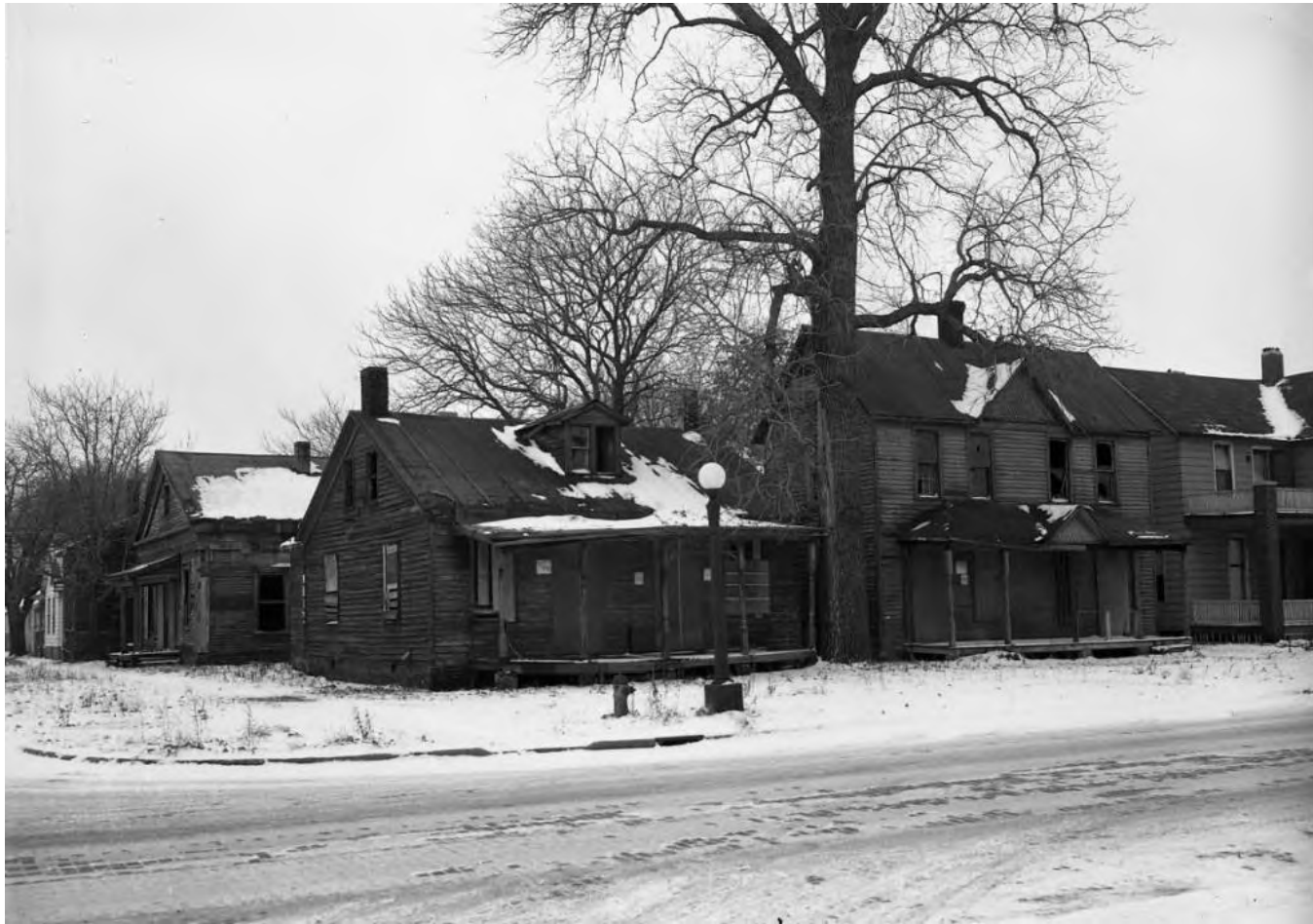
Figure 58. View of dilapidated houses located at Thirteenth and Adams Street, January 1965. By the middle 1960s, some landowners in the Central East Neighborhood had allowed their properties to decline, and the older housing stock in the neighborhood had begun to show signs of neglect. Large-scale demolition of properties in the area were undertaken in the years that followed (Mercury Studio Collections, Lincoln Library).
