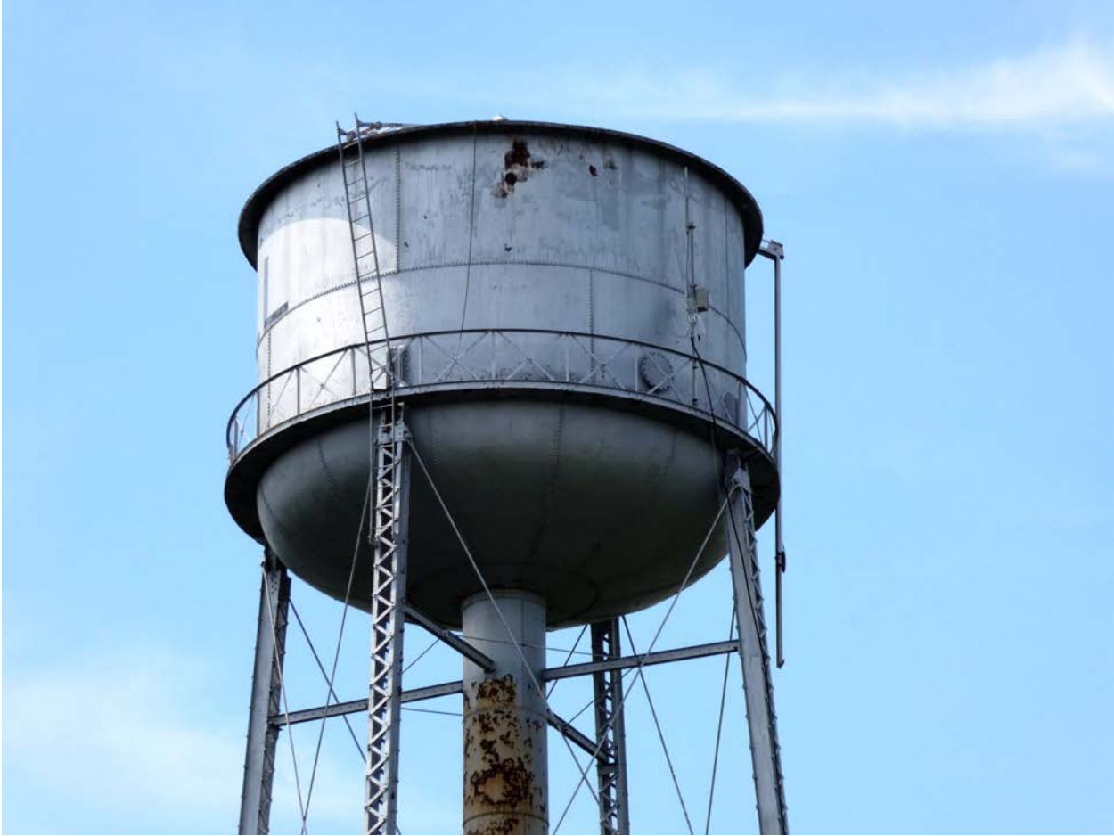
Figure 9. Detail view of storage tank, facing northwest.
