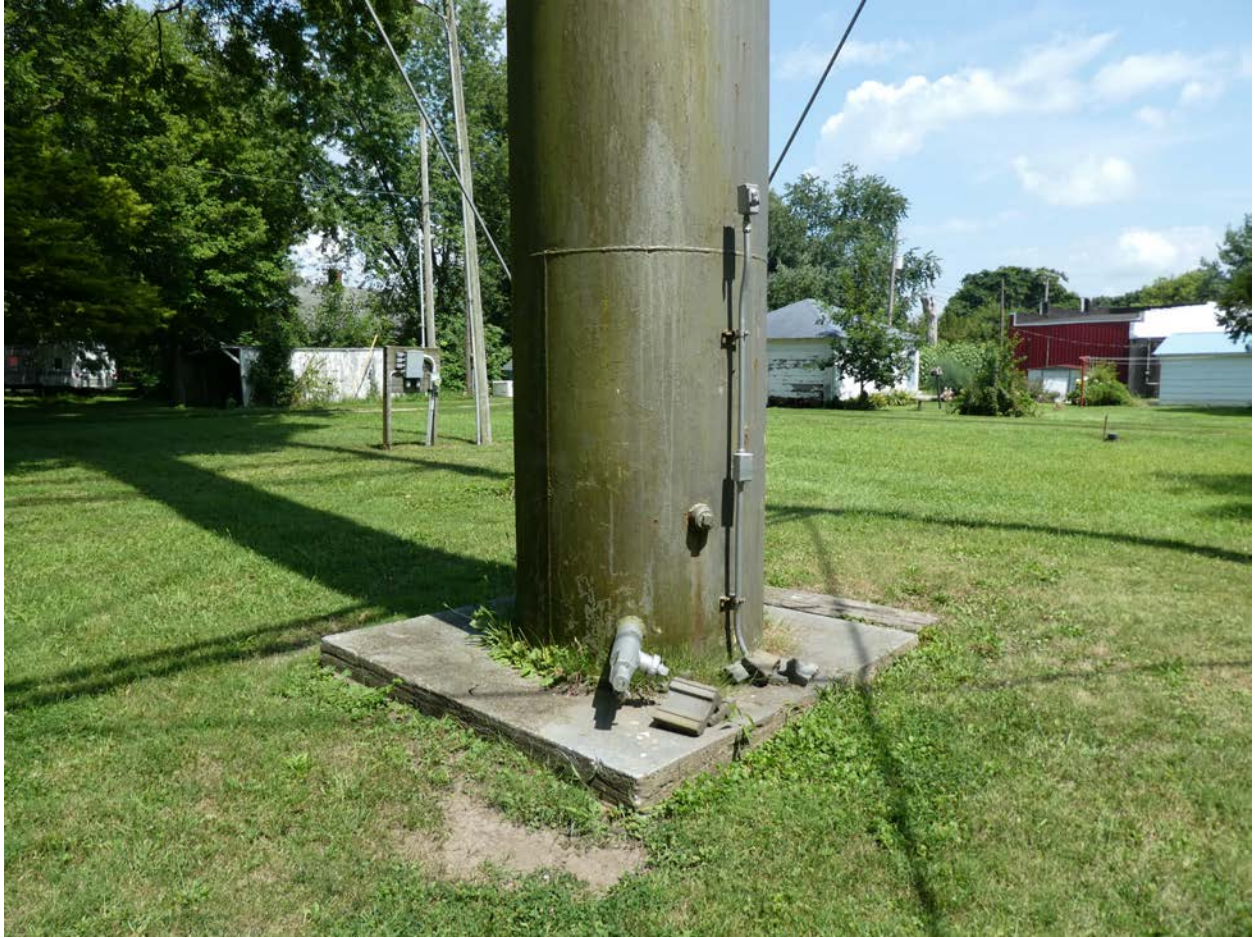
Figure 14. Detail view of uptake riser base and pressure release valve, facing northeast.
