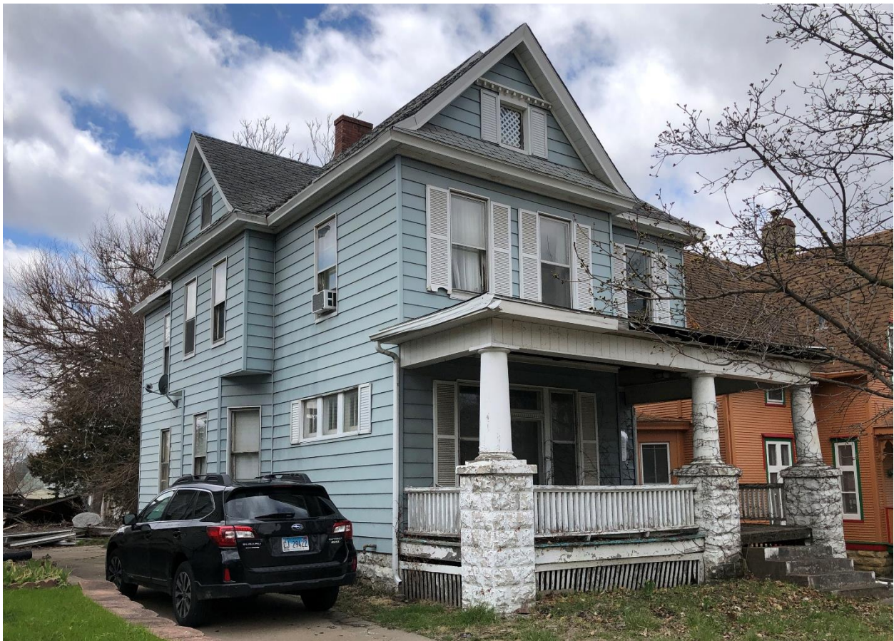
Photograph No. 1: View of the front (east) and side (south) façades of 1206 17 th Street looking northwest with a view of the collapsed historic automobile garage in the background.
