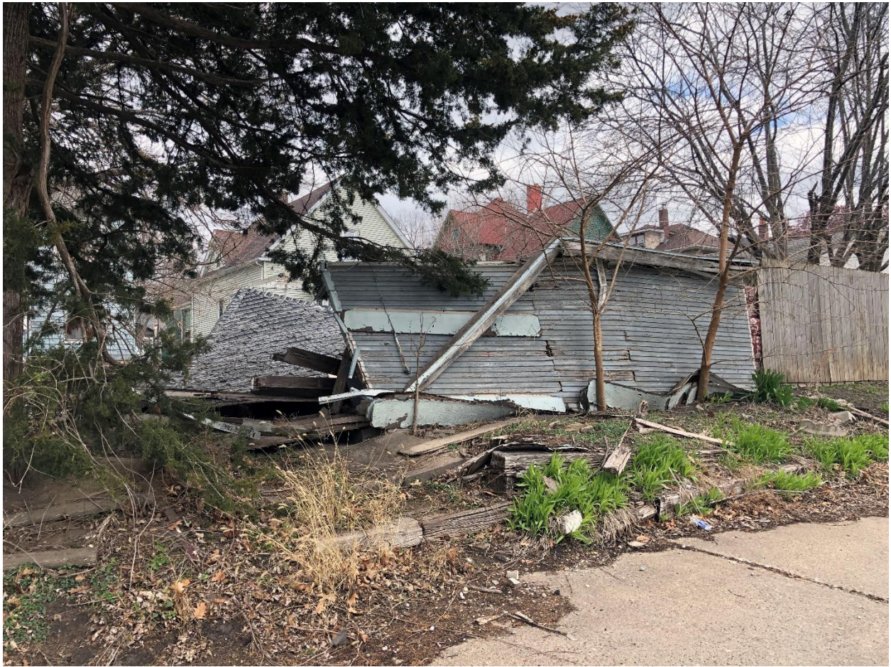
Photograph No. 5: View of the collapsed historic automobile garage looking southeast from the alley.
