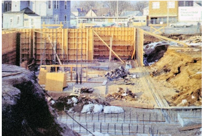
Looking north towards Broadway and Court Streets in 1967, the excavation has been completed, the footings poured and the foundation forms are going up on the new St. Joseph Church.
