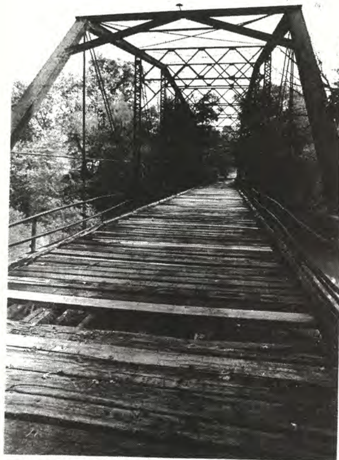
DILAPIDATED BRIDGE over the Big Muddy River at Sand Ridge is no longer in use.
