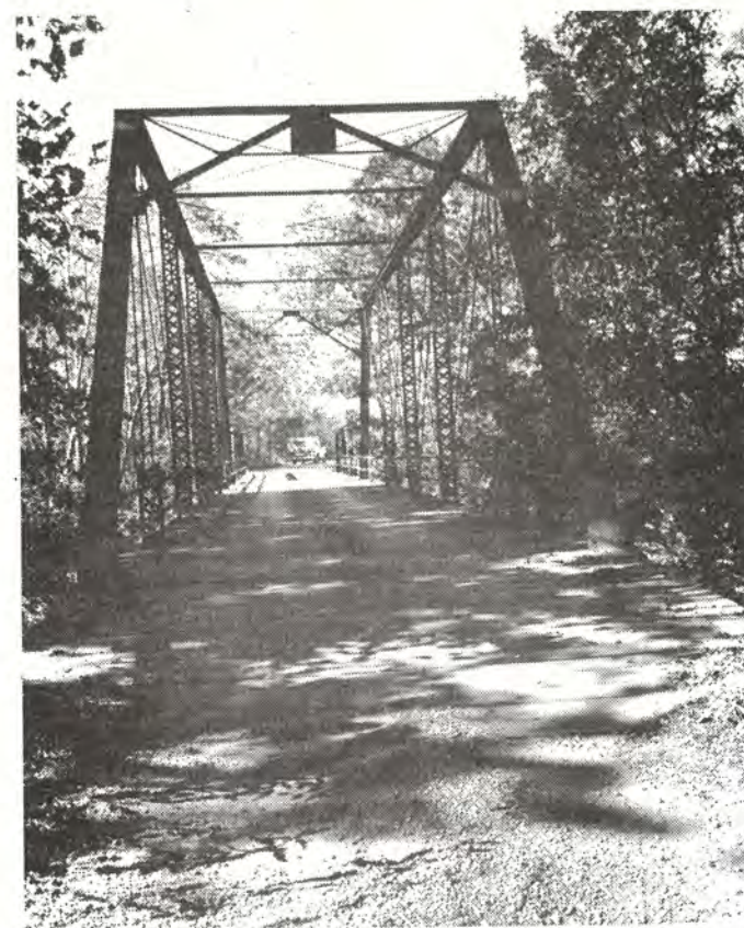
STILL IN USE is this rusty iron bridge over the Beaucoup Creek west of Vergennes.
