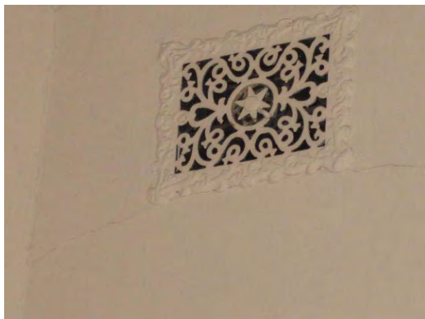
Wall Vent Opening – Star in Center was Connected to Chain Operators to Allow for Opening and Closing Operable Damper Installed Behind Vent Face (Typical)
