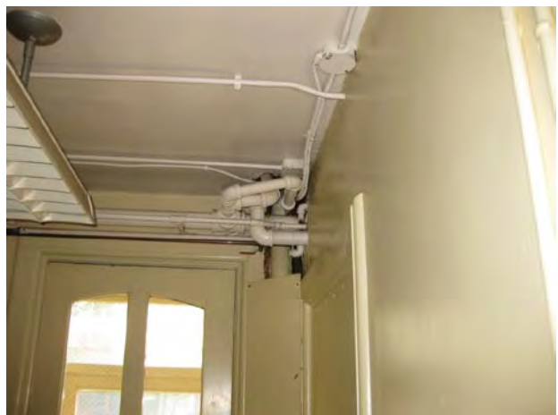
Cast Iron Sanitary Stack at Galvanized Domestic Water up to Third Floor at Back Door Hall
