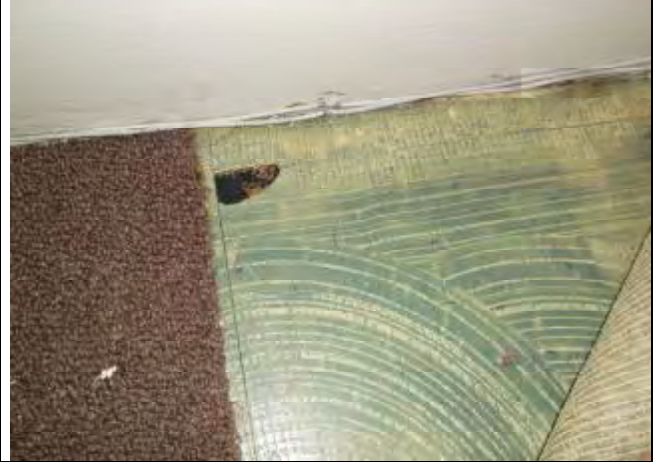
4. View of asbestos containing 9''x 9'' green floor tile located under carpet throughout the east half of the second floor.
