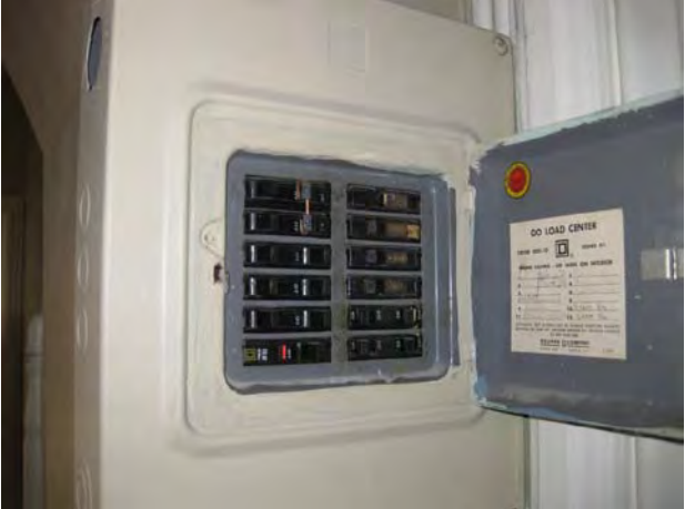
Sub-Panel on Second Floor
