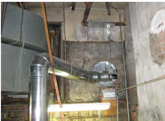
Boiler Flue Forced Draft Fan, Abandoned Ducts From Demolished Grade-Mounted HVAC Unit on Left
