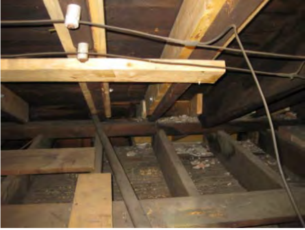
Knob & Tube Wiring in Attic
