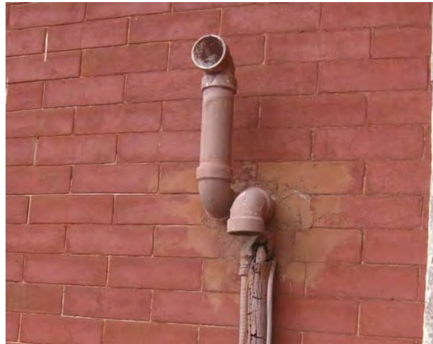
Furnace Flue, Intake and Refrigerant Piping – Painted to Match Adjacent Wall
