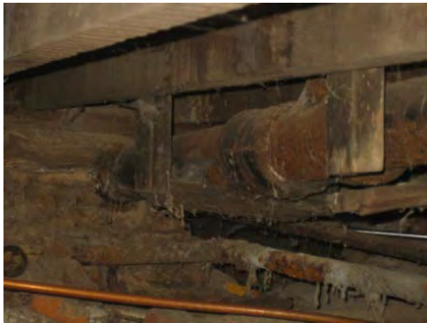
Abandoned Sanitary Piping - Crawlspace
