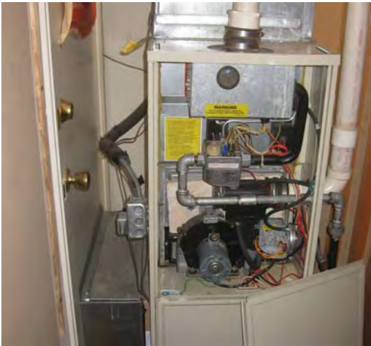
Furnace in Office 303
