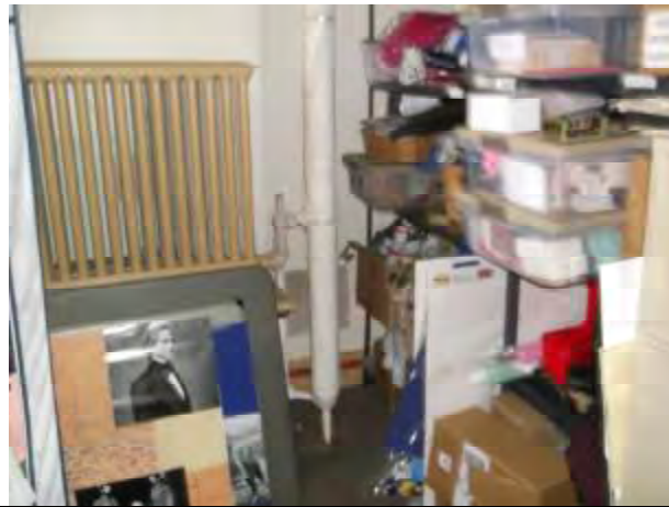
3. View of asbestos containing pipe insulation located on the southwest portion of the ground floor.
