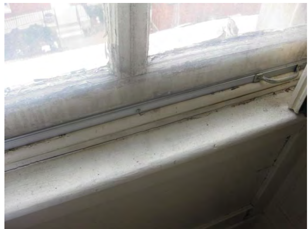
Window Fitted with Plexi-Glass Fixed Interior Storm Pane
