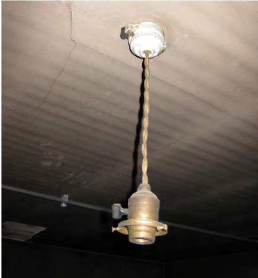
Abandoned Hanging Fixture in Attic
