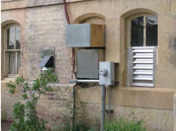
Underground Electric Service at West Side of Building with Surface Conduit Feeding Main Panel and Surface Conduit Up Side of Building to Serve Re-Purposed Fuse Box Floor
