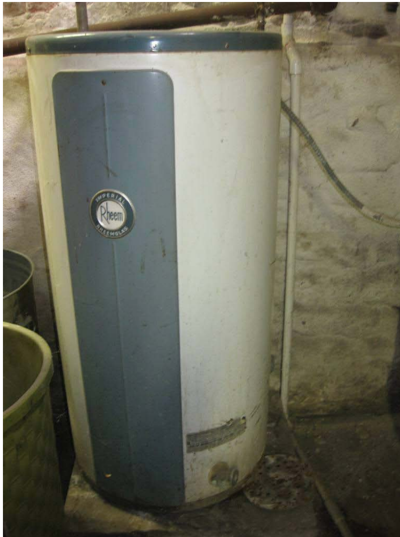
Electric Water Heater in Boiler Room
