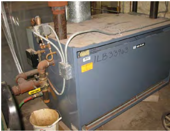
Existing Natural Gas Boiler
