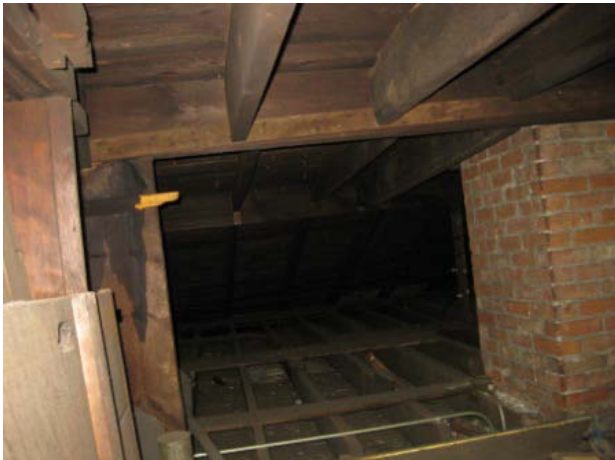
No Insulation in Roof or Floor Joists - Attic
