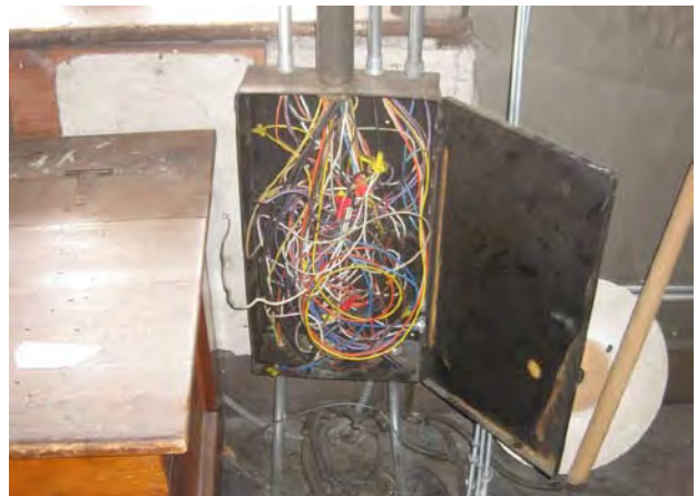
Re-Purposed Fuse Box on Fourth Floor
