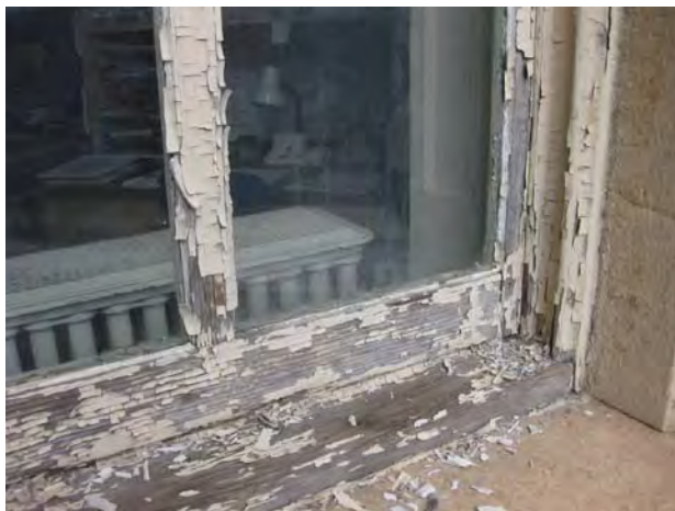
Window in Disrepair Allows Excessive Infiltration
