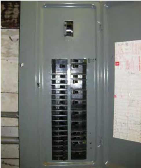
Main Service Panel – 200 Amp, 120-208 Volt, Three Phase
