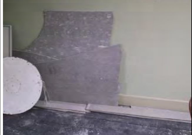
6. View of asbestos containing transite located on the third floor.
