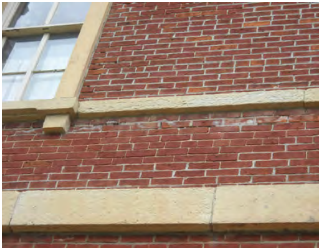
Photo E-4: Efflorescence was noted beneath the limestone stringcourses. This is likely because water enters the wall above the stringcourse and seeps down. It is not particularly of concern.
