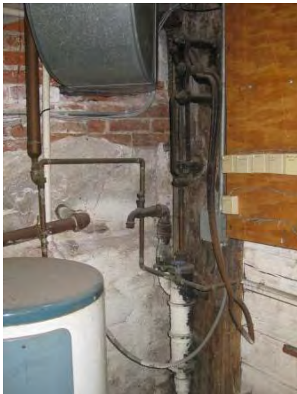
Abandoned Hand Pump on Wall – Boiler Room
