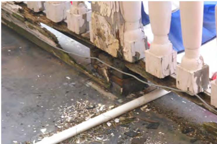
Photo E-35: The bottom member of the porch railing at the Bedroom Level/3 rd Fl. has completely rotted due to excessive moisture from a condensate tube.
