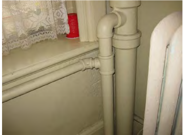
Sanitary and Vent Stack at Third Floor
