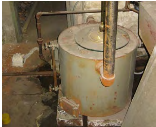
Existing Condensate Receiver
