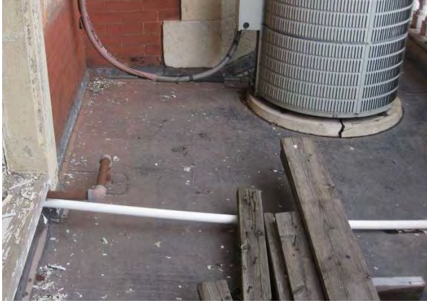
Gas Pipe & Condensate Drain for Furnace in Adjacent Office 303
