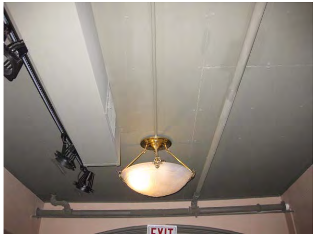
Duct in First Floor Main Hall
