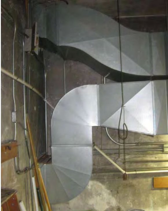
Duct in Boiler Room penetrating Main Hall Wall
