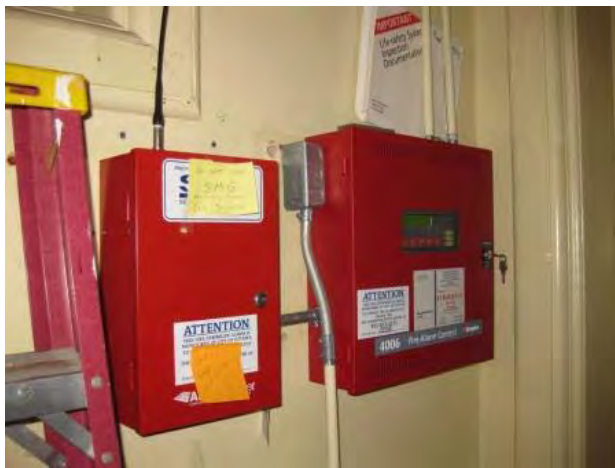
Fire Alarm Panel
