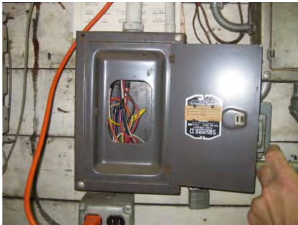
Main Service Panel – 200 Amp, 120-208 Volt, Three Phase
