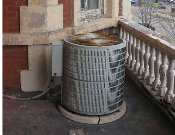
Condensing Unit for Furnace in Office 303
