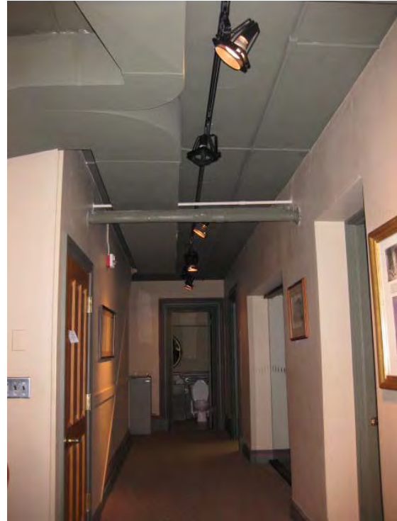
Duct in First Floor Main Hall
