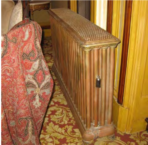
Wrought Tube Radiator – Second Floor
