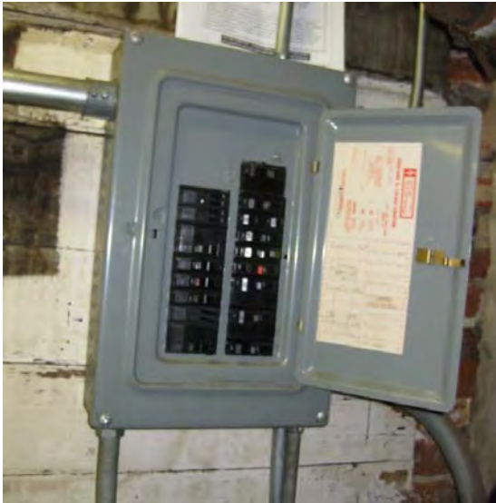
Second Service Panel – 100 Amp, 120-208 Volt, Single-Phase
