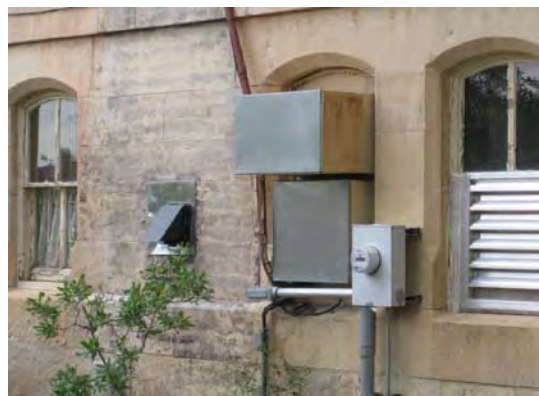
Boiler Forced Flue Vent Cap on Left, Combustion Air Louver on Right, Abandoned HVAC Ducts Penetrating Window Opening in Center
