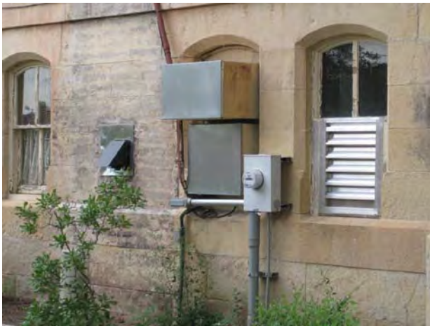
Duct from Demolished Air Conditioner at Boiler Room
