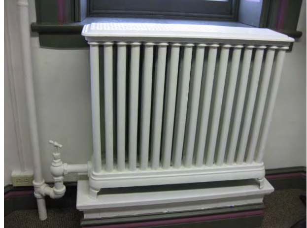
Wrought Tube Radiator – First Floor
