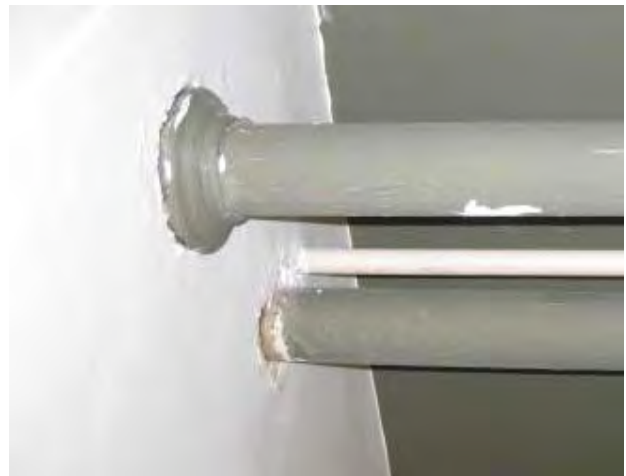
Escutcheon Plate on Pipe at Wall in Normal Location
