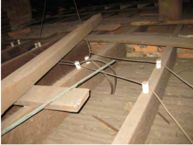
Knob & Tube Wiring in Attic
