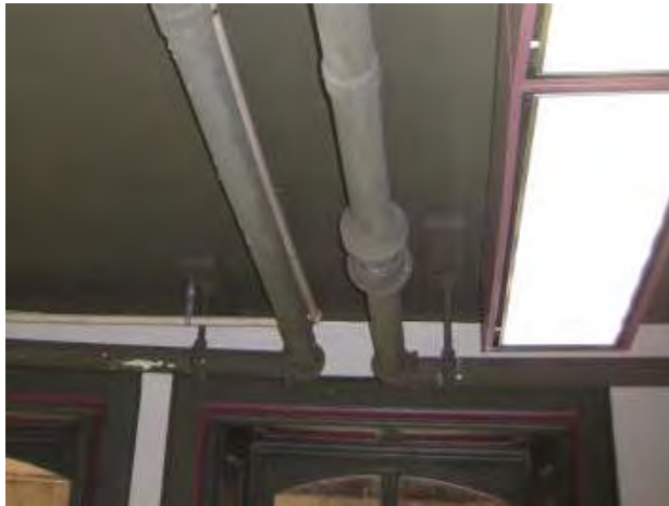
Zone Piping Looking East on 1 st floor – Zone Pipe on Right turns for South Zone and Zone Pipe on Left turns for North Zone. Escutcheon Plates on Pipe Illustrate Possible Location of Demolished Wall on 1 st floor
