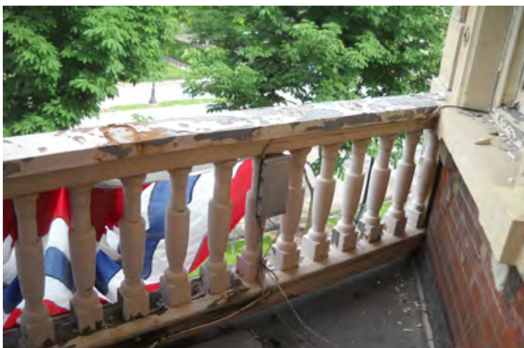
Photo E-36: View looking down on the railing, showing the galvanized sheet metal cap that was placed over the top of the rail. This helps protect the wood rail, but it has not been painted and is starting to rust.
