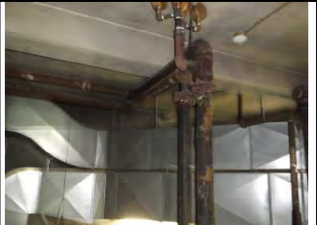
2. View of asbestos containing pipe insulation and fittings located in the boiler room.
