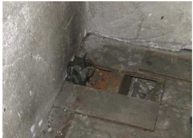
Lead Fill and Distribution Pipes in Former Water Tank Room – 4 th Floor
