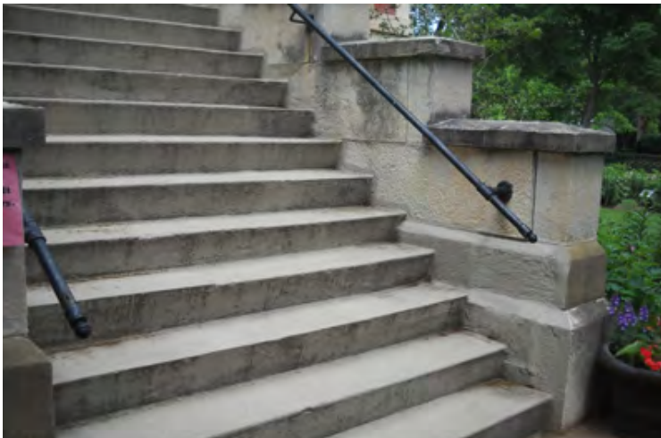
Photo E-19: The front entry steps are limestone, although they are covered with a durable rubberized coating system. This system may keep the water out, but it also traps the moisture in.
