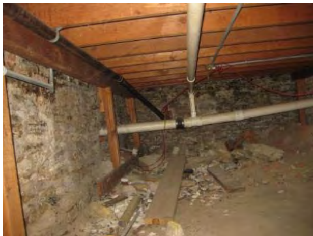
PVC Sanitary Routed to West Through Crawlspace and Black Steel Gas Main Entering at North Wall of Crawlspace, Routed South to Boiler Room
