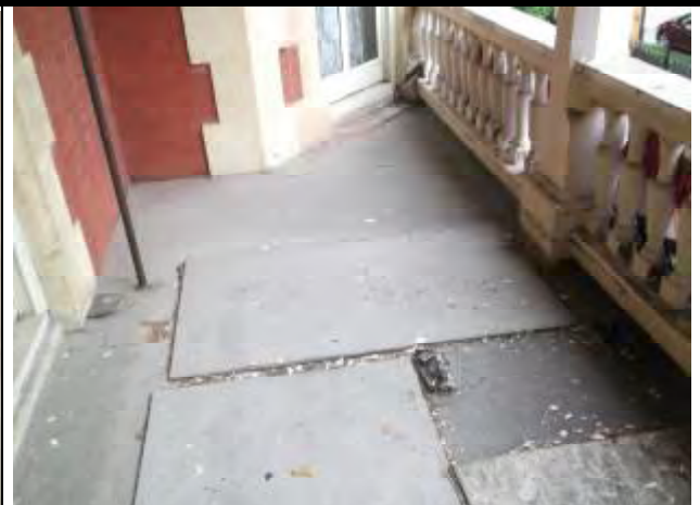
8. View of Presumed Asbestos Containing Materials (PACM), roof field and flashing materials located on the landings and roof areas.
