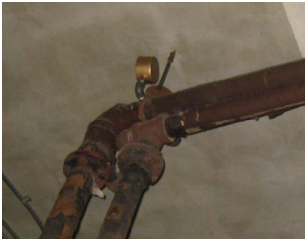
High Point Automatic Air Vent in Boiler Room
