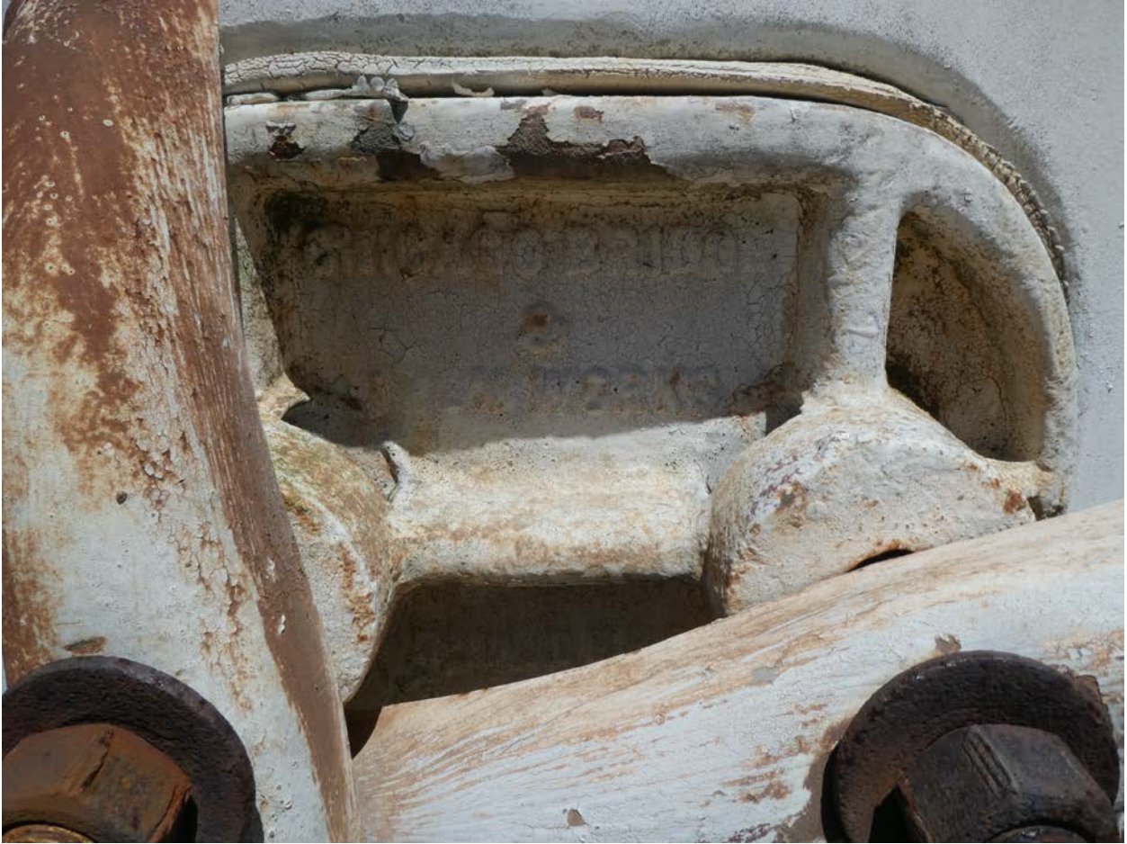
Photo 14 - Detail view of base hatch with embossed lettering - CHICAGO BRIDGE AND IRON WORKS (BUILDERS), facing northeast.
