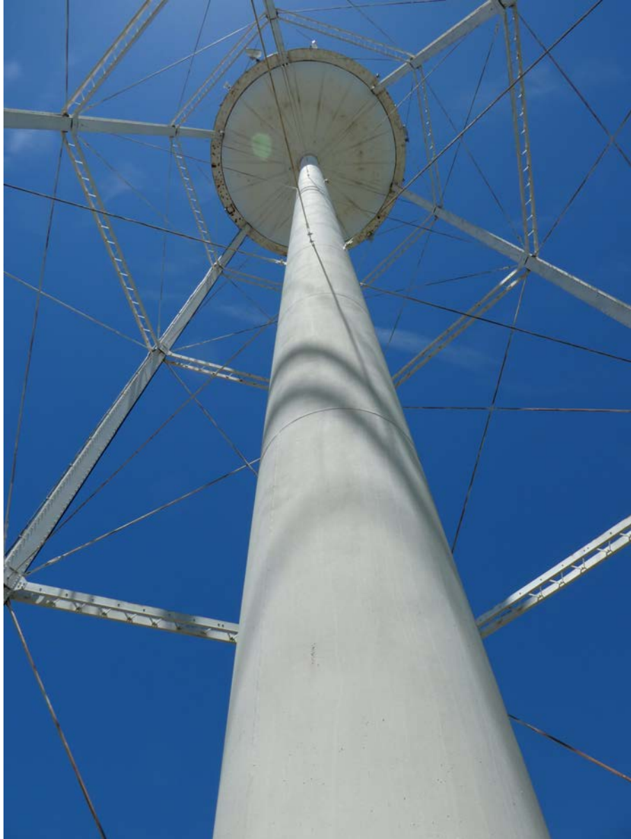
Figure 12. Detail view of uptake pipe to storage tank, facing north.
