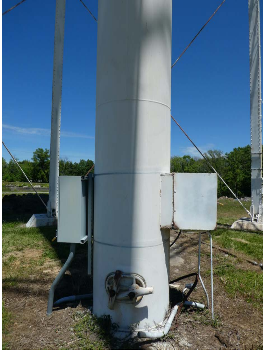
Photo 13 - Detail view of base of uptake pipe with base hatch, facing northeast.
