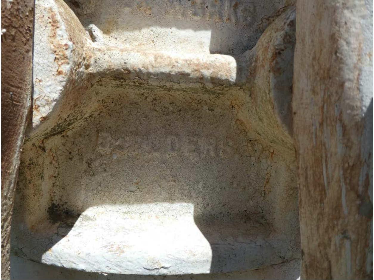
Photo 15 - Detail view of base hatch with embossed lettering – (CHICAGO BRIDGE AND IRON WORKS) BUILDERS, facing northeast.
