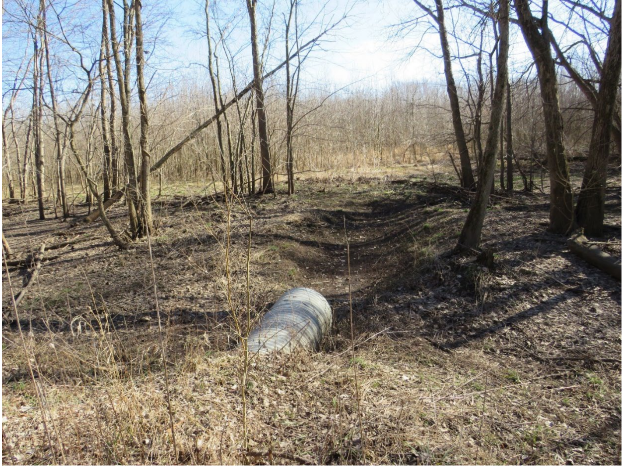
Figure 4-15. BH-RR-03. Bruce Hannon Levee Trail. Culvert. Photograph taken from Tour Stop 5. View to the East. Tetra Tech, 2024.
