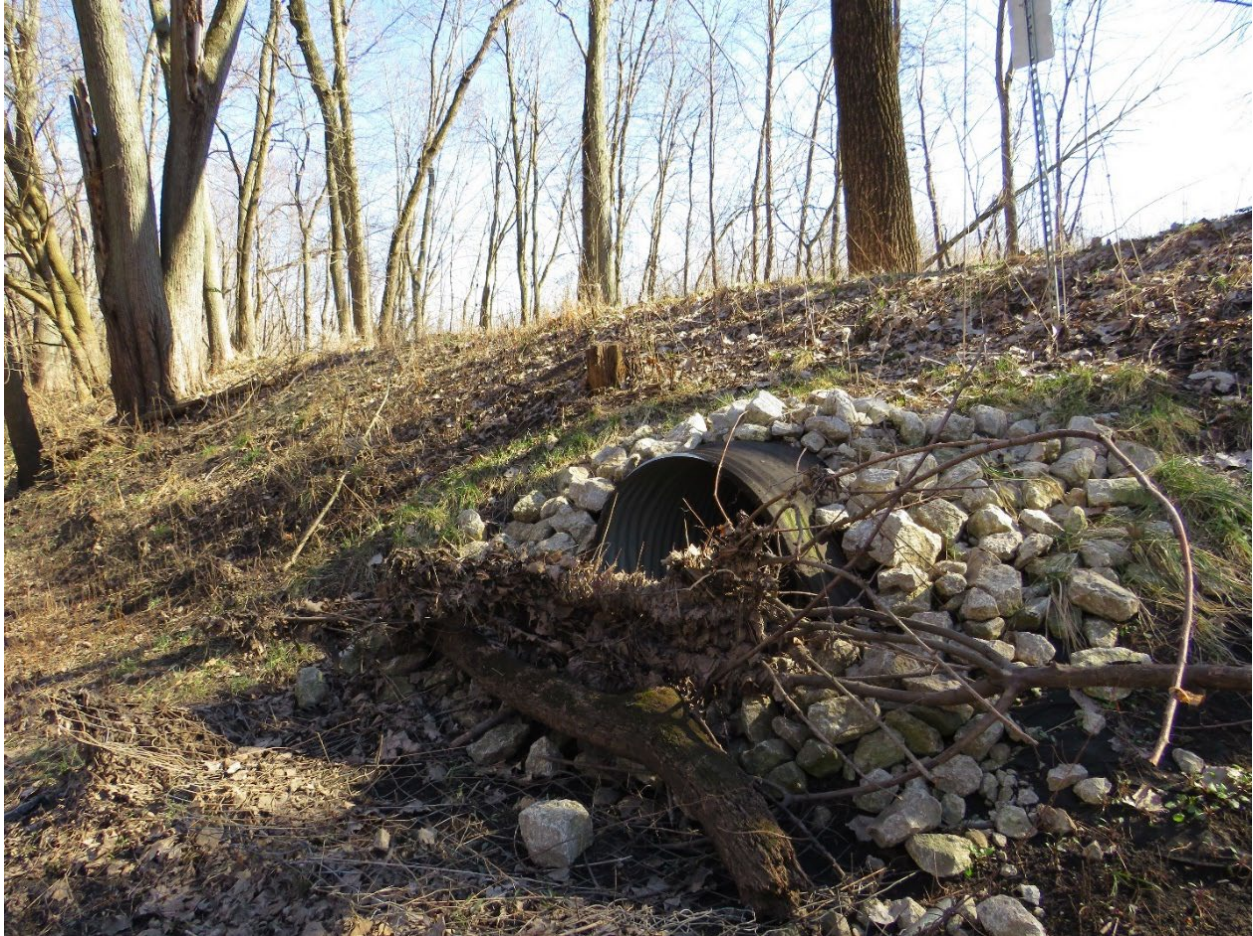
Figure 4-14. BH-RR-03. Bruce Hannon Levee Trail. Culvert. Photograph taken from Tour Stop 5. View to the Southeast. Tetra Tech, 2024.
