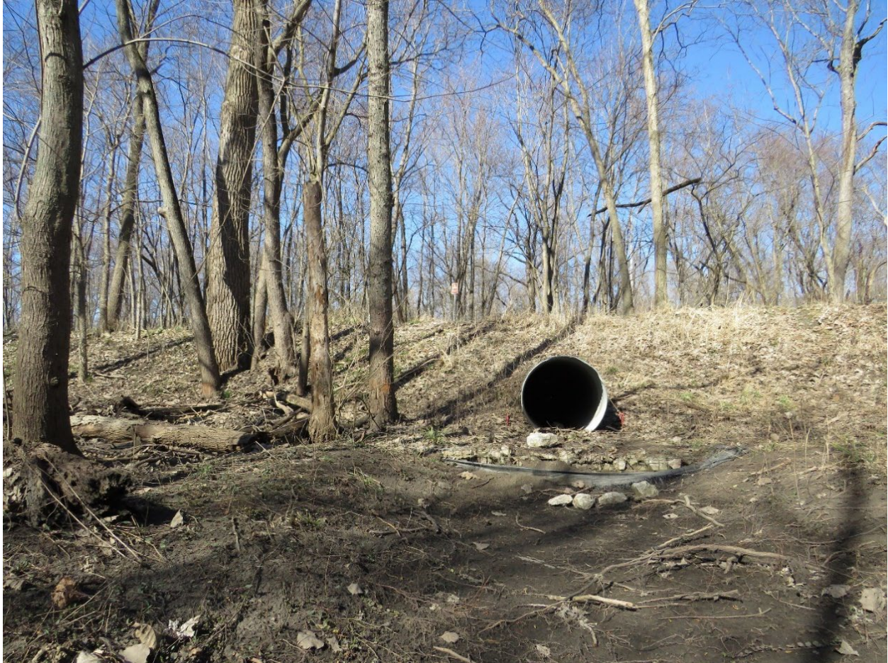
Figure 4-8. BH-RR-01. Bruce Hannon Levee Trail. Culvert. Photograph taken near Tour Stop 4. View to the North-Northeast. Tetra Tech, 2024.
