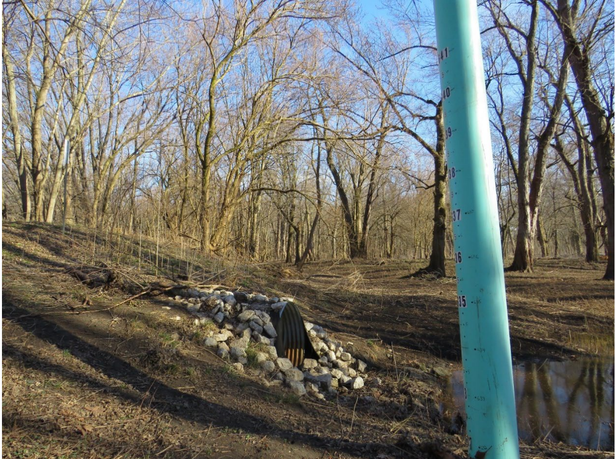
Figure 4-19. Bruce Hannon Levee Trail. Culvert and Water Level Gauge. Photograph taken from Tour Stop 10. View to the East-Southeast. Tetra Tech, 2024.
