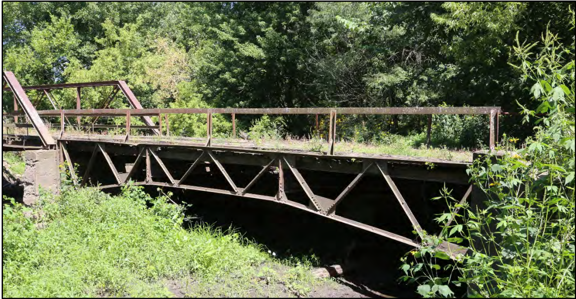
Figure 4: This image of the subject bridge illustrates well a Cantilevered Bedstead Truss of the Indiana Bridge Company, a plan sheet for which is found in Figure 3, Page 9.
