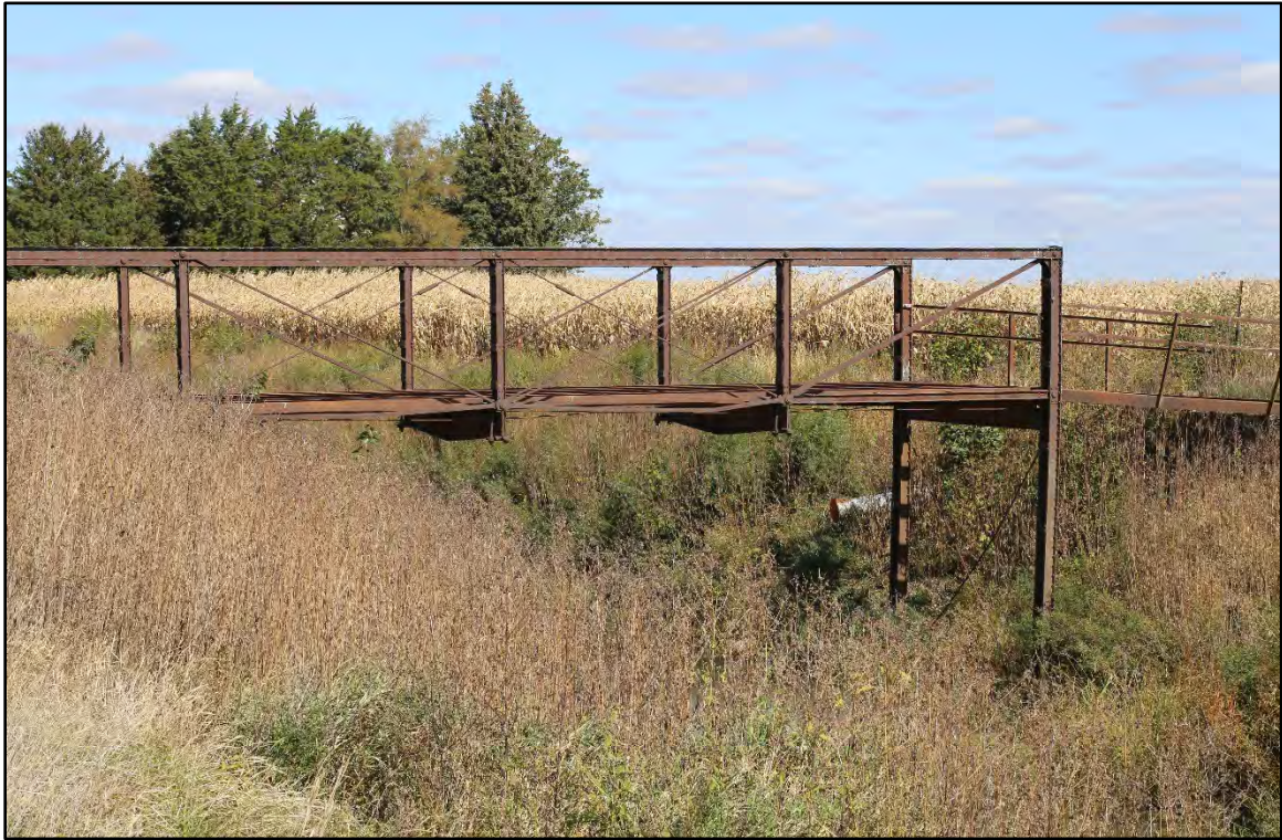
Figure 2: This image illustrates a Bedstead Truss bridge in its most simple form, that is a span carried by nothing more than four end posts that extend down to a mud sill several feet below ground. Note that there are no restraints behind the legs to hold fill for the approaches since this structure used approach spans to either side of the legs. This is an abandoned bridge in Iroquois County, Illinois.
