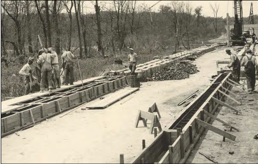
Figure 14: “Pouring concrete piling[s]” describes the activity shown (adapted from the original Bridge Photoset in possession of IDOT and ISAS).
