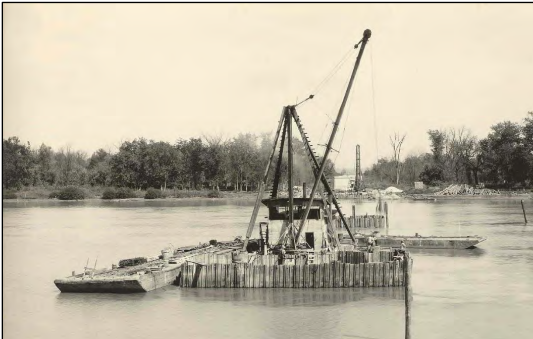
Figure 13: Identified with a caption acknowledging “construction view showing coffer dams for piers 3, 4 and 6” (adapted from the original Bridge Photoset in possession of IDOT and ISAS).
