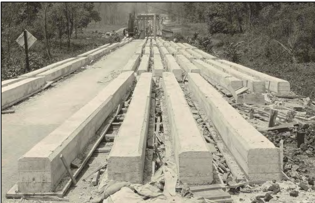
Figure 15: This photograph had no apparent caption. It shows the concrete piles used for the east approach spans which are the product of the activity shown in Figure 14 above (adapted from the original Bridge Photoset in possession of IDOT and ISAS).
