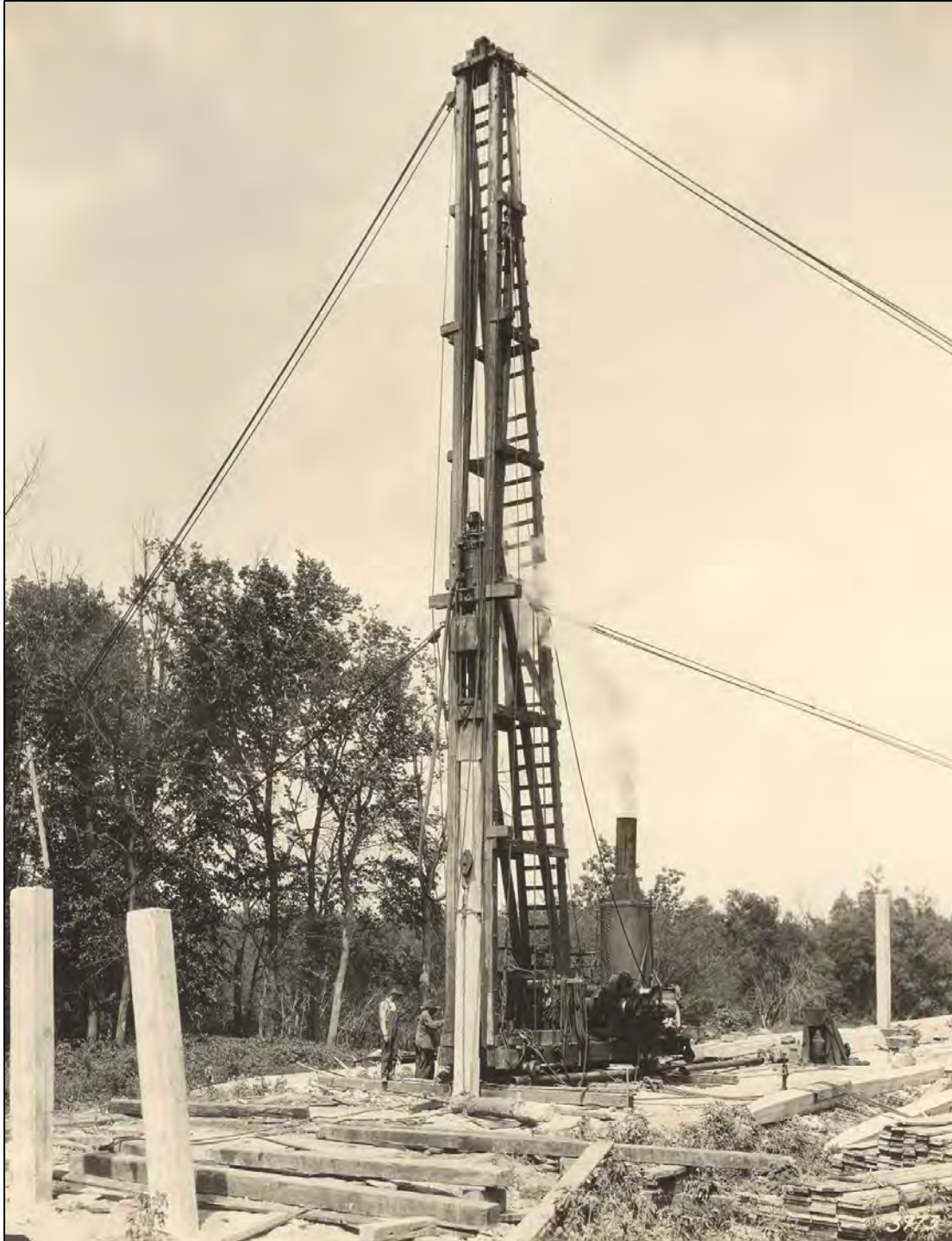
Figure 16: Although a caption was not found for this image, it shows the concrete piles for the easternmost, post-and-beam approach spans (see Figures 14 and 15 for images of how the piles were produced) being driven into the ground (adapted from the original Bridge Photoset in possession of IDOT and ISAS).
