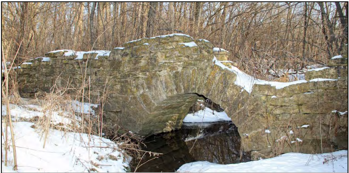
Figure 1: This image pictures in January 2016 the remains of the ca. 1830s stone arch bridge situated on the nineteenth-century Chicago-Galena Road.
