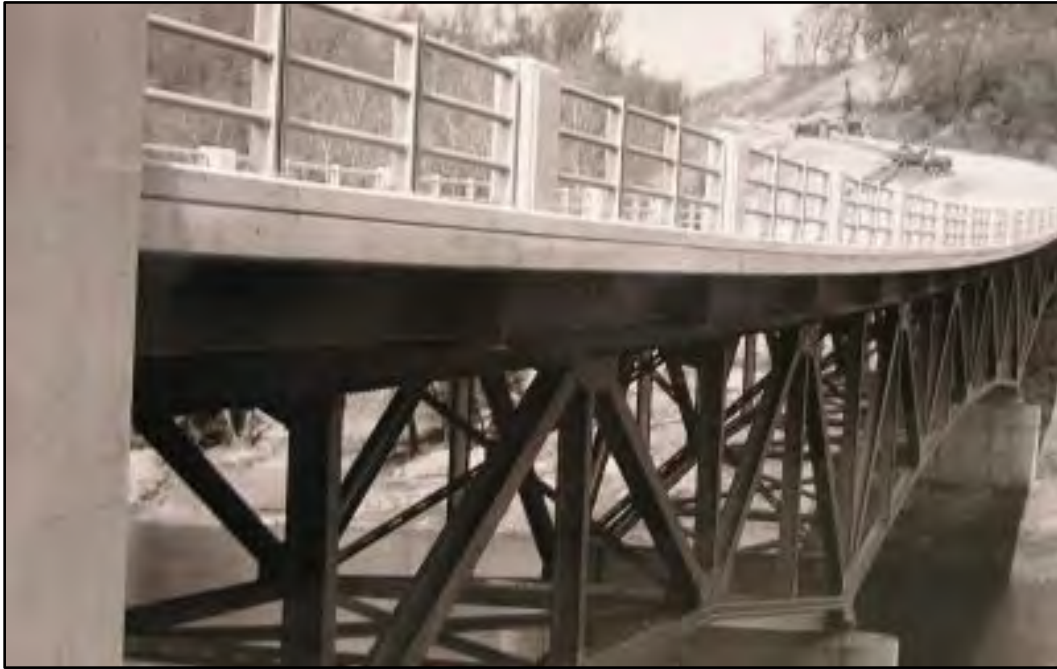
Figure 9: View to North picturing both the bridge's original railing, as well as the truss work below. Viewed at http://bridgehunter.com/il/la-salle/5030381146/ on 05 December 2015.
