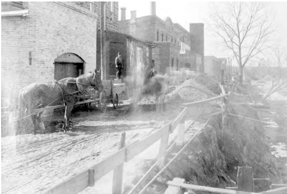
Figure 2. View from south bank of North Head Race, looking west and showing excavation work at the North Head Race, ca.1904. Square tower in background is part of the former Pitt's Manufacturing Company building.
