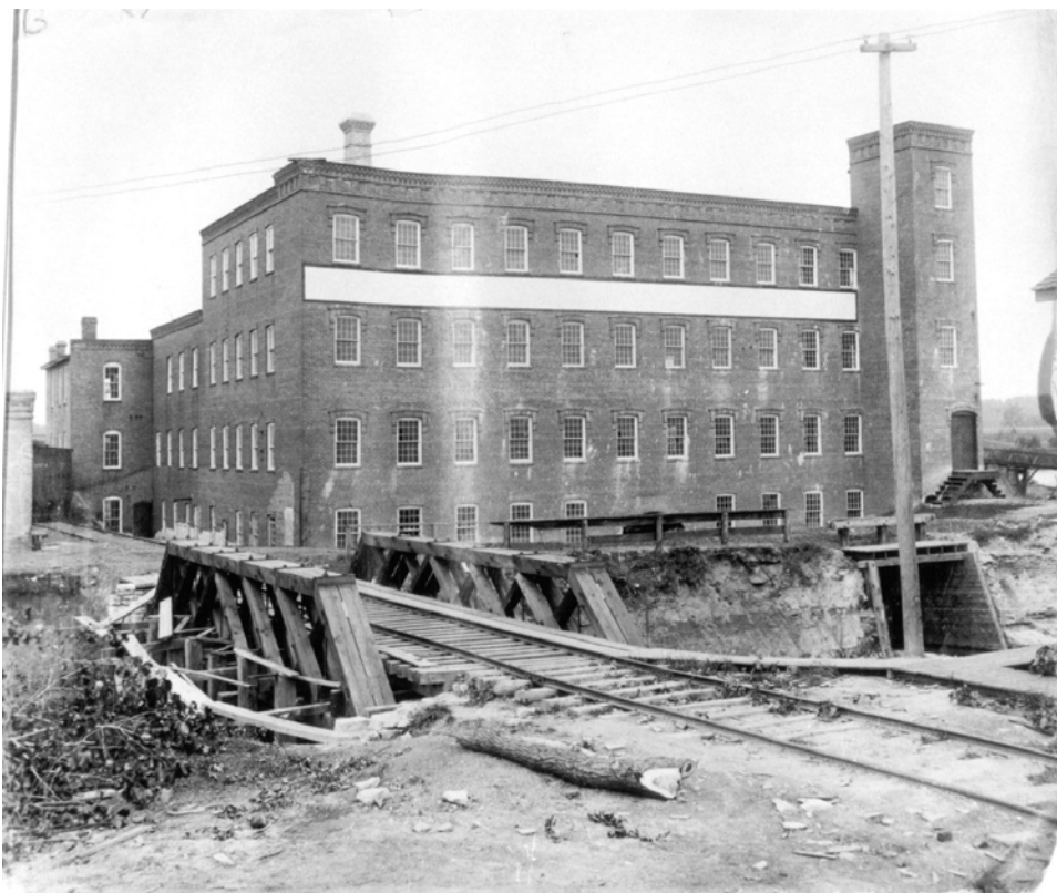
Figure 4. View looking south toward the former Pitt's Manufacturing Company, and showing progress of construction work at the North Head Race, ca. 1904 From the archives of: Marseilles Land & Water Company
