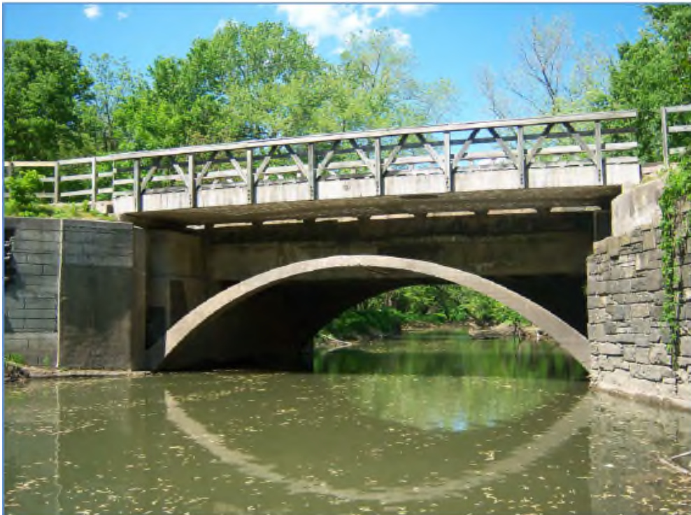
Modern-day views of the Nettle Creek Aqueduct, showing conditions prior to the 2013 flood event. (TOP) View of the north elevation in 2012. (BOTTOM) View of the south elevation in 2009.
