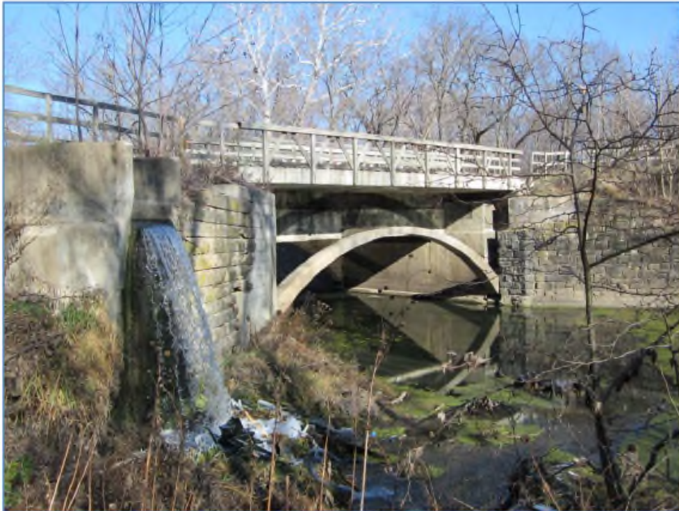
Additional modern-day views of the aqueduct, showing pre-2013 conditions. (TOP) View looking east along the pedestrian walkway and trunk. (BOTTOM) View of the south elevation, looking northeast. The spillway can be seen at left.
