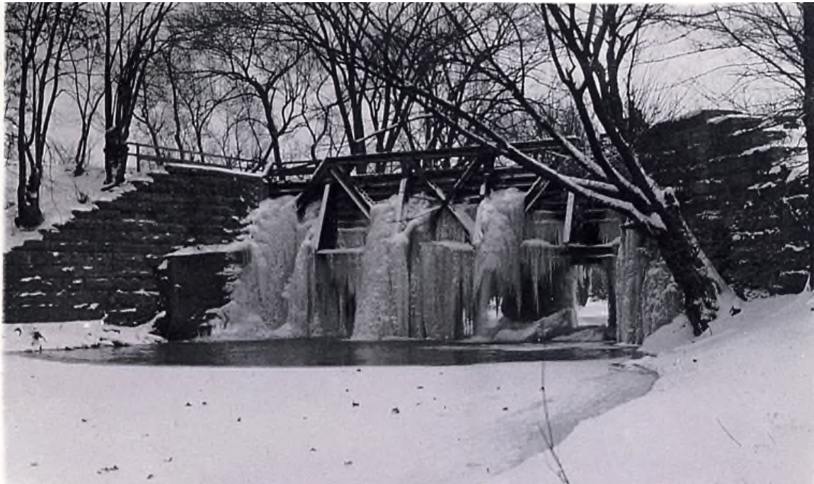
Two views of the Nettle Creek Aqueduct showing the steel-frame structure that was installed in 1910. These photographs are undated but possibly were taken in the 1920s or early 1930s (based on the drastic leaks in the aqueduct's trunk). Both views show the north side of the aqueduct and look southeast. Note the addition of poured concrete along the lower part of the east abutment.
