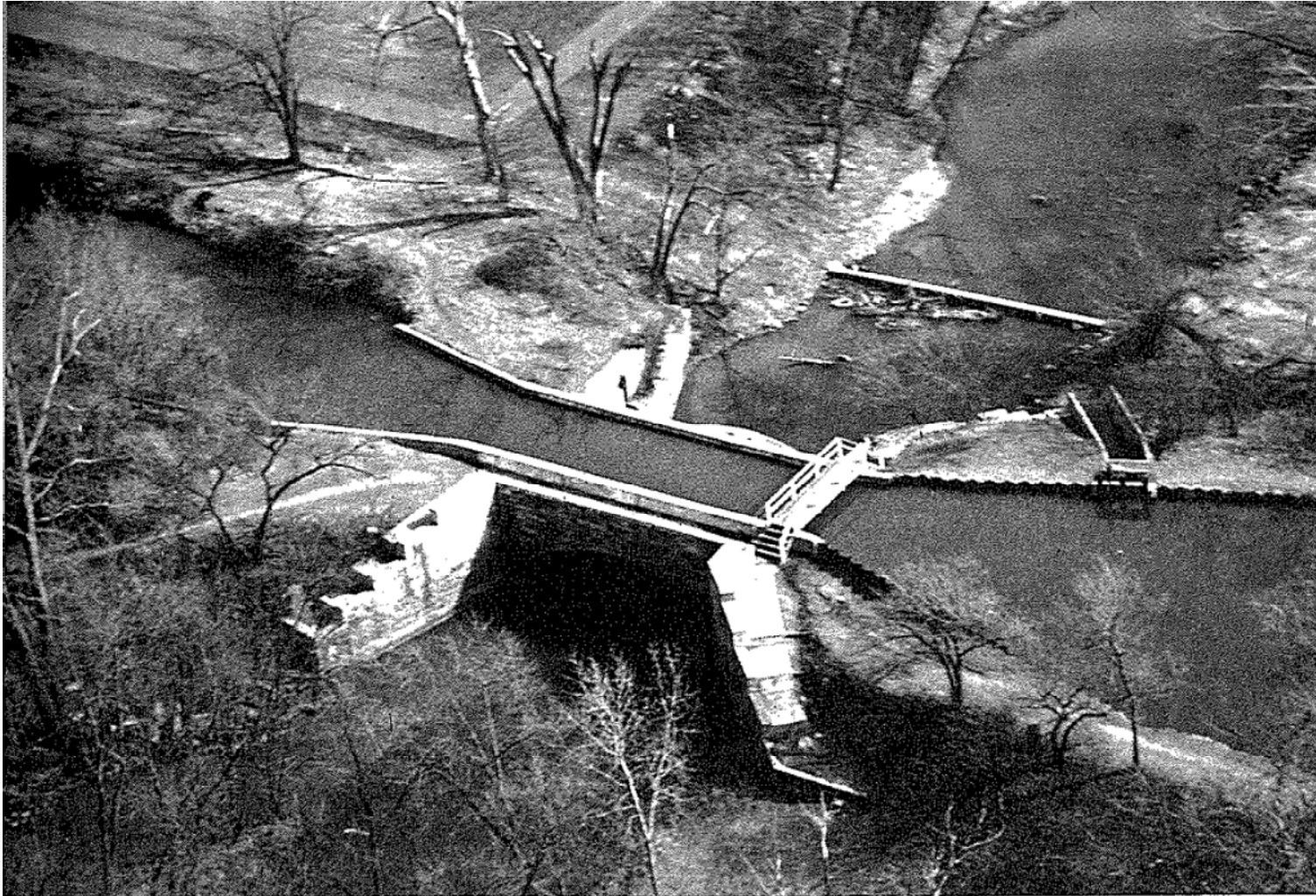
Photograph of the Nettle Creek Aqueduct, taken circa 1974. By this date, the bridge deck on the south side of the aqueduct apparently had been removed.
