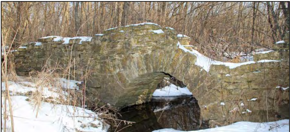
Figure 1: This image pictures in January 2016 the remains of the ca. 1830s stone arch bridge situated on the nineteenth-century Chicago-Galena Road.
