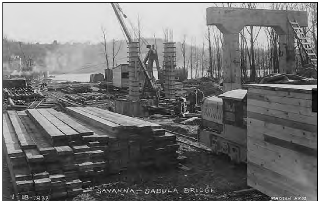
Image viewed at https://www.flickr.com/photos/45436499@N02/6828577832/ on 08 May 2015. Work on the foundation of the Savanna-Sabula Bridge, 18 January 1932. View to East Southeast.
