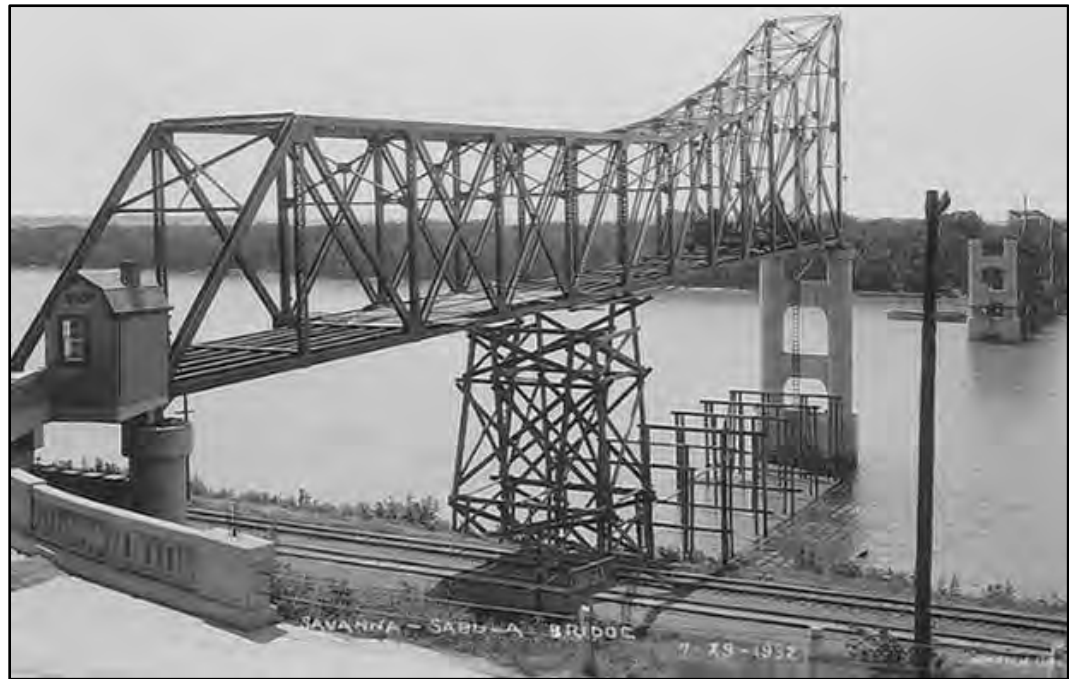
Image viewed at https://www.flickr.com/photos/45436499@N02/6974704091/ on 08 May 2015. Construction of the Savanna-Sabula Bridge on 29 July 1932. View to West Southwest.
