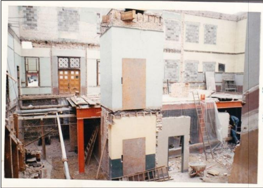
Photograph, 1967, showing interior remodel of the Carnegie library building, elevator shaft. Source: Rockford Public Library, Local History & Genealogy Department.
