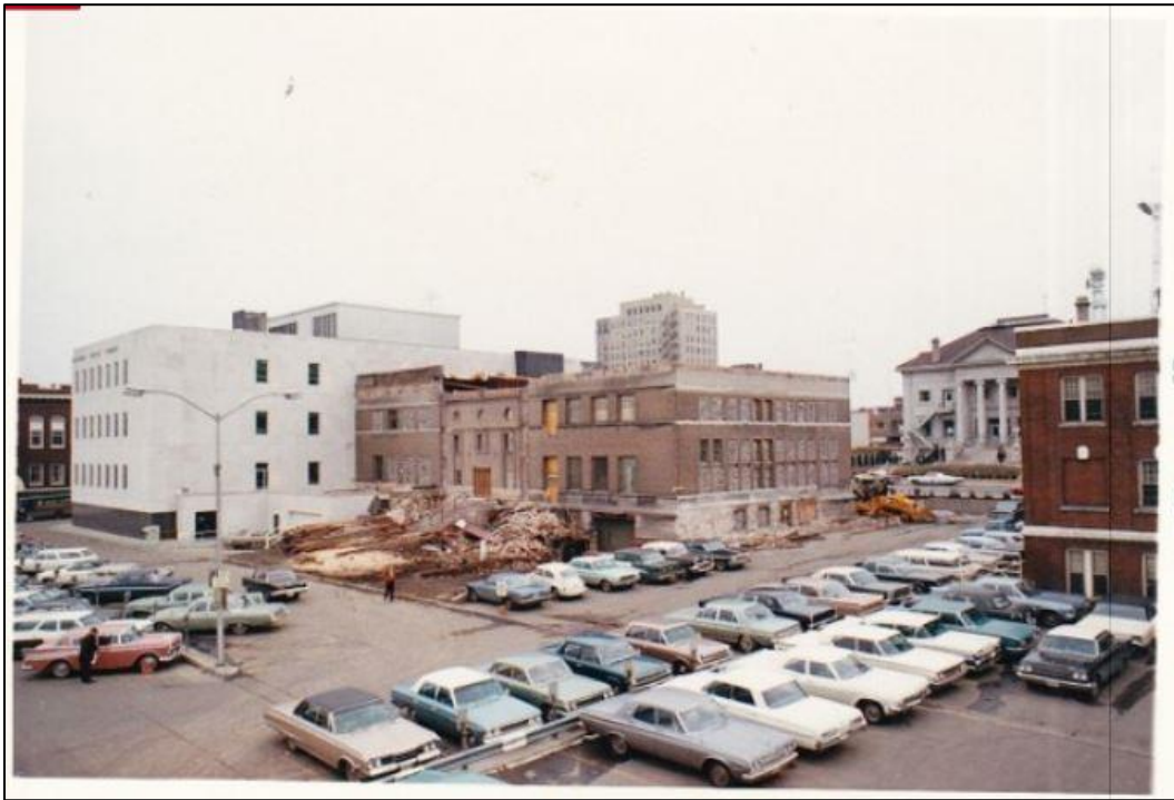
Photograph, 1967, showing remodel of the Carnegie library building. Source: Rockford Public Library, Local History & Genealogy Department.
