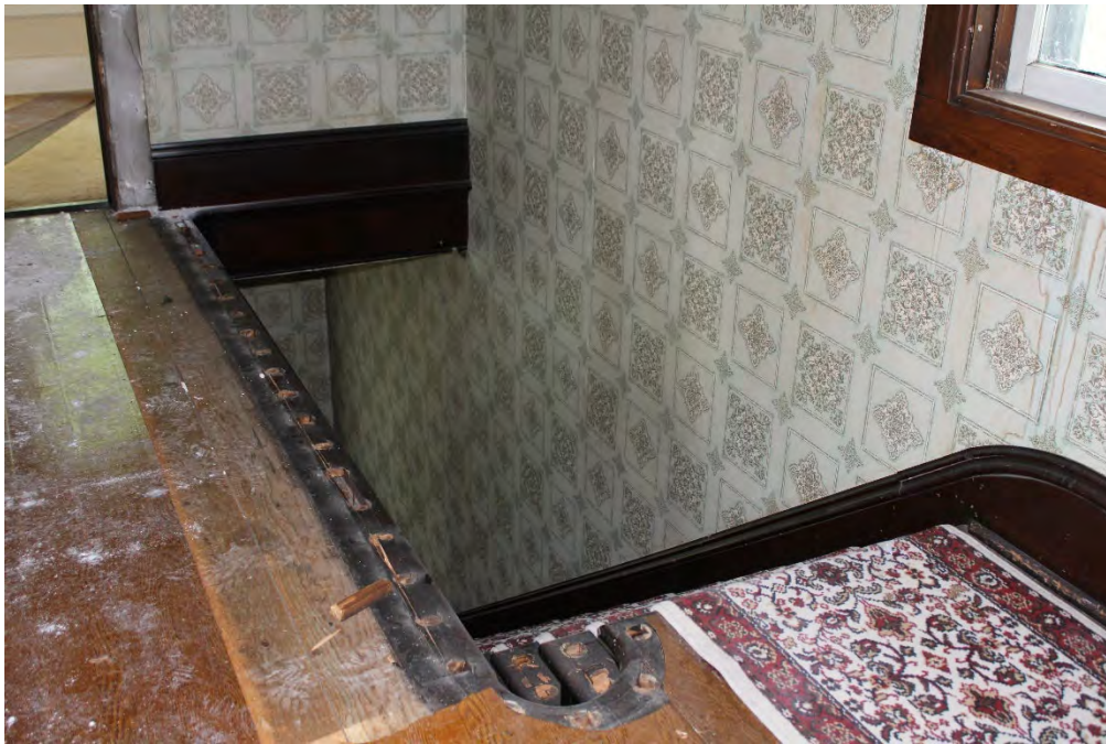
Figure 26. Interior, second floor main stair hall; Habitat for Humanity removed banister and railing, any posts, other trim
