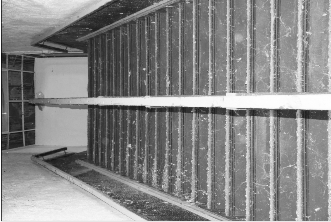
Photo #25 of 29 (turn 90° to the right for viewing)
