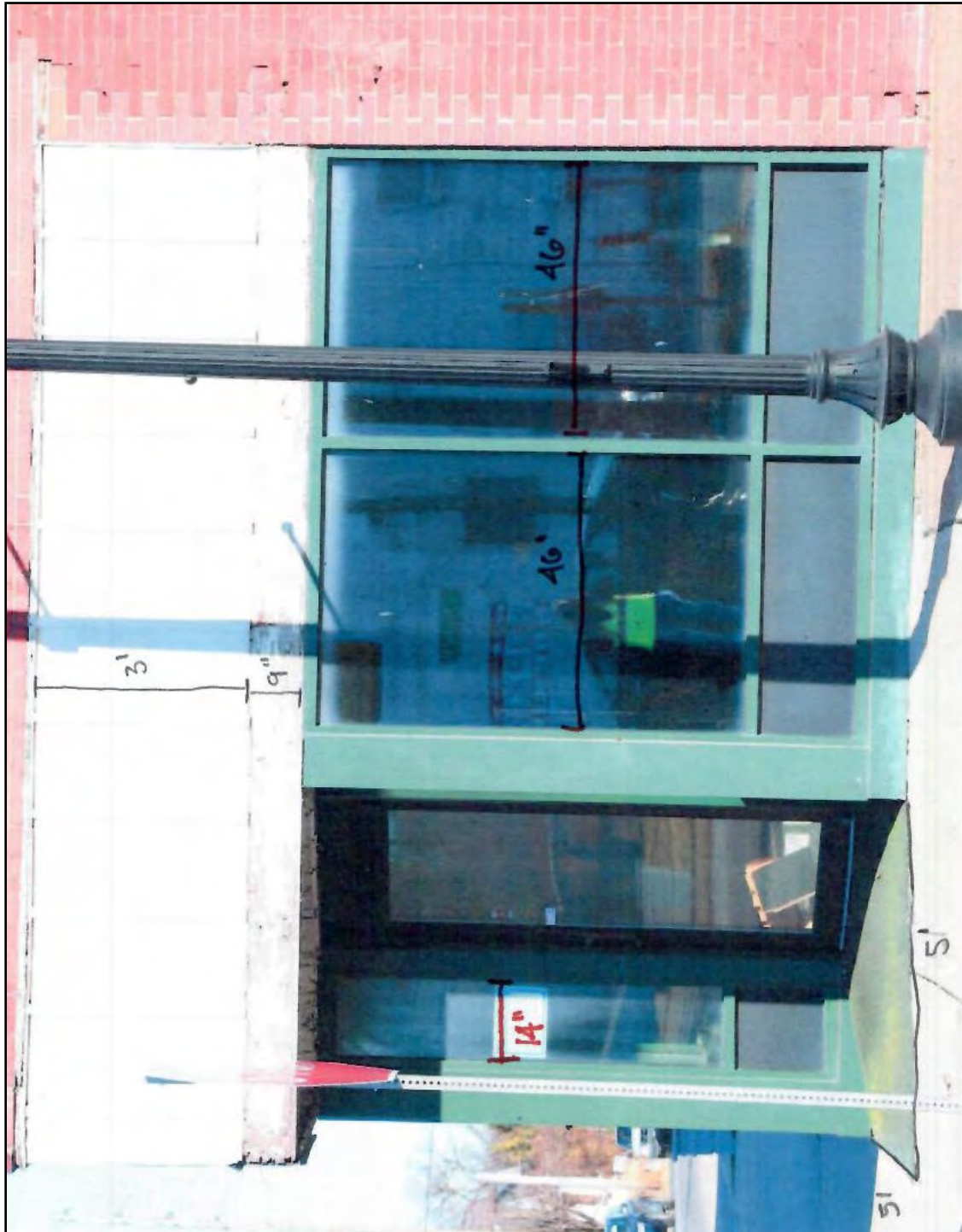
Figure 13: West side of 2 East Water Street. Storefront section at north end of wall.
