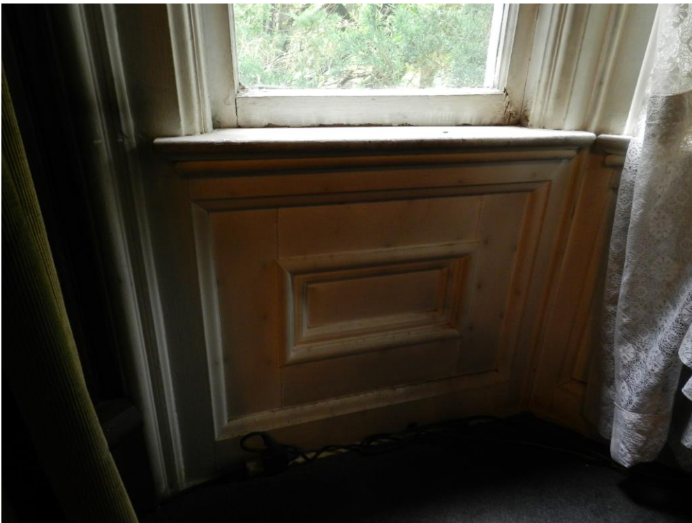
Plate 12. Original panel modeling in the Dining Room, below the bay window openings. Photograph from the Phase I investigations (89).
