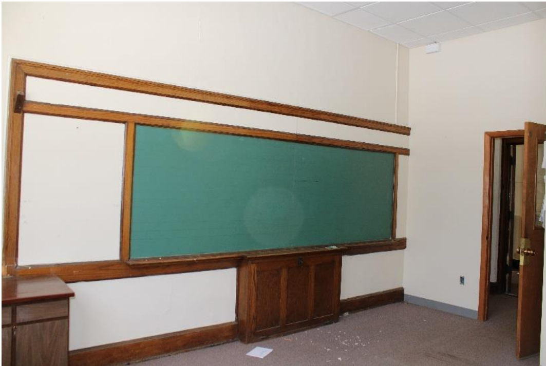
Figure 15: Classroom near the southeast corner of the school with original wood-trimmed chalkboard and cabinet.
