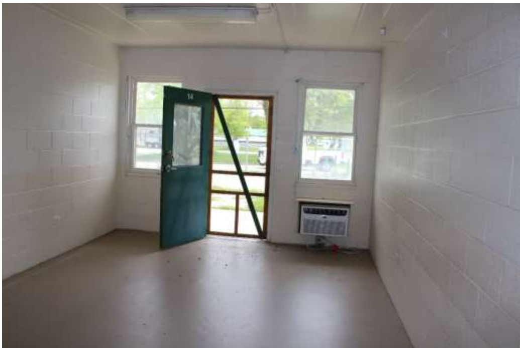
Photograph 72: Entrance to a room in one of the dormitories with concrete block walls built post-2000.
