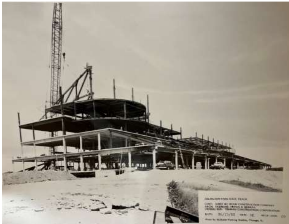
Figure 49: Arlington Park grandstand under construction, June 15, 1988, view northwest. McShane-Fleming Studios, photographer. Source: Arlington Heights Historical Museum.
