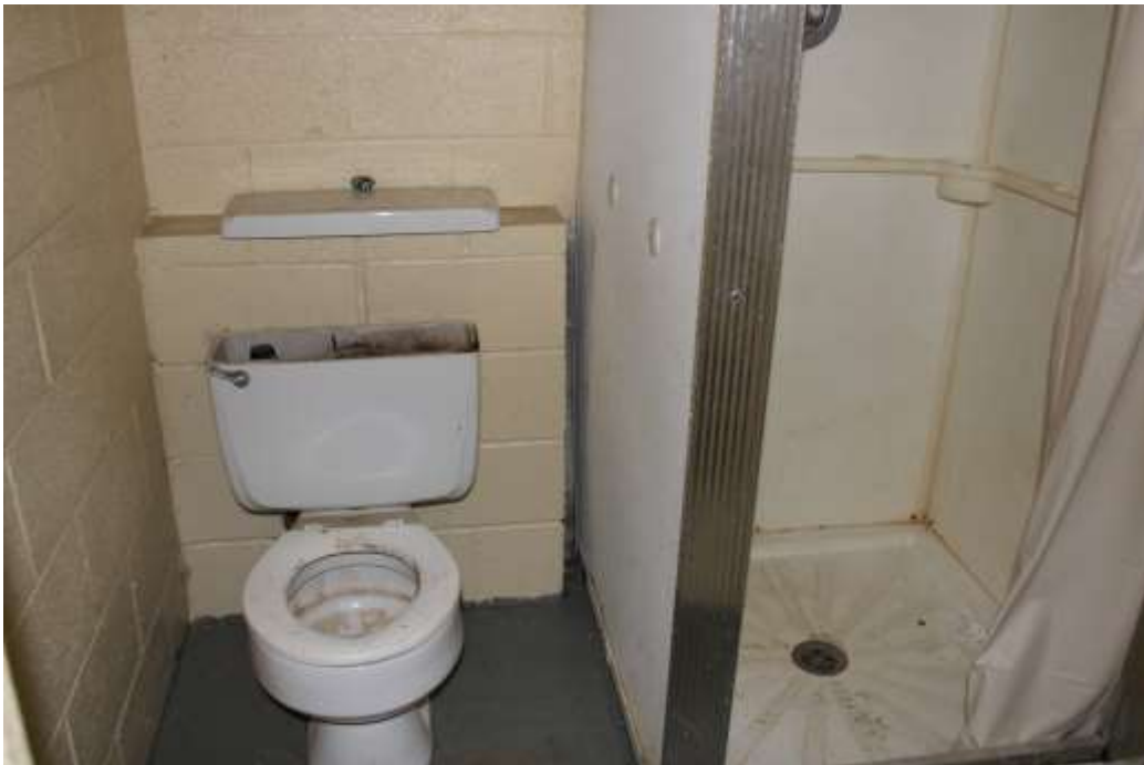
Photograph 68: Private bathroom in one of the concrete block dormitories that were built c. 1985 (sink not shown).
