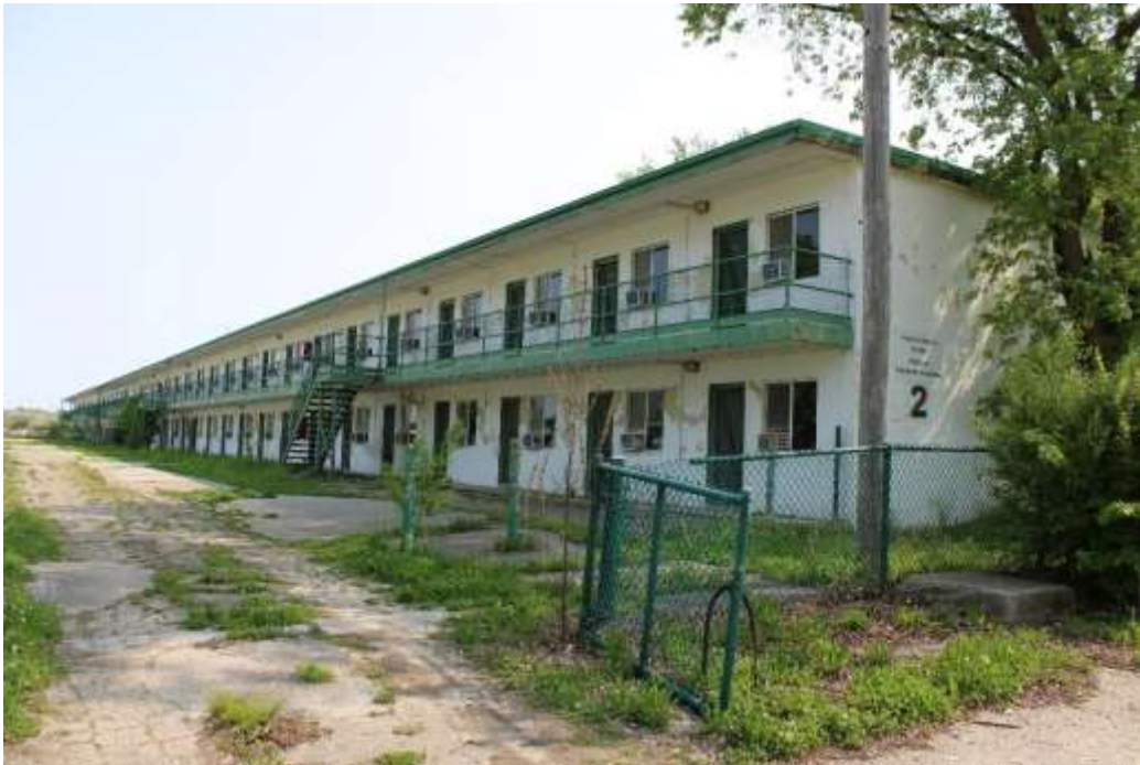
Photograph 63: One of three concrete block, motel-style dormitories with communal bathrooms that were built c. 1973.
