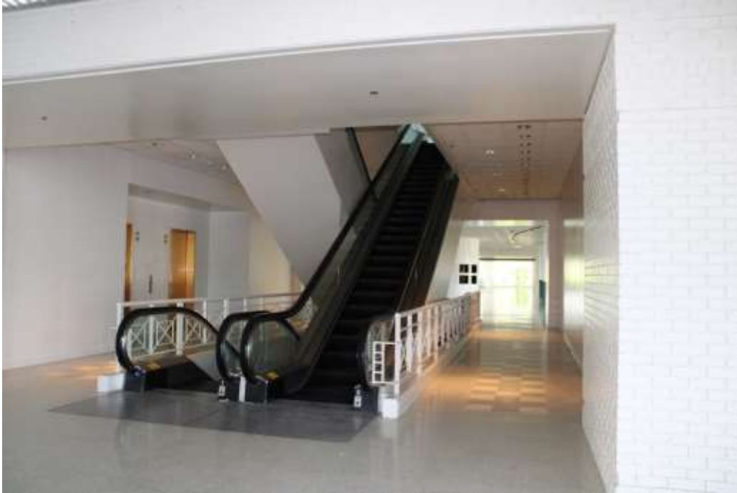
Photograph 19: Typical pair of escalators in the grandstand.
