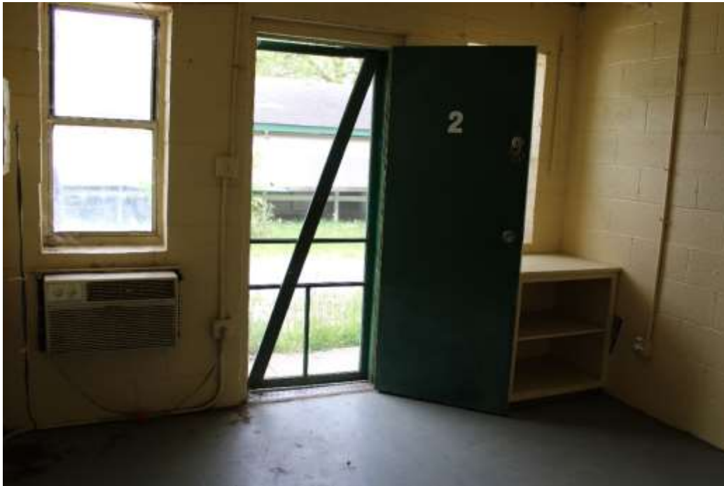
Photograph 69: Entrance to room in one of the concrete block dormitories built c. 1985.
