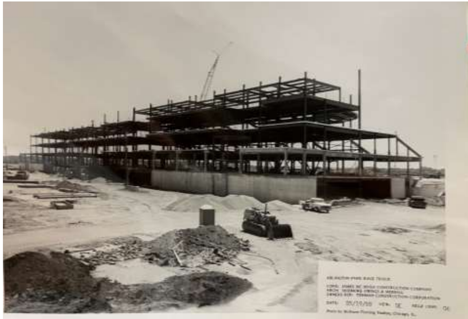
Figure 48: Arlington Park grandstand under construction, May 19, 1988, view southeast. McShane-Fleming Studios, photographer. Source: Arlington Heights Historical Museum.
