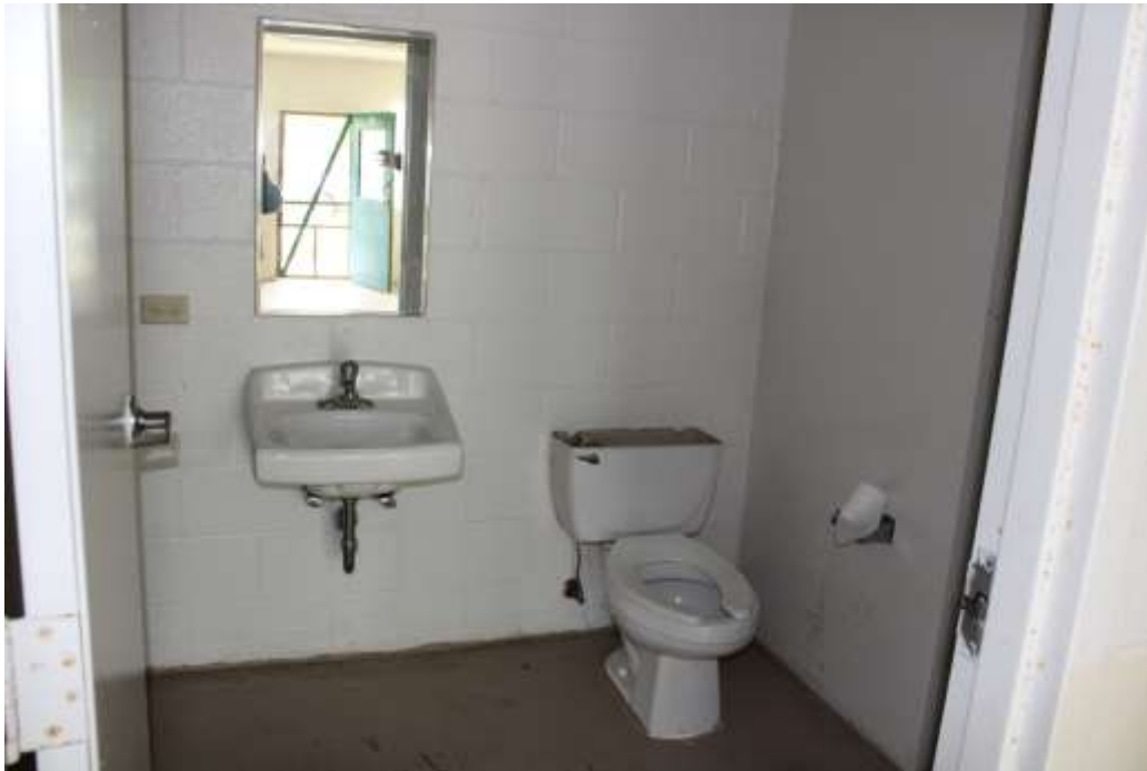
Photograph 73: Private bathroom in one of the dormitories with concrete block walls built post-2000.
