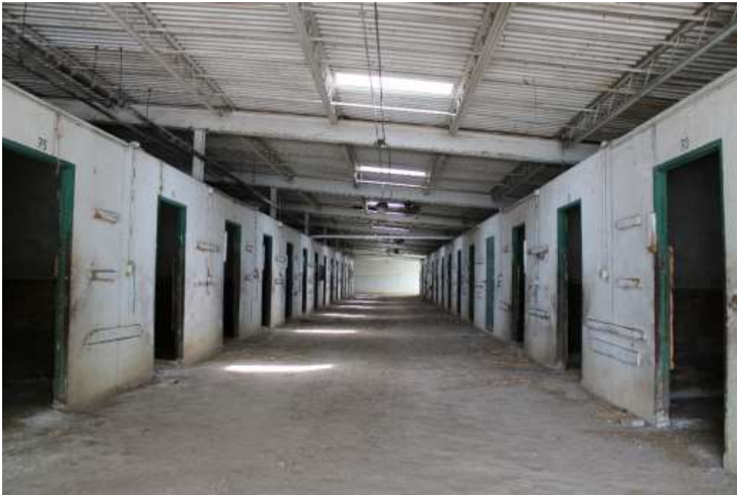
Photograph 57: Typical stable with precast concrete wall panels showing one of the double-loaded aisles opening onto stalls.
