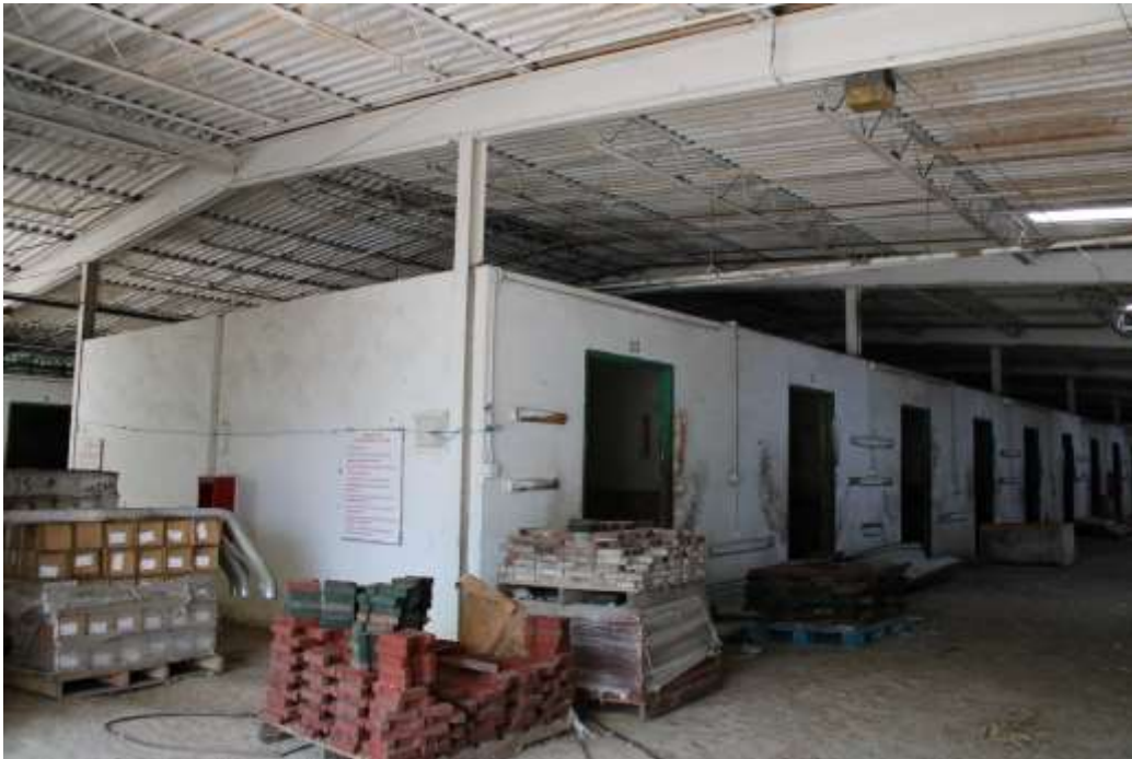
Photograph 55: Center row of stalls in typical stable with precast concrete wall panels.
