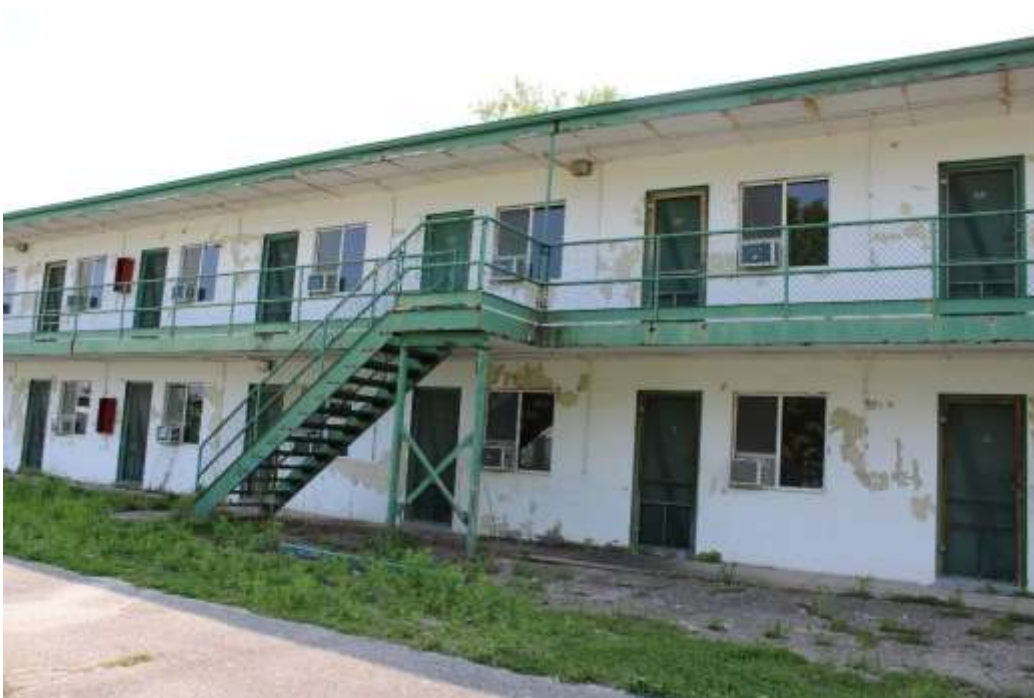
Photograph 64: Detail of a concrete block, motel-style dormitory with communal bathrooms that were built c. 1973.
