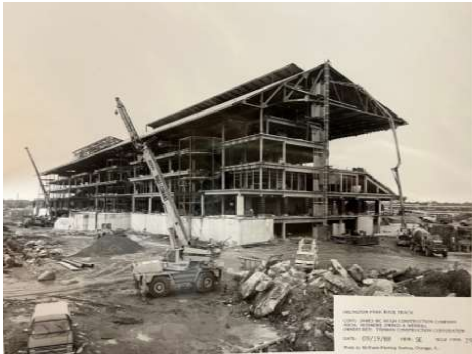
Figure 50: Arlington Park grandstand under construction, September 19, 1988, view southeast. McShane-Fleming Studios, photographer. Source: Arlington Heights Historical Museum.
