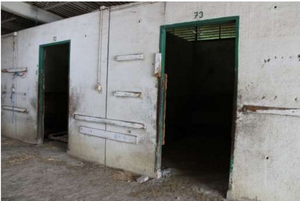
Photograph 58: Openings to stalls within a typical stable with precast concrete wall panels.
