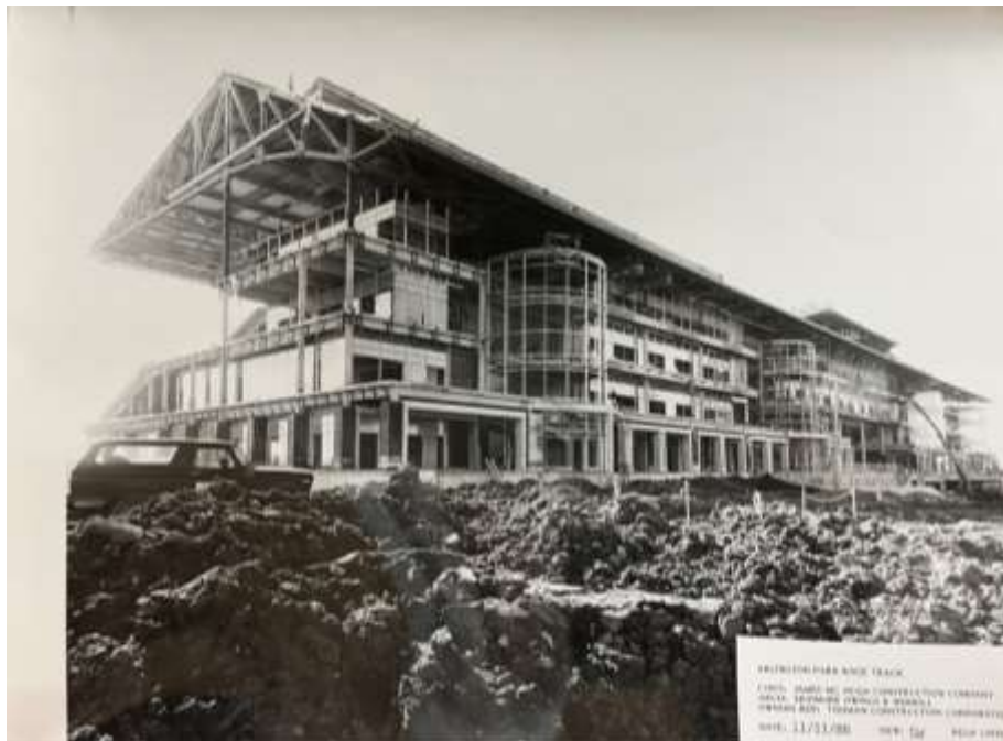
Figure 53: Arlington Park grandstand under construction, November 11, 1988, view southwest. McShane-Fleming Studios, photographer. Source: Arlington Heights Historical Museum.
