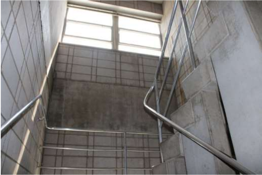
Photograph 19: Concrete staircase linking the balcony levels at the east end of the laboratory.
