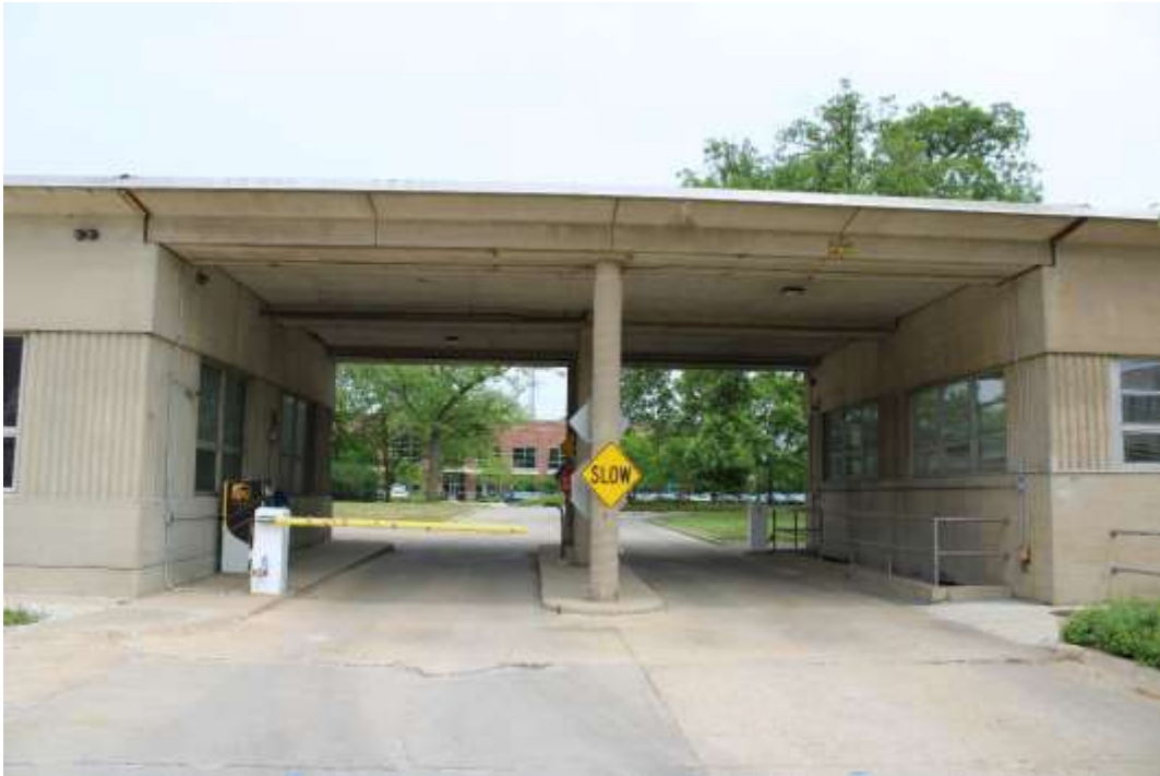
Photograph 17: Canopy linking the Research Building (right) with the Material Storage Building (left).
