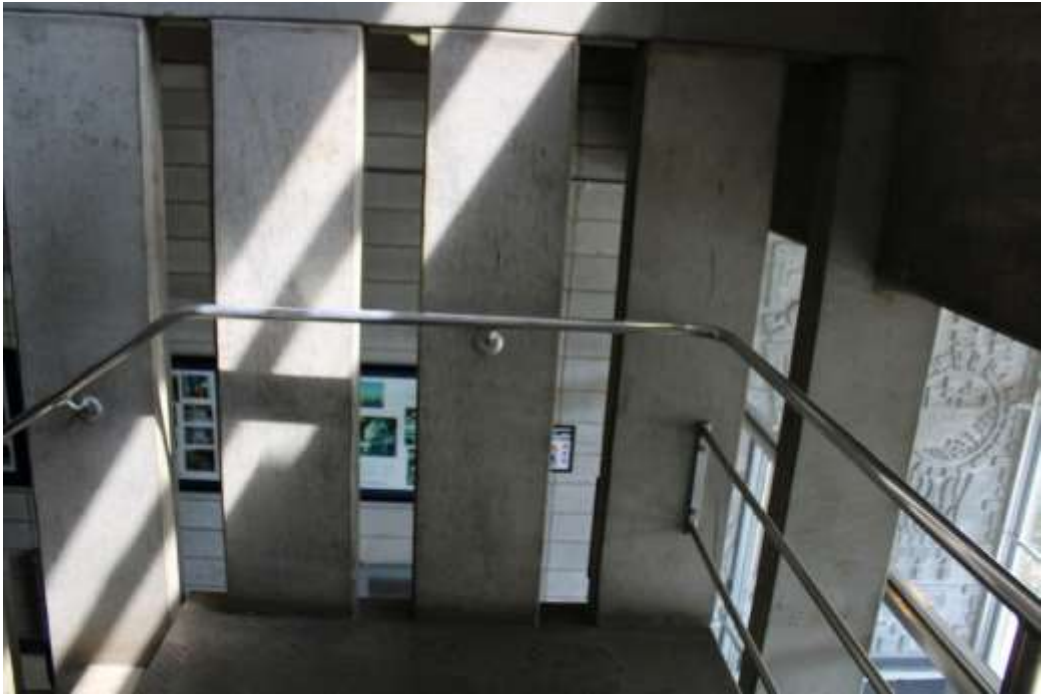
Photograph 18: Concrete staircase linking the balcony levels at the east end of the laboratory.
