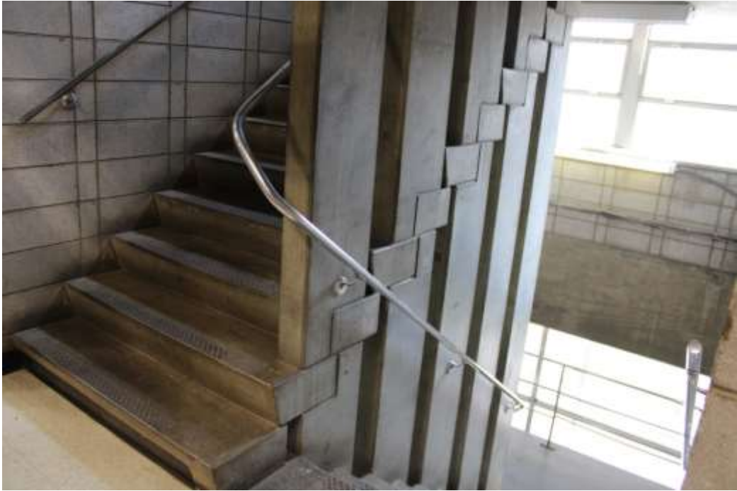
Photograph 17: Concrete staircase linking the balcony levels at the east end of the laboratory.
