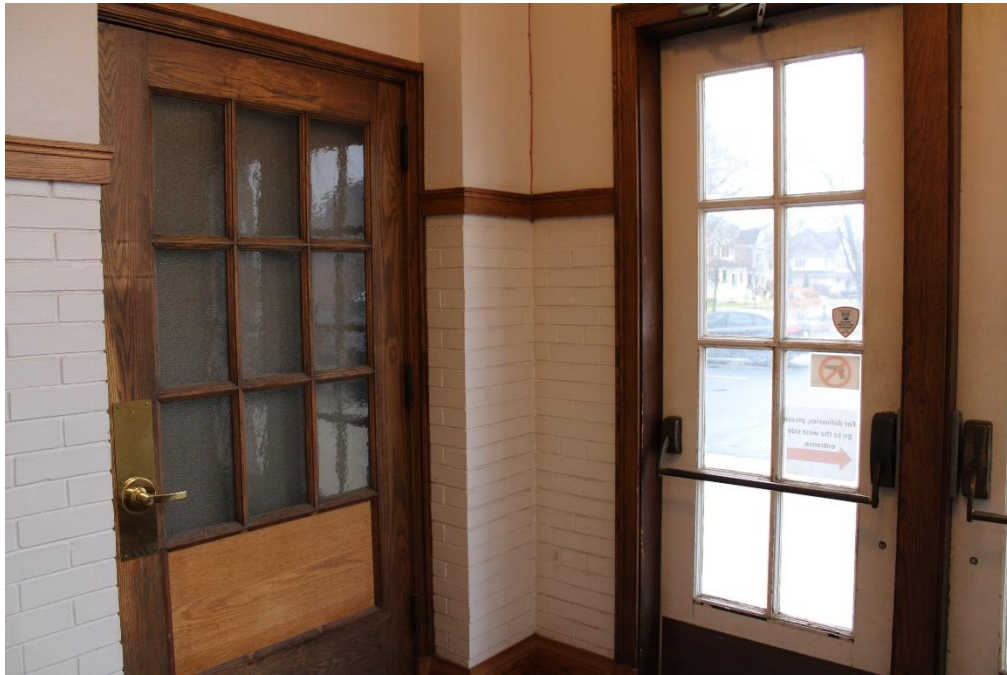
Photo 36: East wing's south entrance vestibule. The door on the left originally opened onto the waiting room for the nurse's office.
