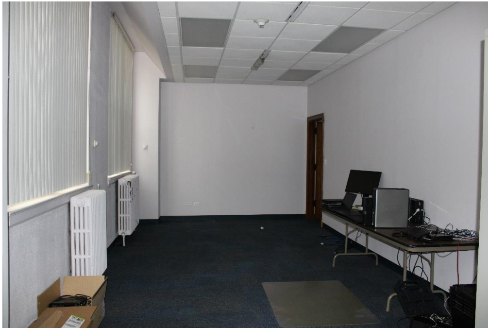
Photo 42: First floor space in the south half of the east wing. This space was originally subdivided into three rooms: principal's office, teachers' room, and nurse's office.
