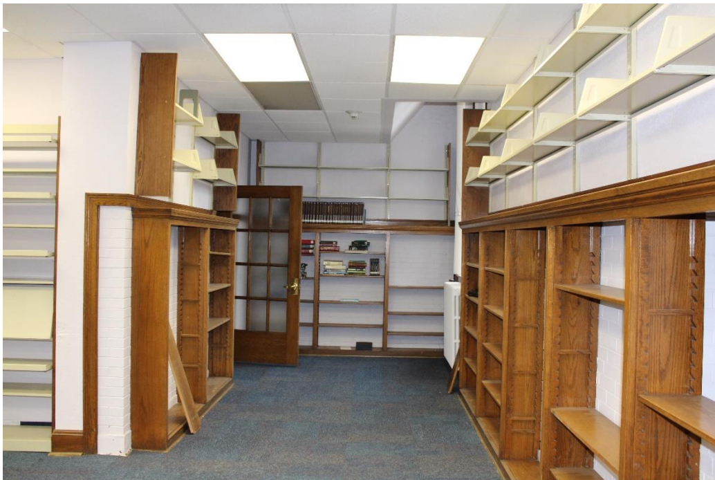
Photo 45: Section of a second-floor room in the south half of the east wing, view south. This space replaced a corridor that originally led to a classroom, the door to which is shown on the left.
