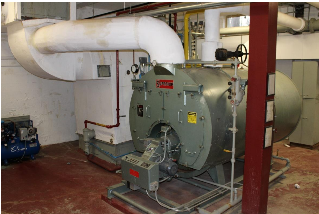
Photo 64: Basement furnace room.
