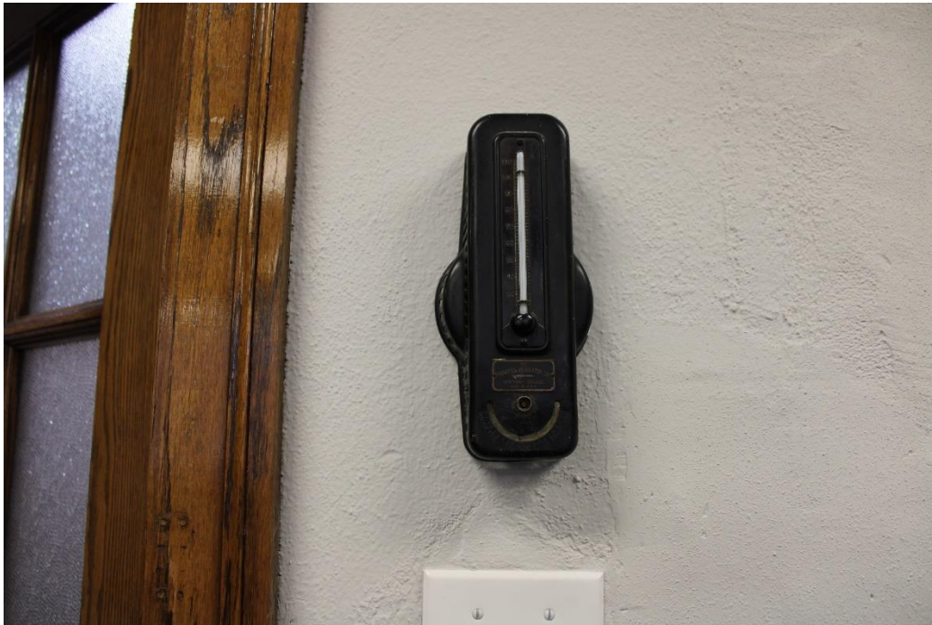
Photo 32: Original thermostat in a former classroom space.
