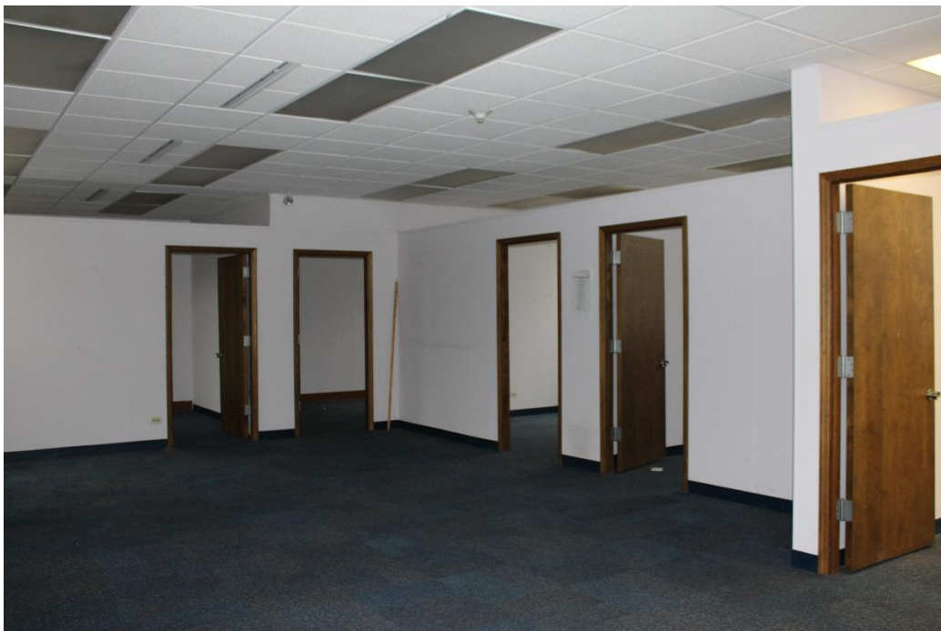
Photo 47: Large second-floor meeting room opening onto offices in the north half of the east wing. These spaces replaced the original music room.
