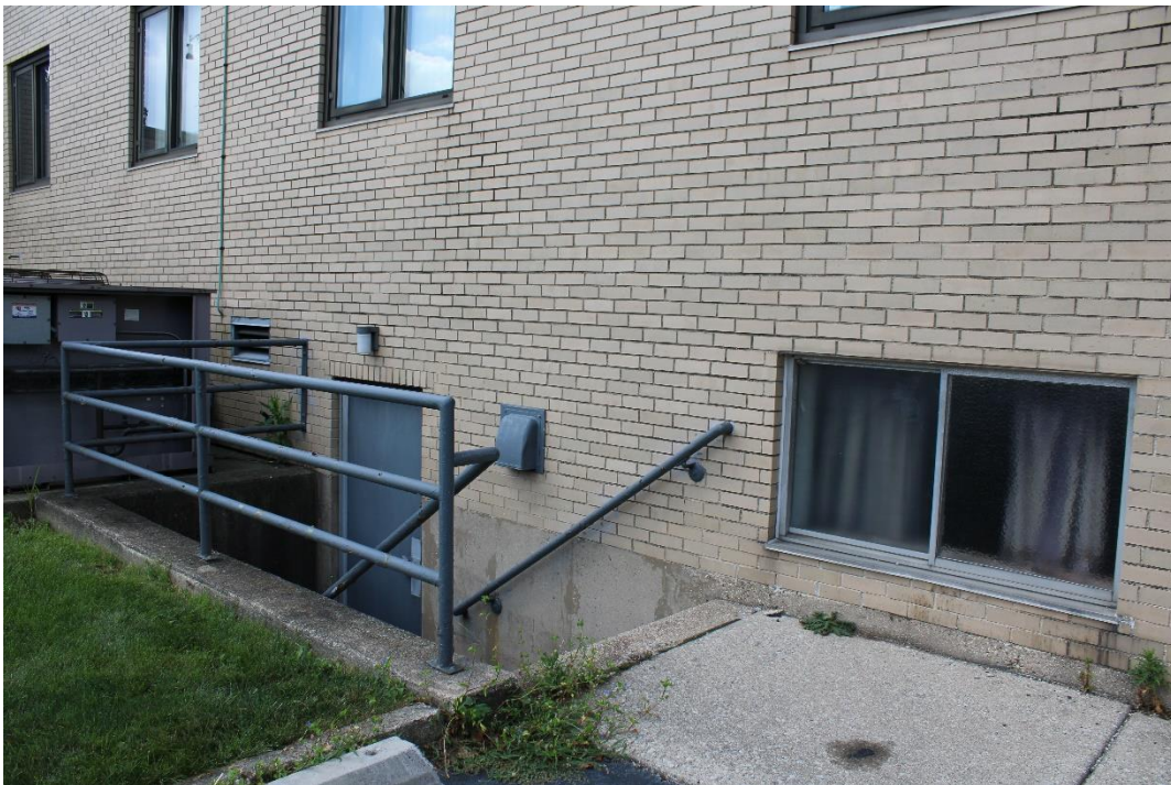
Figure 17: Stairway to lower level entrance along the east façade of the west wing.
