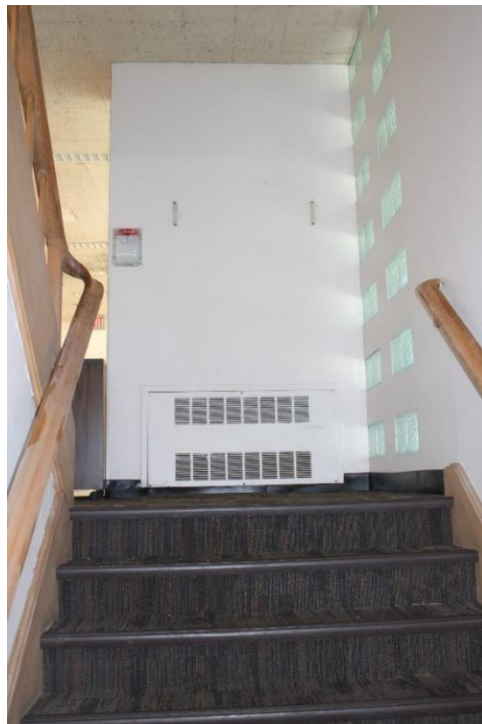
Figure 53: Stairway from lower level to first floor showing vertical strips of glass block on the right.
