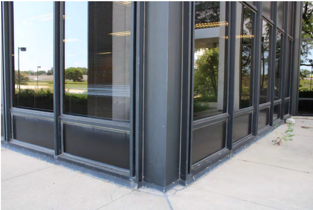
Figure 22: South Plaza Complex, corner of I building's first floor showing window wall details.
