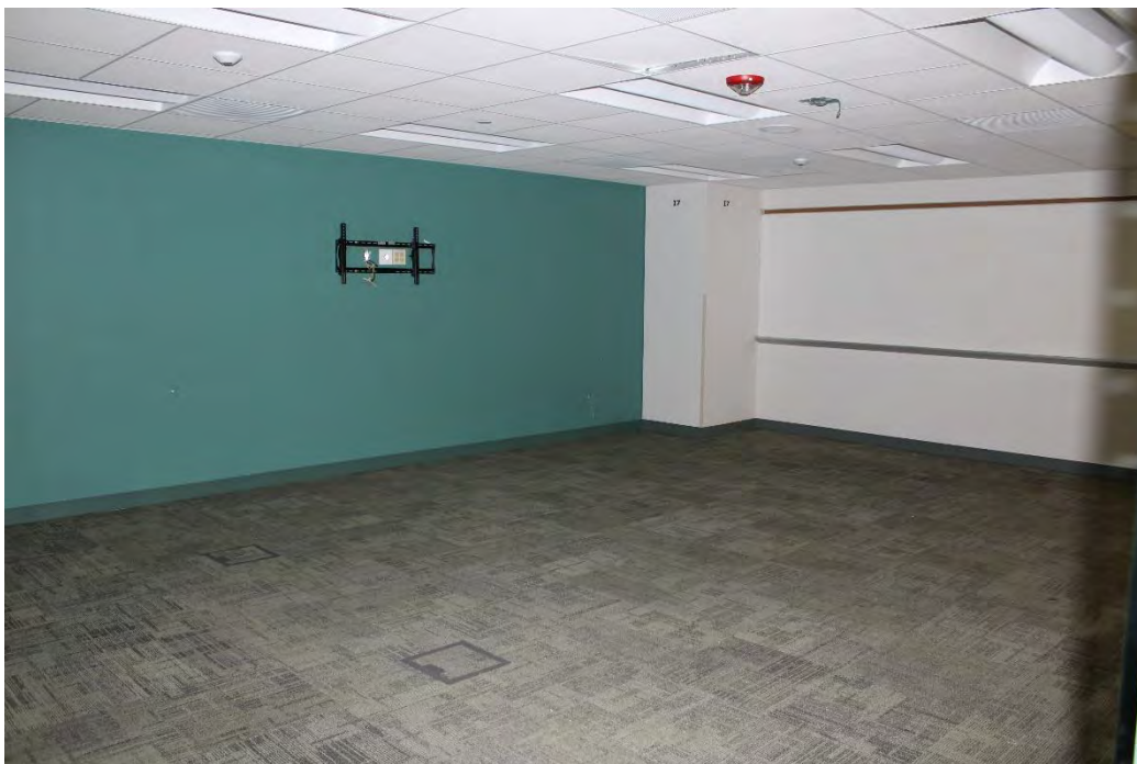
Figure 16: Willow (aka Nielsen) Plaza Building, typical lower level meeting room,
