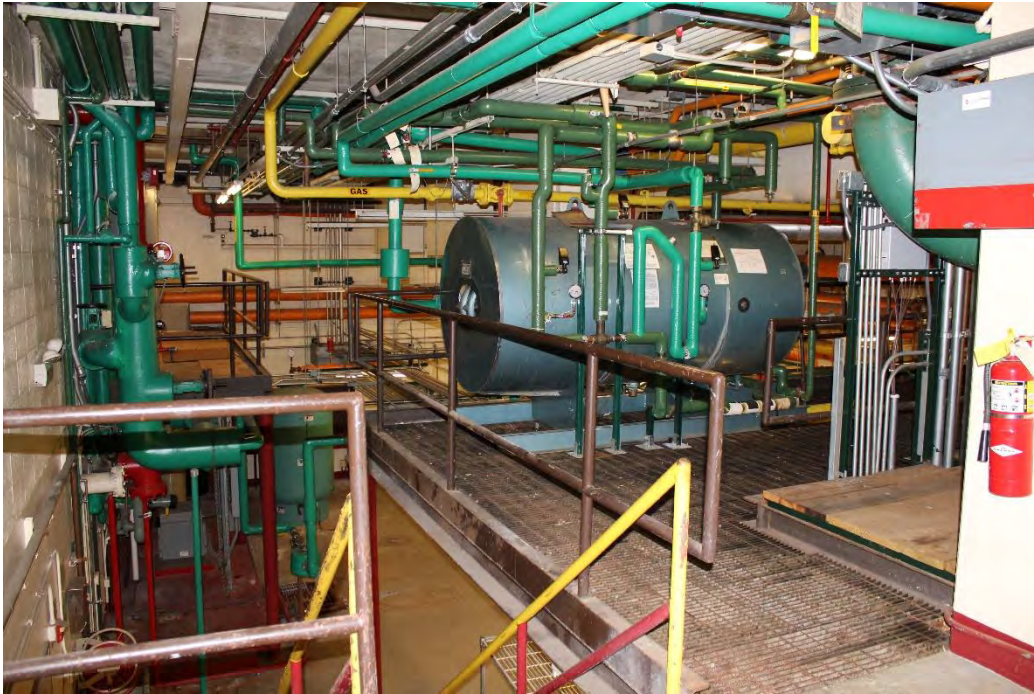
Figure 19: Willow (aka Nielsen) Plaza Building, mechanical room on lower level.
