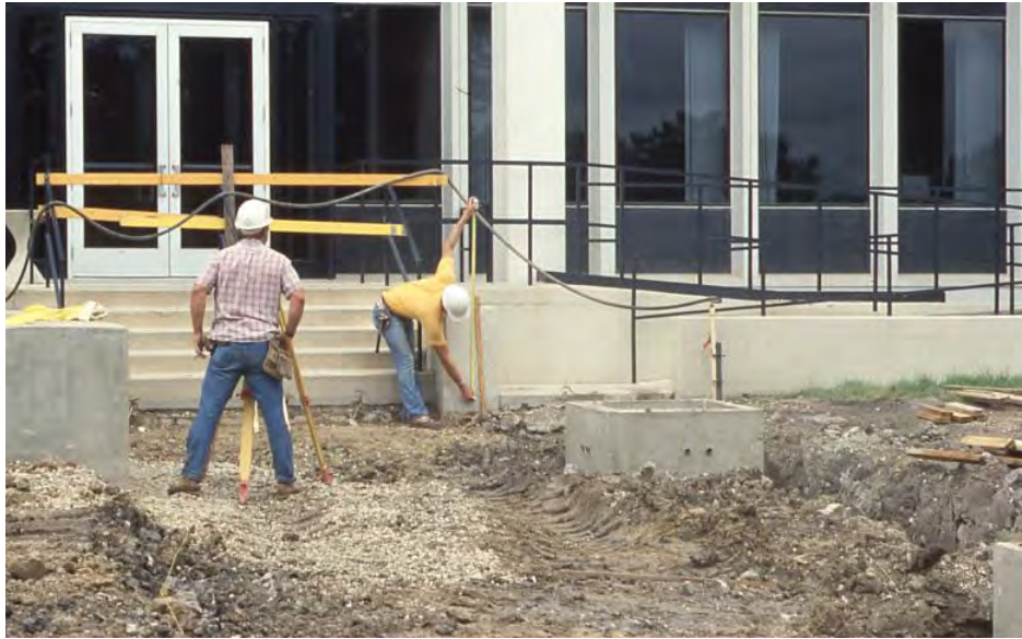
Figure 28: One of the North Plaza complex's buildings under construction. Photo courtesy of the Allstate Corporation Archive.
