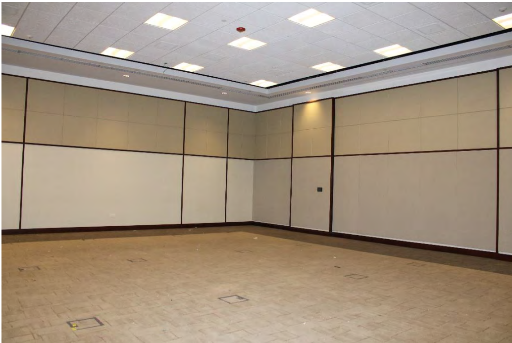
Figure 40: North Plaza Complex, typical conference room on 2 nd floor of C building.
