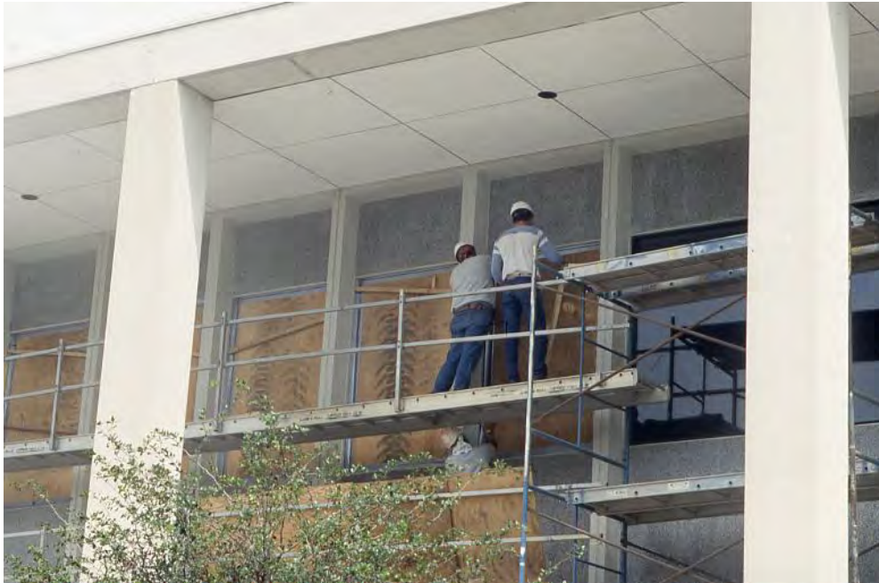
Figure 30: One of the North Plaza complex's buildings under construction. Photo courtesy of the Allstate Corporation Archive.
