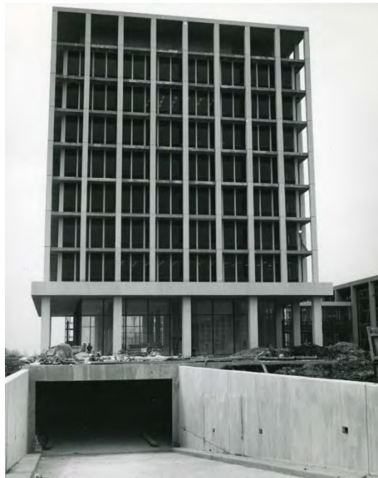
Figure 21: North Plaza's Building F and its underground garage under construction. Photo courtesy of the Allstate Corporation Archive.
