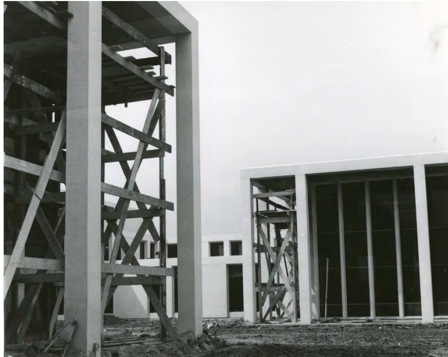
Figure 26: North Plaza complex under construction. Photo courtesy of the Allstate Corporation Archive.
