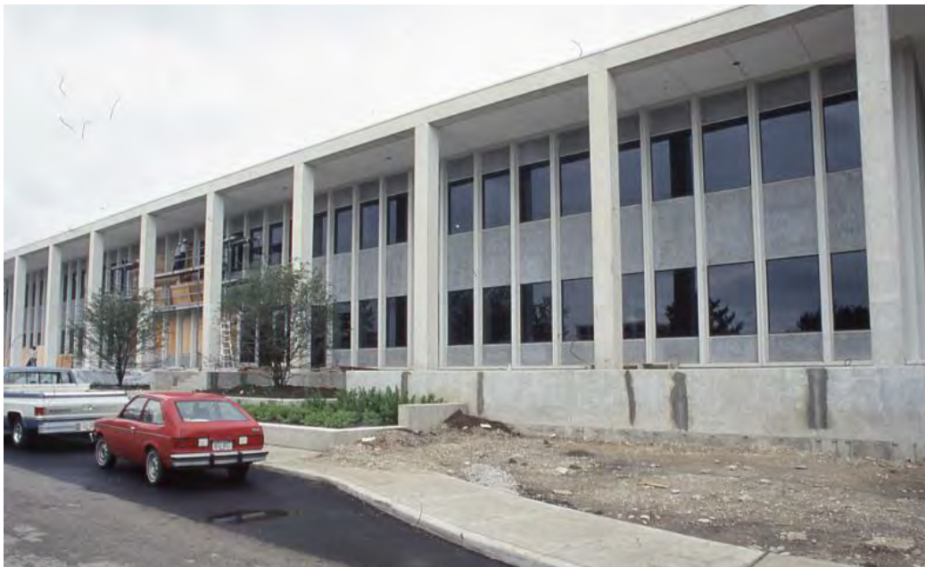
Figure 29: One of the North Plaza complex's buildings under construction. Photo courtesy of the Allstate Corporation Archive.
