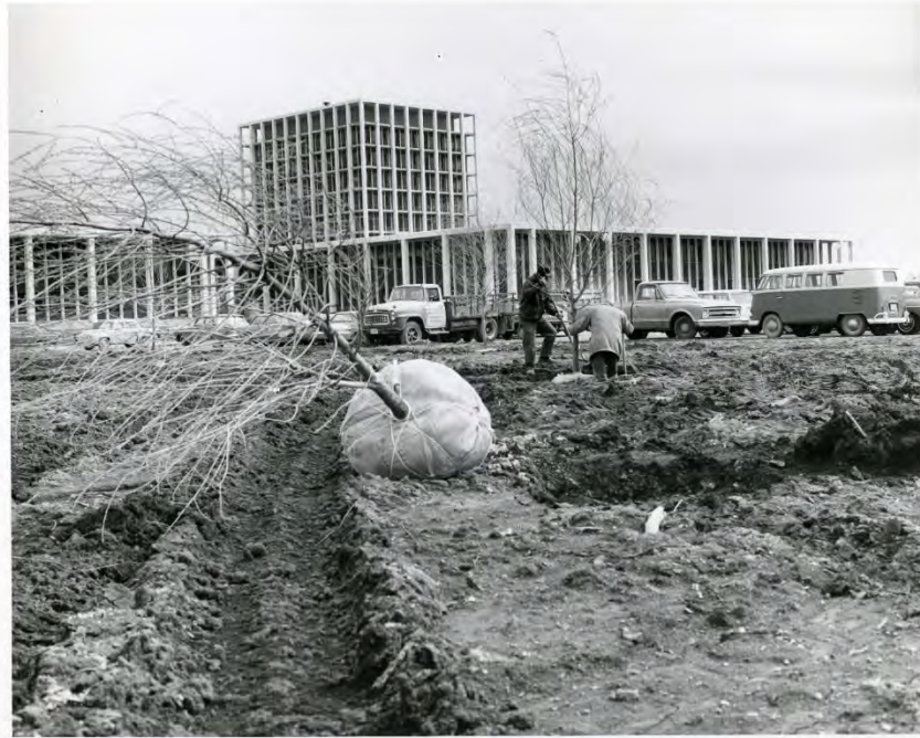
Figure 20: North Plaza complex under construction. Photo courtesy of the Allstate Corporation Archive.
