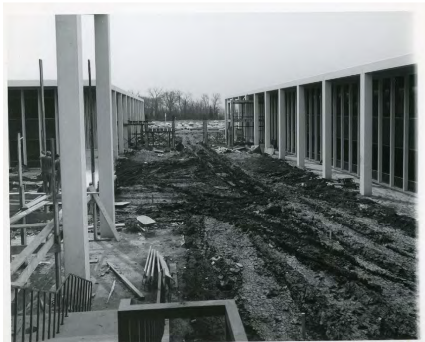
Figure 23: North Plaza complex under construction. Photo courtesy of the Allstate Corporation Archive.
