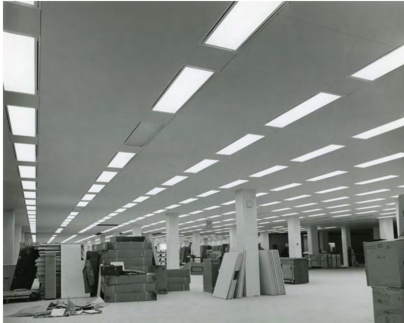
Figure 24: Interior of unidentified North Plaza building under construction. Photo courtesy of the Allstate Corporation Archive.
