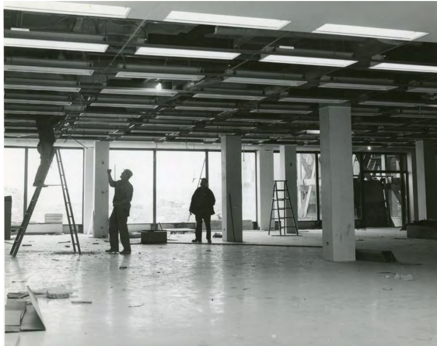
Figure 22: One of the North Plaza buildings under construction. Photo courtesy of the Allstate Corporation Archive.
