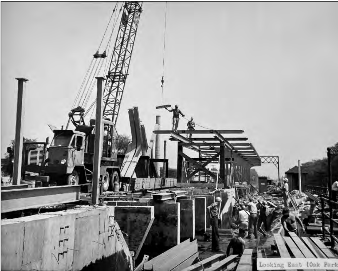
Figure 8: Construction of the Oak Park platform and canopy atop concrete footers within the embankment, 1962. CTA Photo 325-62 #8.
