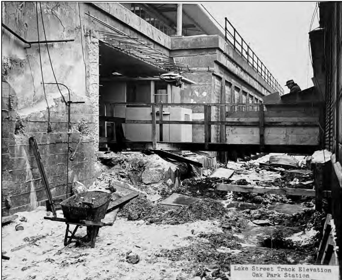
Figure 10: Removal of a portion of the concrete wall of the embankment to construct the Oak Park Stationhouse in 1963. Note the customer assistant kiosk, which has already been installed. A bridge connects the new station to the old wooden platform. CTA Photo 111-63 #18.
