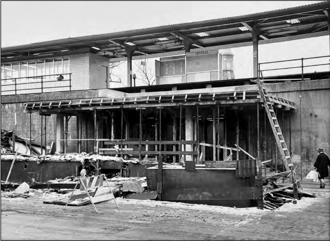
Figure 11: Construction of the Central Stationhouse in 1962. Note formwork for the steel-reinforced concrete roof. CTA Photo 111-63 #30.
