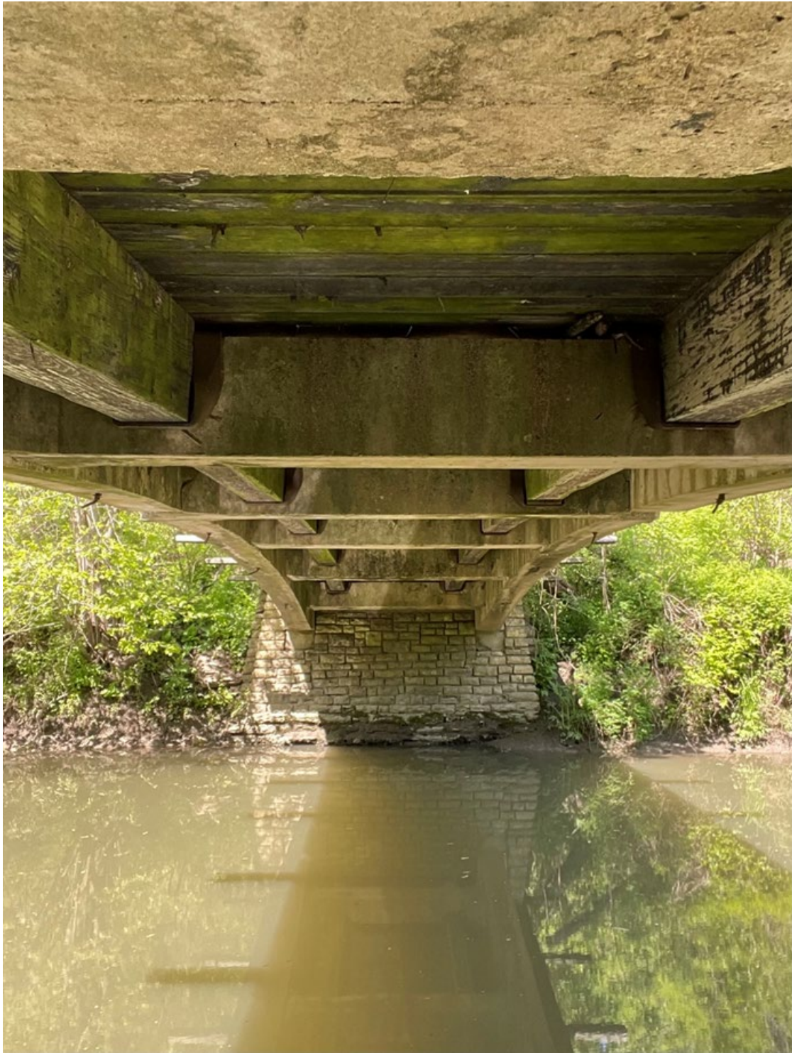
Figure 6. Looking north from underneath the footbridge towards the south abutment. Photograph by Joseph. S. Murphey, USACE.
