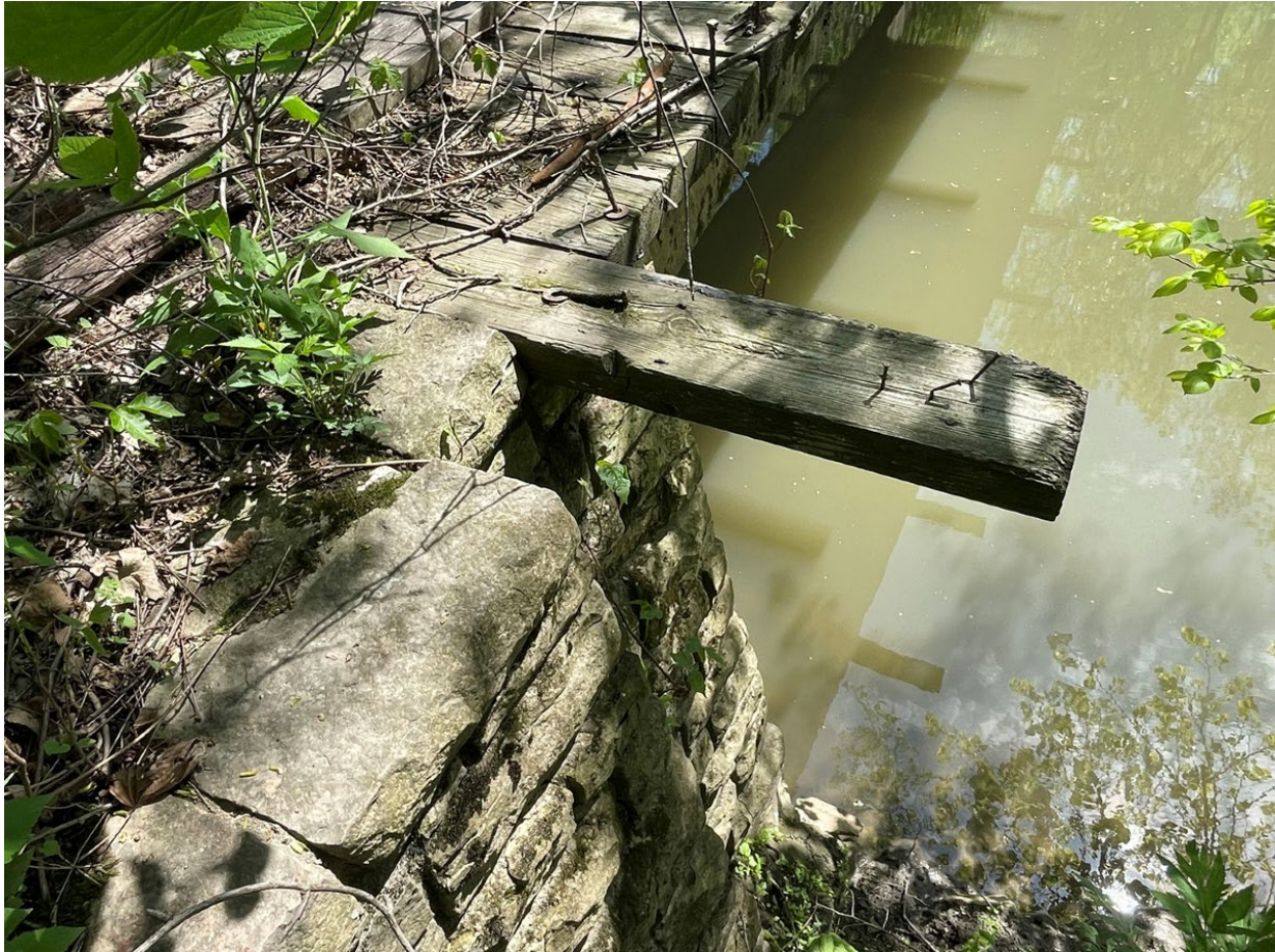
Figure 4. Detail view of the west side of the north abutment. Photograph by Joseph S. Murphey, USACE.
