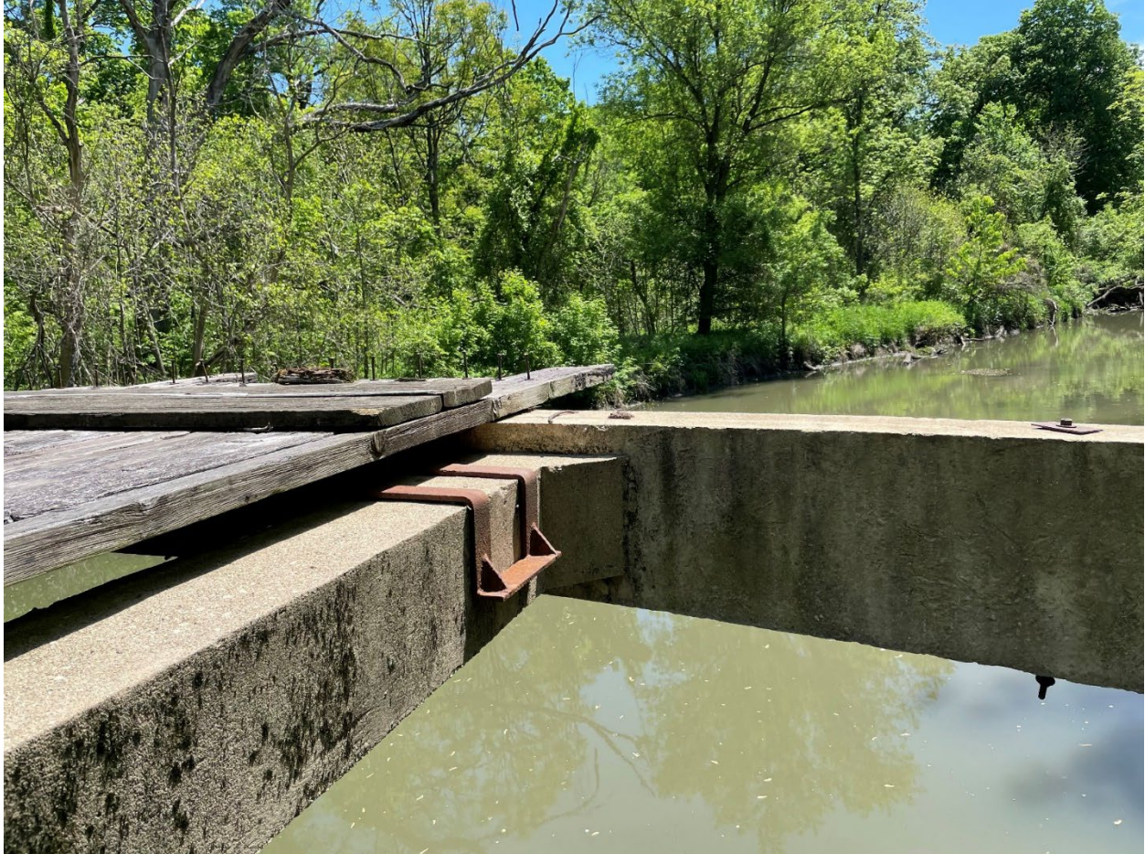
Figure 5. Detail view looking northeast from the southside of the footbridge showing missing bridge deck that exposes the concrete structural system and the iron joist hanger. Photograph by Joseph S. Murphey, USACE.
