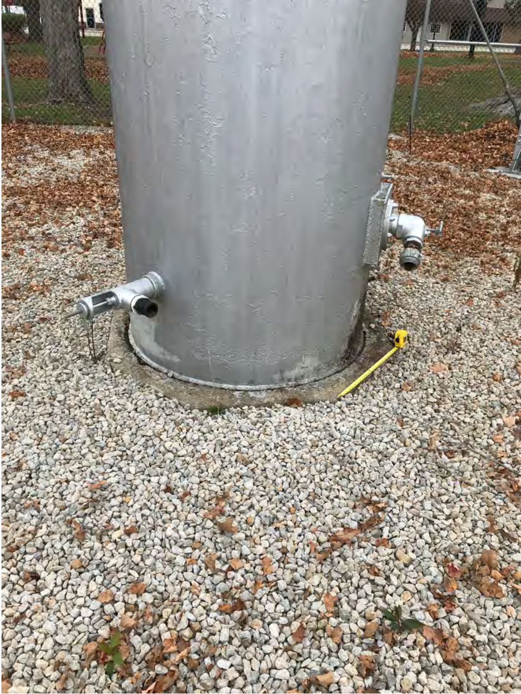
HAER No. IL-1201-23: Base of riser with blowout valves
