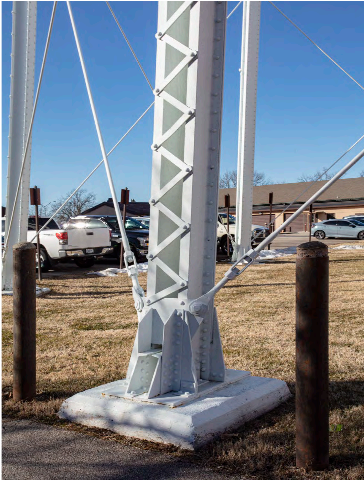
Figure 13: Detail view of the welded steel columns of Water Tower 8010 at the southwest corner of the tower, January 2020.
