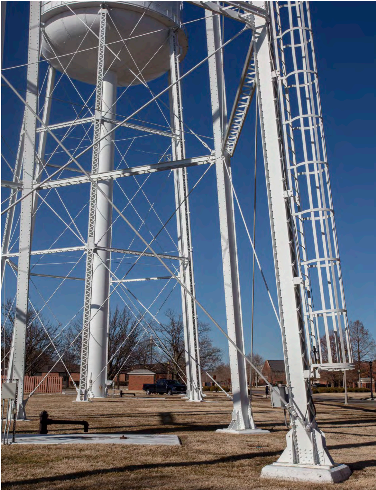
Figure 11: Detail view of the welded steel columns of Water Tower 8010 at the southeast corner of the tower, January 2020.
