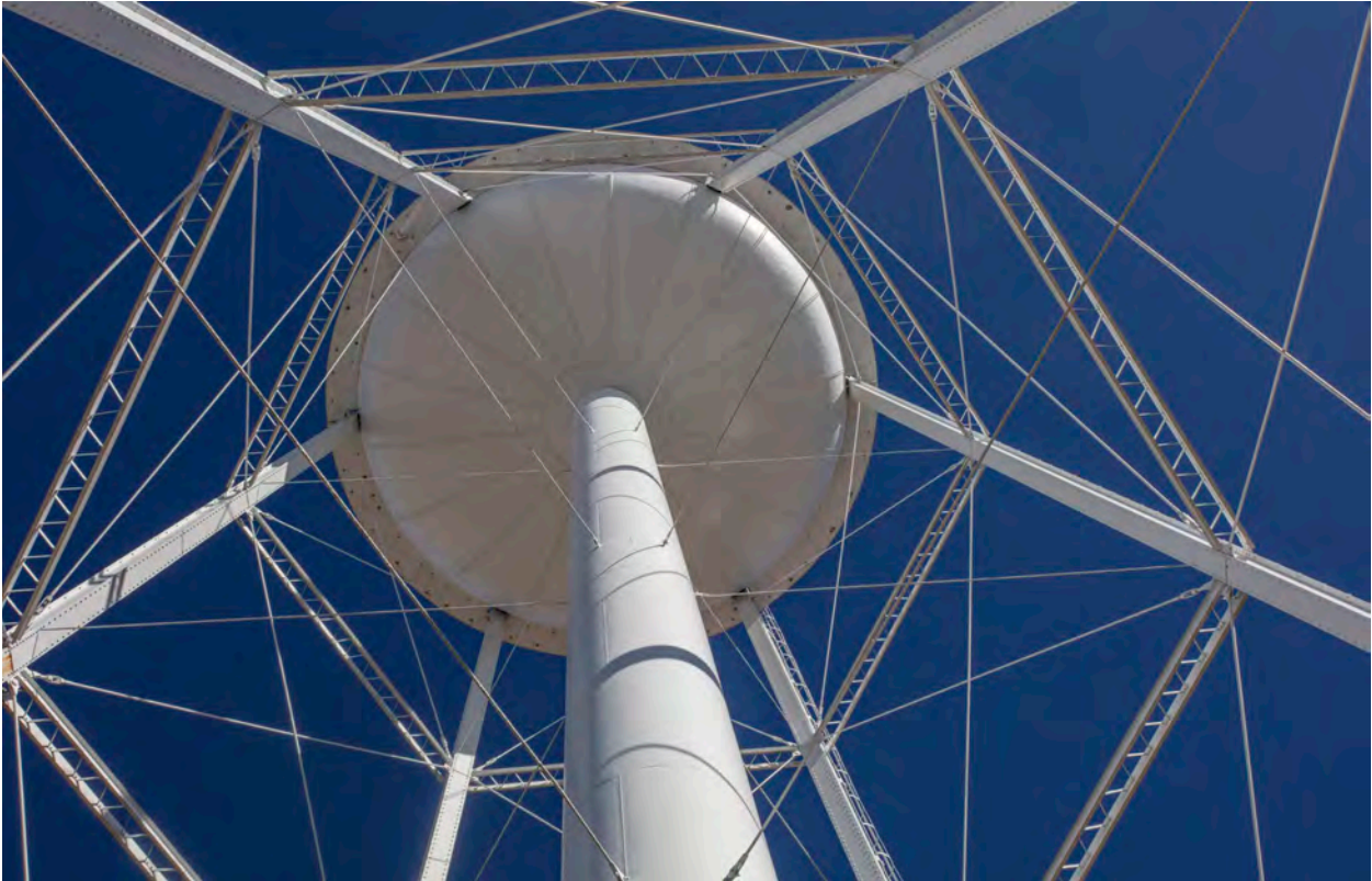
Figure 12: Detail view of the welded steel structure and base of the elevated storage tank of Water Tower 8010 looking up, January 2020.
