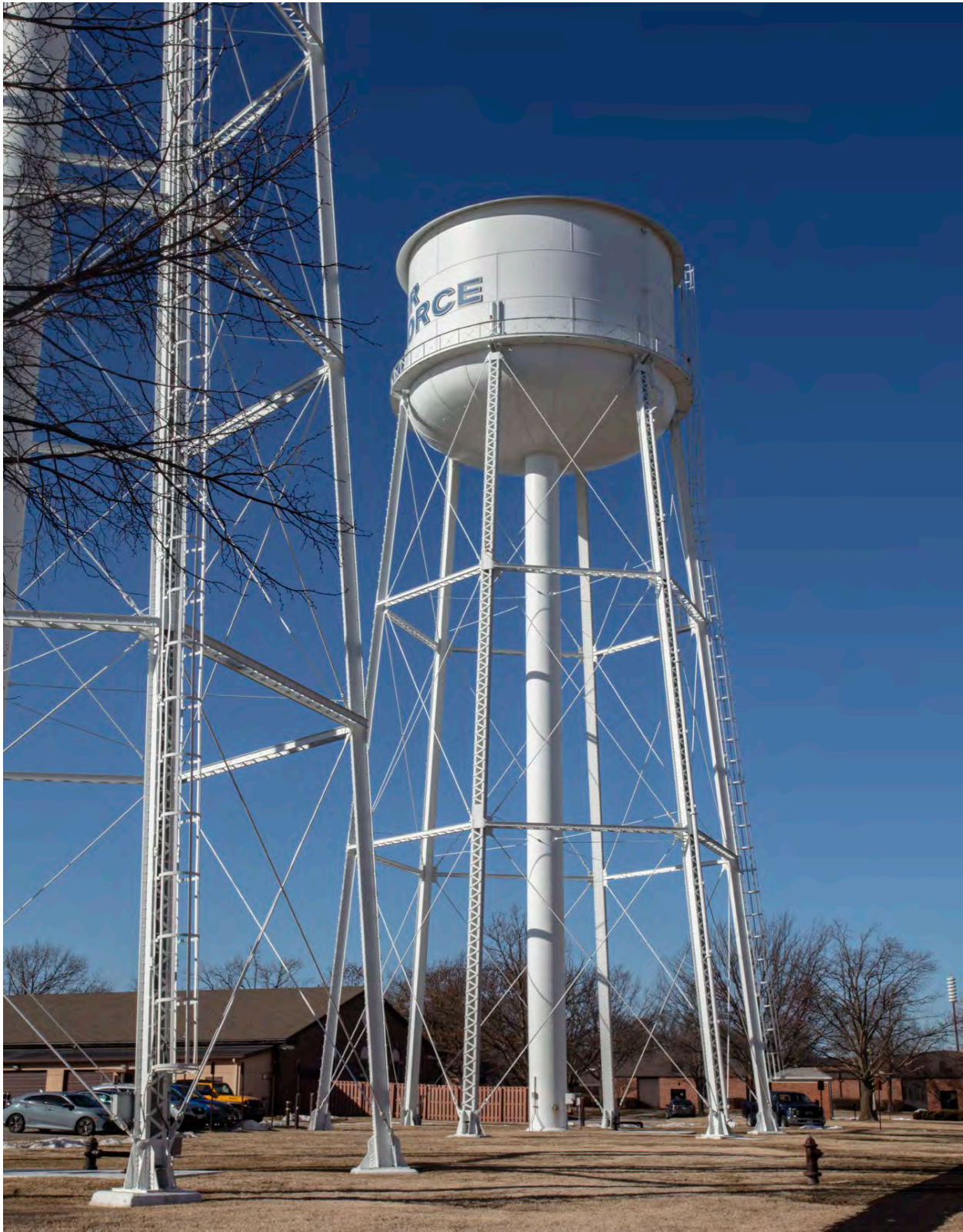
Figure 9: View of Water Tower 8020 looking northwest from the west side of Hangar Road at the entrance to the parking lot, January 2020.
