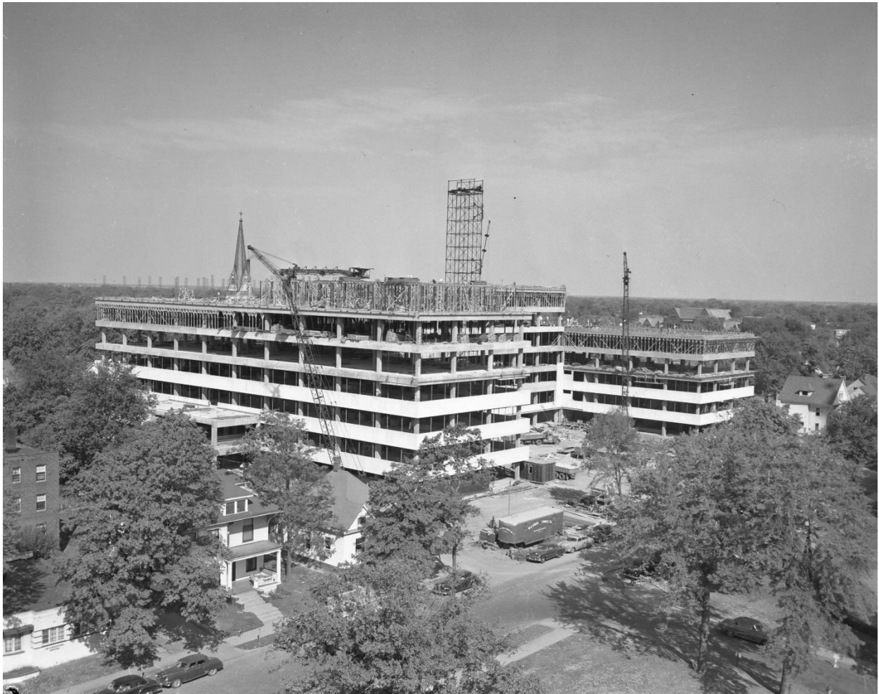
Figure 15. Construction in progress, 1954, view from the southeast. Also note houses and apartment buildings lining Spring Street to the north and south.
