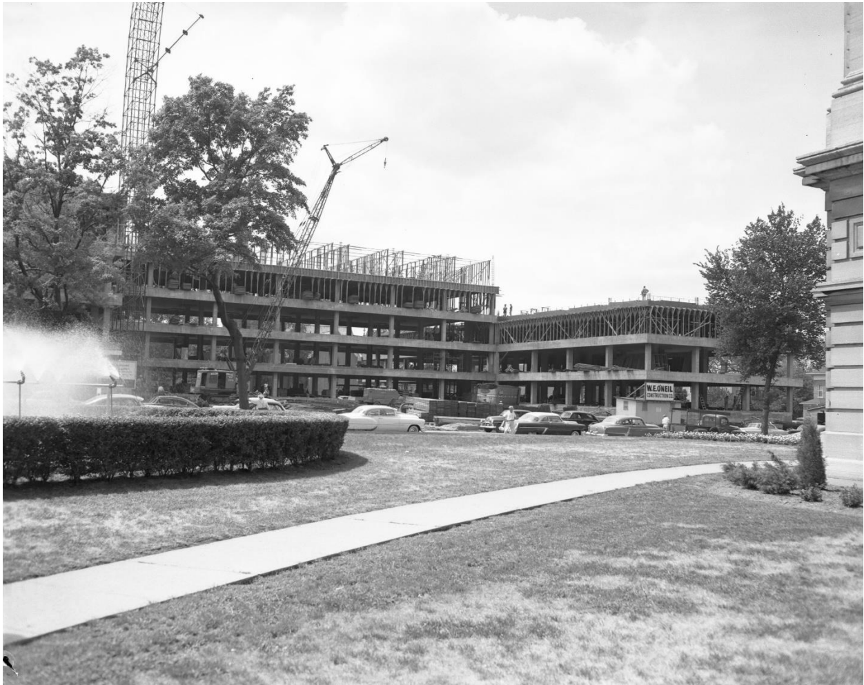
Figure 14. The concrete structural frame of the building takes shape, 1954, view from the southeast, with the corner of the Capitol Complex visible at right.
