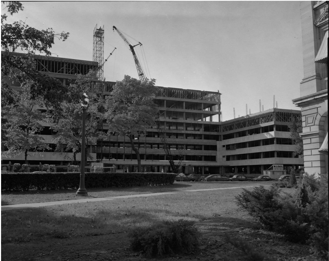
Figure 16. The structure is in progress, and installation of the limestone cladding has begun, 1954, view from the southeast with the corner of the Capitol Complex visible at right.
