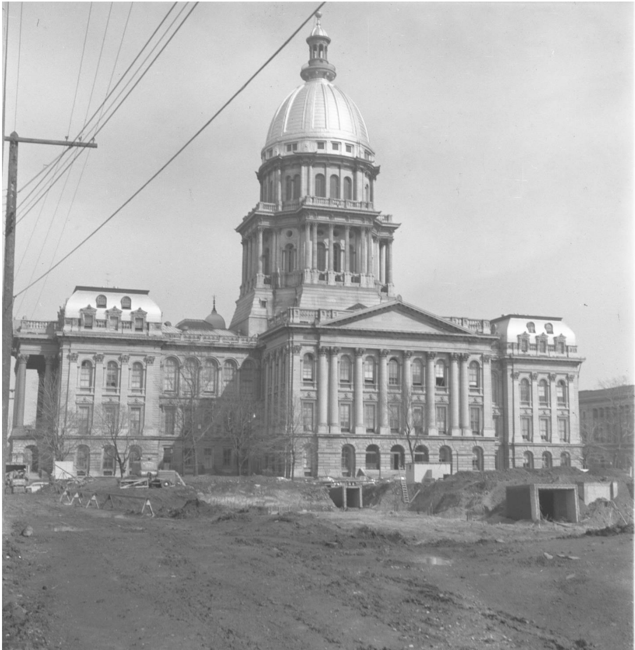
Figure 12. The site for the building is cleared, and construction of the tunnels connecting the capitol has begun, 1954 view from the northwest.
