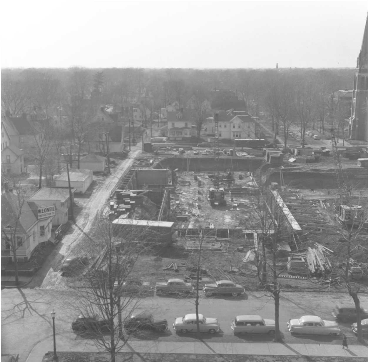
Figure 13. Excavation and construction of the foundation and basement, 1954, view from the east.
