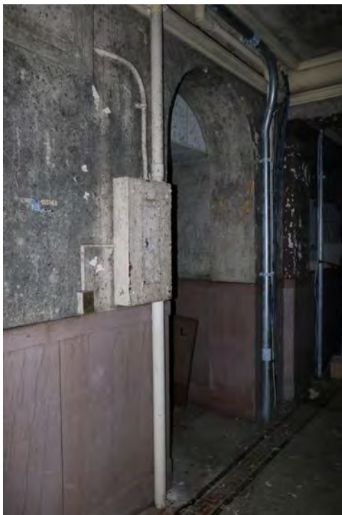
Exhibit F - First floor corridor, showing original arch mosaic floor, and Tennessee marble wainscot
