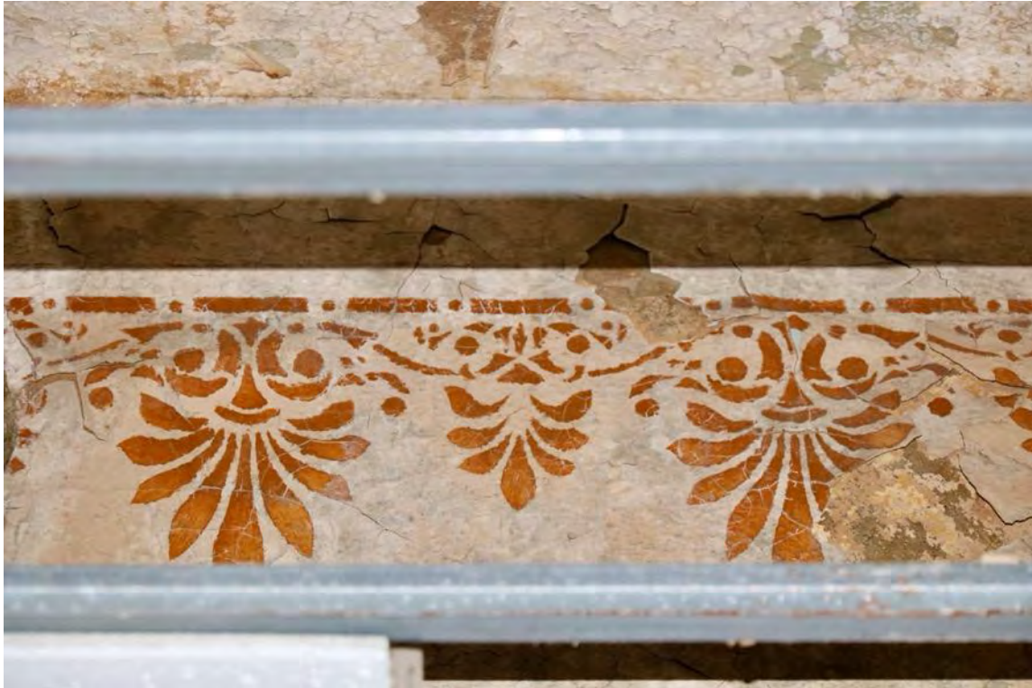
Exhibit R - Historic stencil behind dropped ceiling
