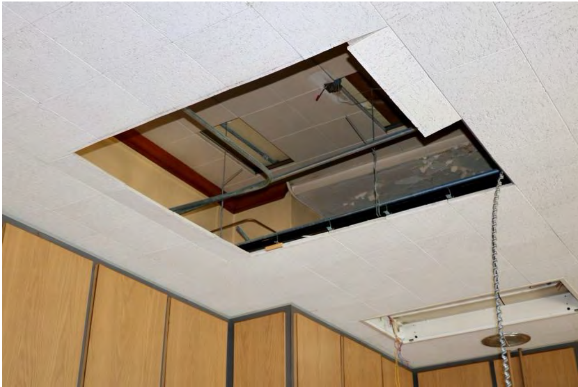
Exhibit K - Second floor northwest courtroom showing multiple layers of ceiling replacement
