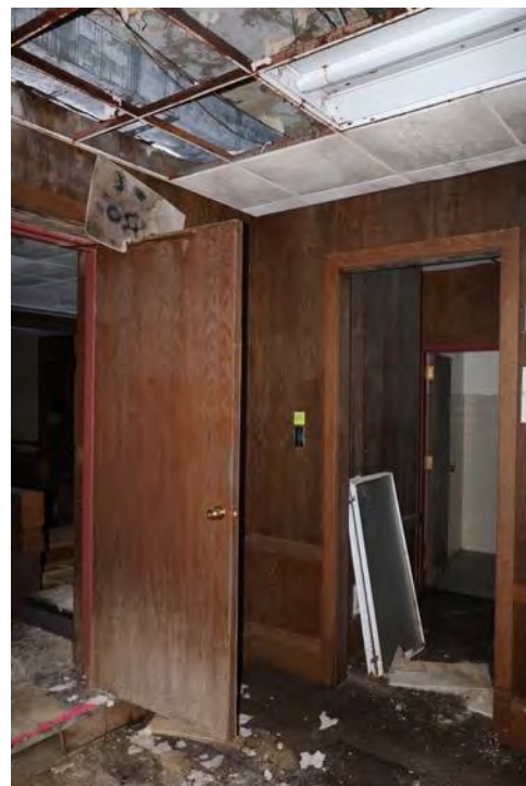
Exhibit G - First floor chambers vestibule, showing drop ceiling grid, modern wood paneling and doors
