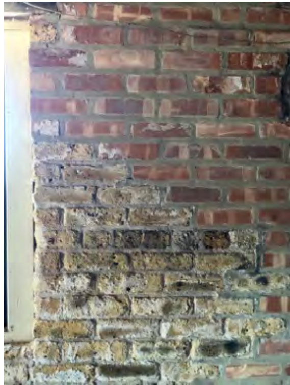
Detail of attic north wall, showing later brickwork repair
