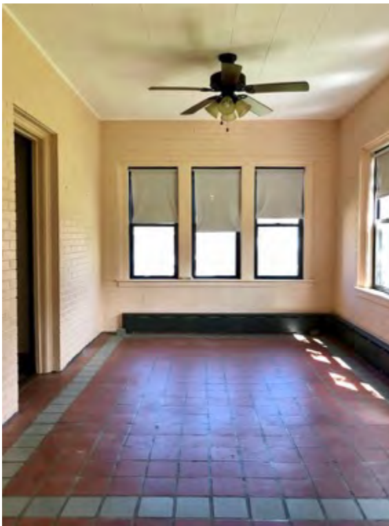
Sun room, showing painted brick walls and terra cotta floor, looking east
