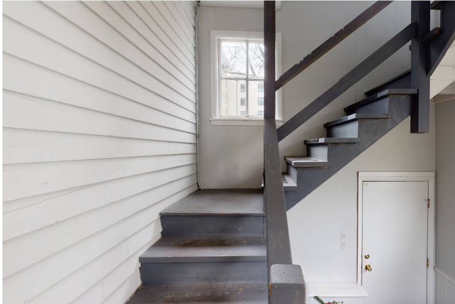
17: General view of rear entrance to the house and staircase, looking west. Wood clapboard siding and a four-lite wood window is visible left of center.
