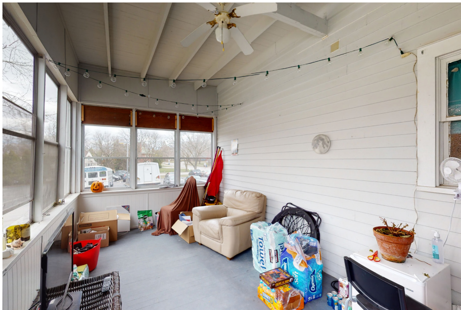
16: General view of first floor sleeping porch, looking east. Wood clapboard siding is right of center, and painted wood flooring and framing remain partially visible throughout.
