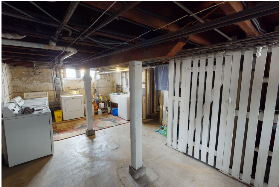
24: General view of basement, looking southeast. A portion of the limestone foundation is visible in the background.
