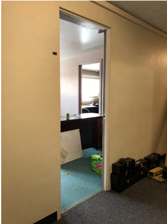
Figure 15: Flush-finished door jambs
