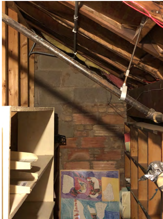
Figure 17: Fireproof construction in third floor
