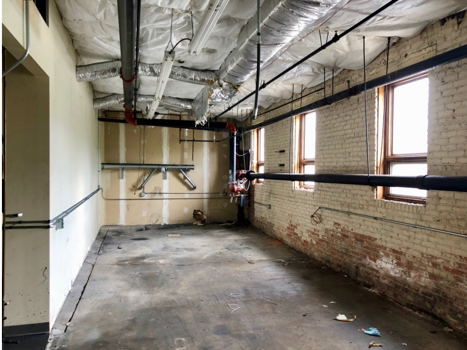
Room C in Section 61a (to be demolished), western section looking south
