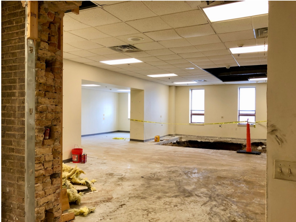
Stamping in Section 61 (to be demolished), showing wall construction of brick, looking east
