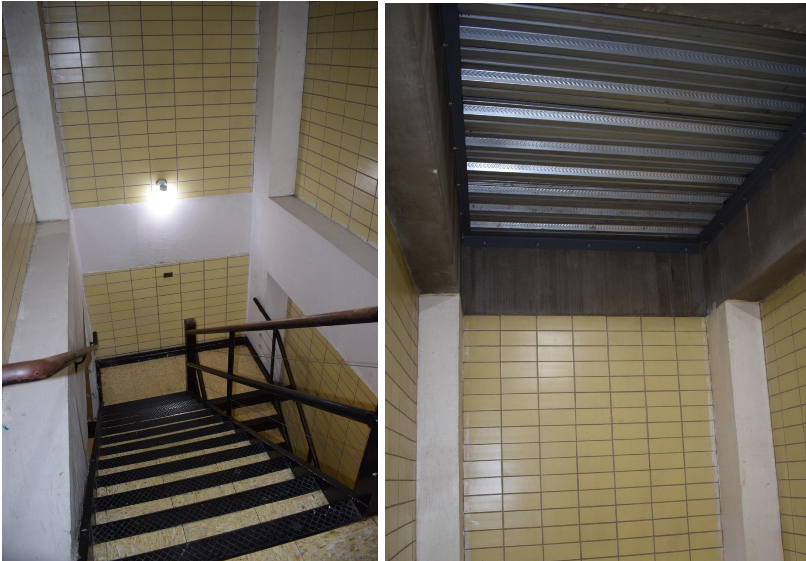
Figure 74. Two views of Stairway No. 1 illustrating the re-enforced concrete frame (columns, girders, and beams), infilled curtain walls of glazed tile, and metal stairs with pipe railings. Note the infilled ceiling of this stairway, which was added in 1976, after the four-story dormitory wing had been completely removed for consideration (2020).
