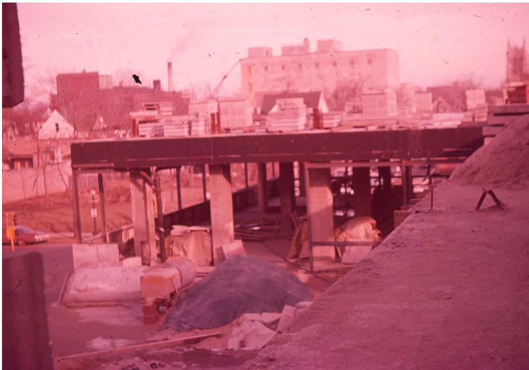
Figure 37. Forming columns, pouring floors, and masonry work enclosing superstructure (summer 1959) (YMCA Color Slides 1959).
