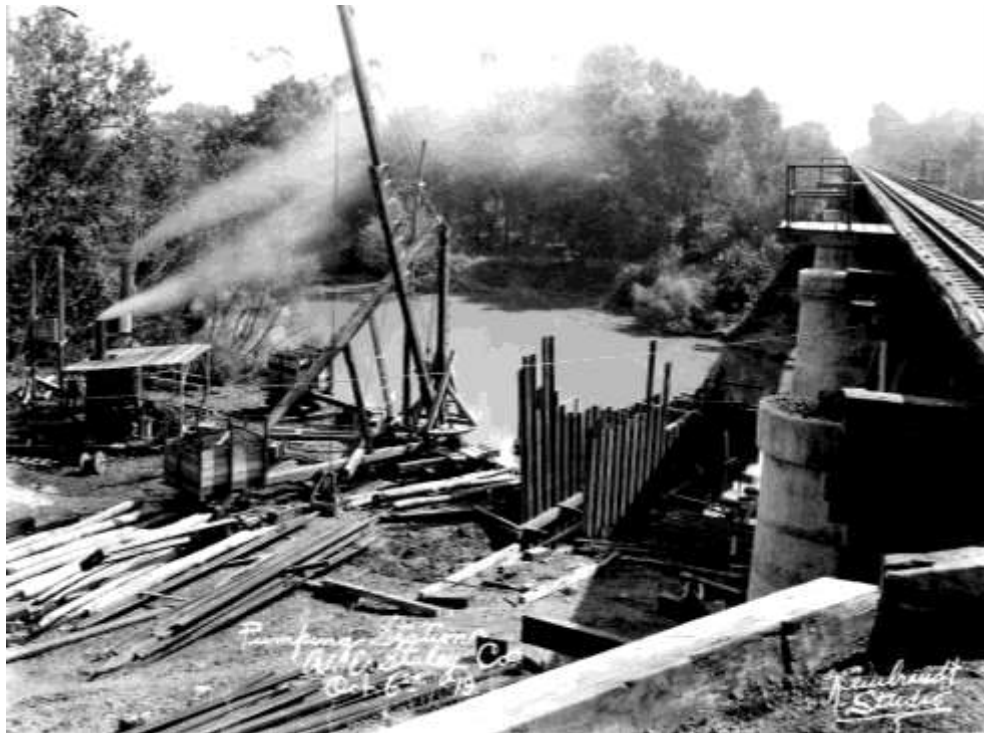
Figure 11. Two views of work on the intake pipe to the Pumping Station, both dated 6 October 1919. The bottom image was published as “View of Work on Pumping Station from the I. C. Tracks” (Staley Museum; Staley Fellowship Journal [November 1919], p. 14).
