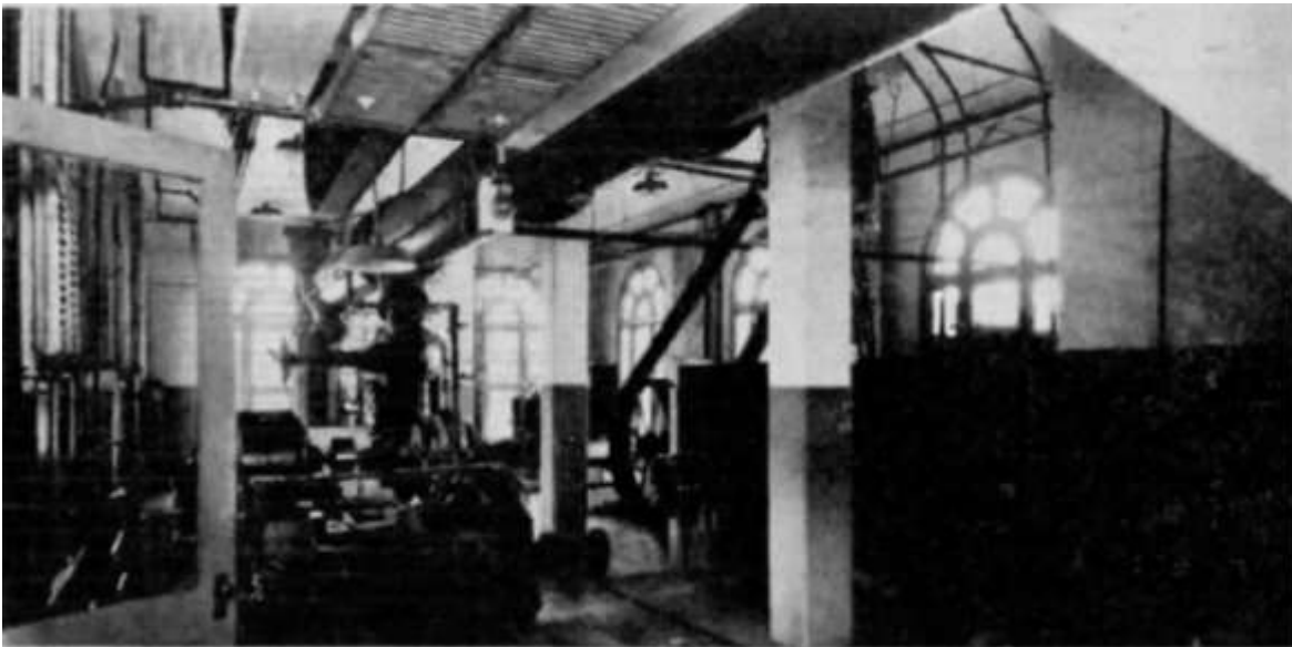
Figure 55. Two early views of the interior of the Staley Pump House, illustrating the interior of the pump room (or “landing”) level of the building (Watson 1923:6). (Top) “First Floor Pumping Station—The two 100 H. P. pumps in the foreground. Intake valves in background.” (Bottom) “First Floor Pumping Station—West End, 150 H. P. pump in foreground.”
