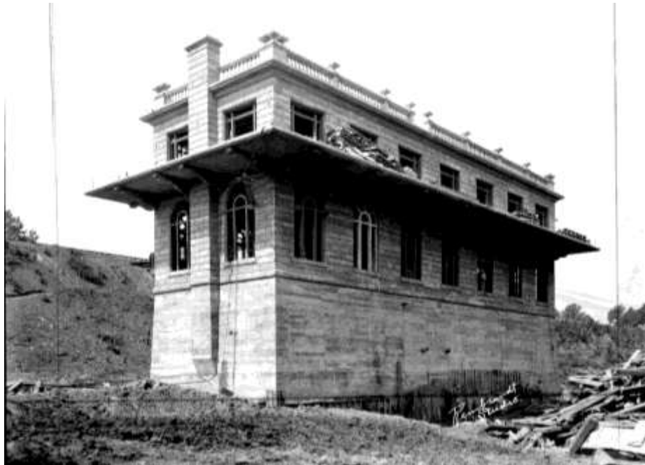
Figure 19. (Top) “The pumping station has finally crept this far above the surface of the ground” ( Staley Fellowship Journal [July 1920], p. 8). This photograph illustrates the scaffolding and wooden forms in place for the pouring of the concrete walls. (Bottom) “The Pumping Station which is rapidly nearing completion.” Southwest view of the building as illustrated in the October 1920 edition of the Staley Fellowship Journal ([October 1920, p.23; Staley Museum). The balustrade around the balcony had yet to be installed at this point. The opening in the roof-line balustrade marks the point to which the exterior stairway was aligned.
