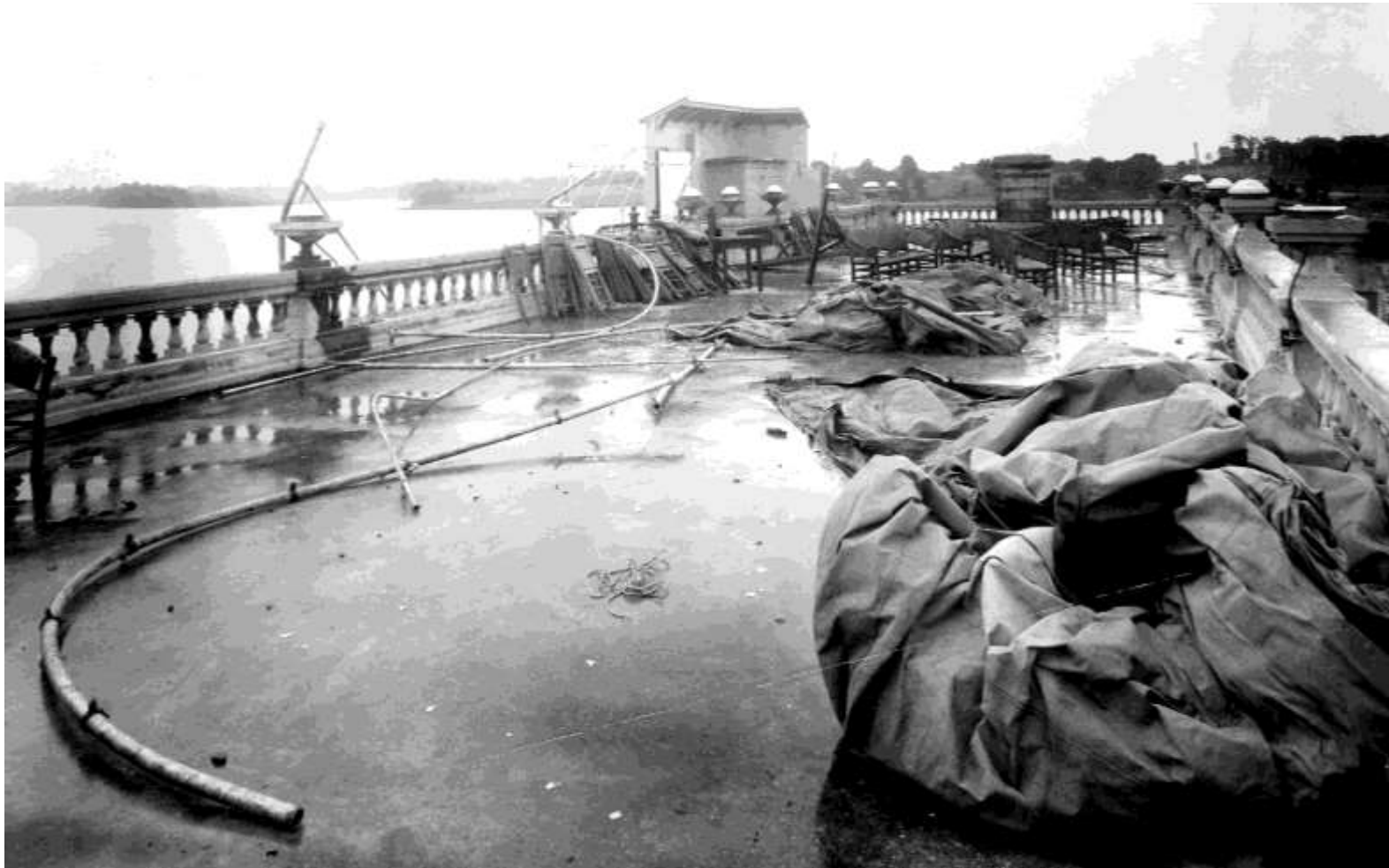
Figure 41. View of Roof Level illustrating storm damaged canopy and a couple of lamp globes (looking east). Note frame toilet structure at the far end, adjacent to the stair landing (Undated [ca. 1929] photograph; Staley Museum).
