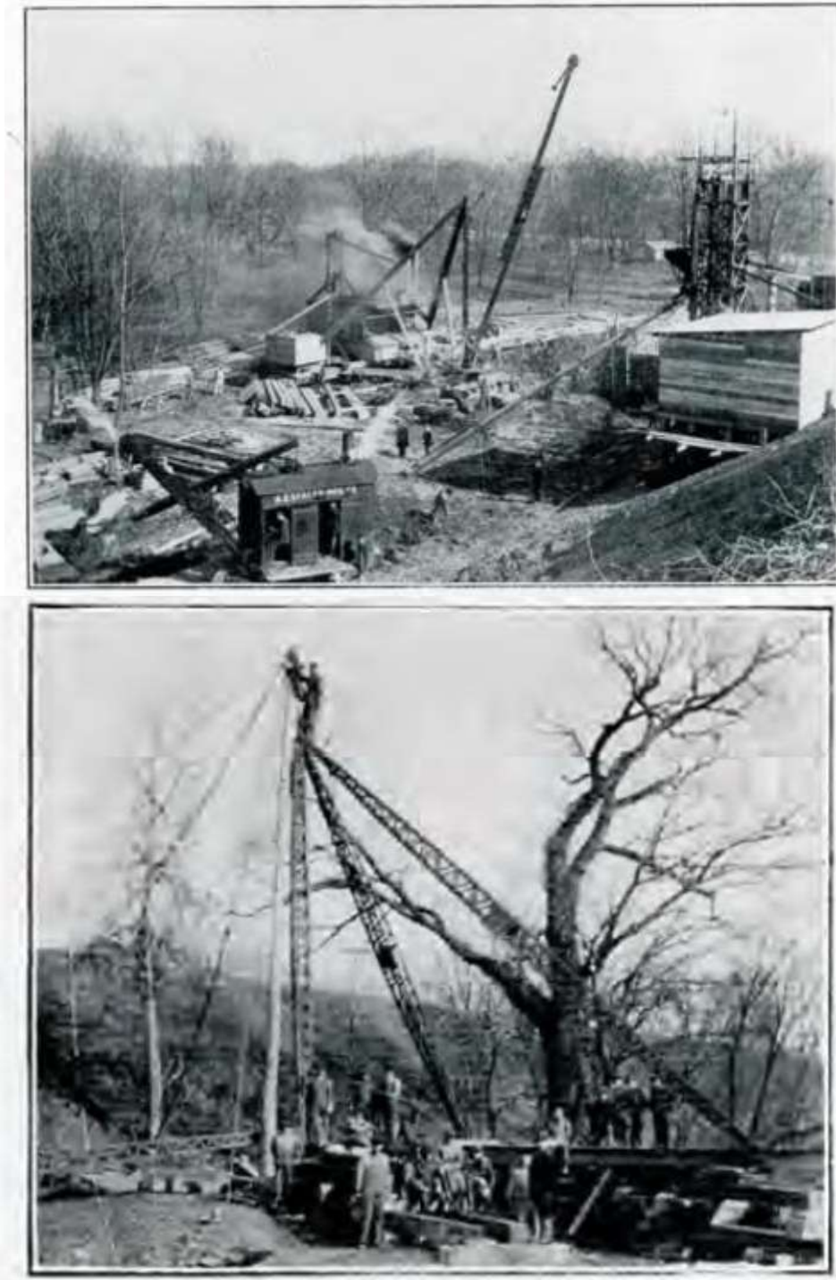
Figure 17. Two photographs of work at the Pumping Station ( Staley Fellowship Journal [April 1920], pp. 11, 17). (Top) “Showing the Steam Shovel Near the End of the Job of Digging the Ditch from the Plant to the Pumping Station.” (Bottom) “Beginning the Construction of Staleys Temporary Dam.” The temporary dam was located immediately to the south of, on opposite side of, the railroad trestle.
