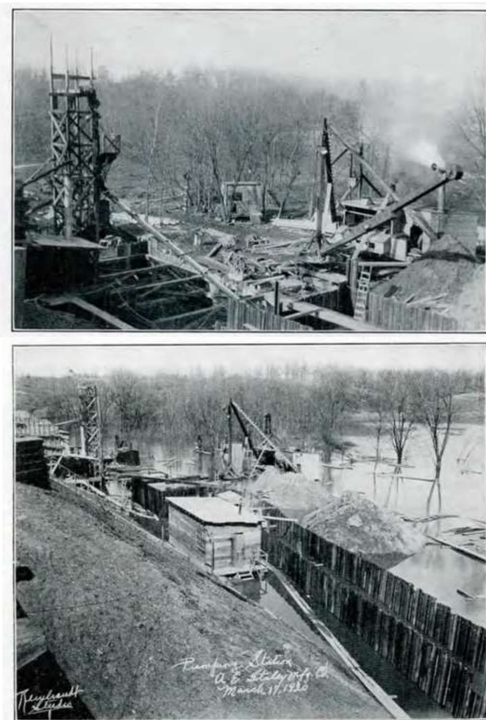
Figure 16. (Top) “Pouring Concrete for the Foundation of the Pumping Station.” (Bottom) Photograph dated March 1920, and with published caption that read: “The River’s Rise of 8 Feet Completely Flooded the Site of the Pumping Station” (Staley Fellowship Journal [April 1920], pp. 2, 16).
