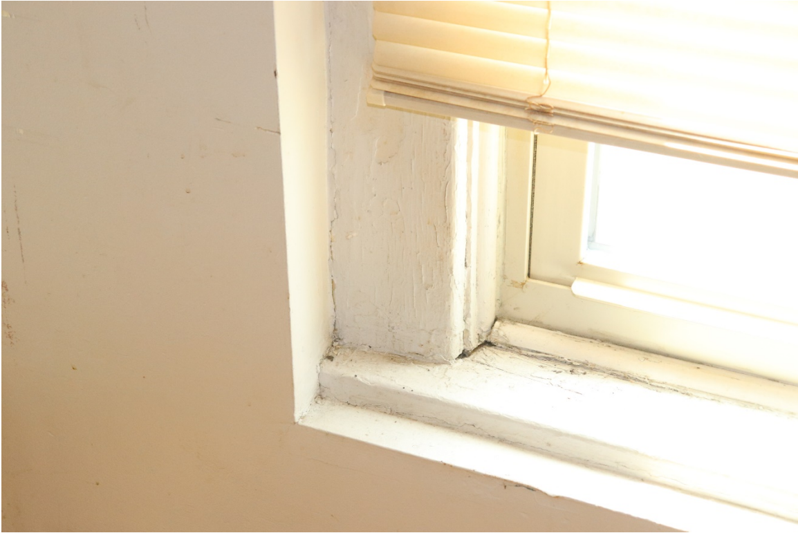
Detail of window casing in bay window of southwest bedroom in Apartment 3
