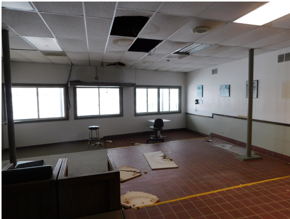
Figure 10: Second story drivers lounge overlooking racetrack.
