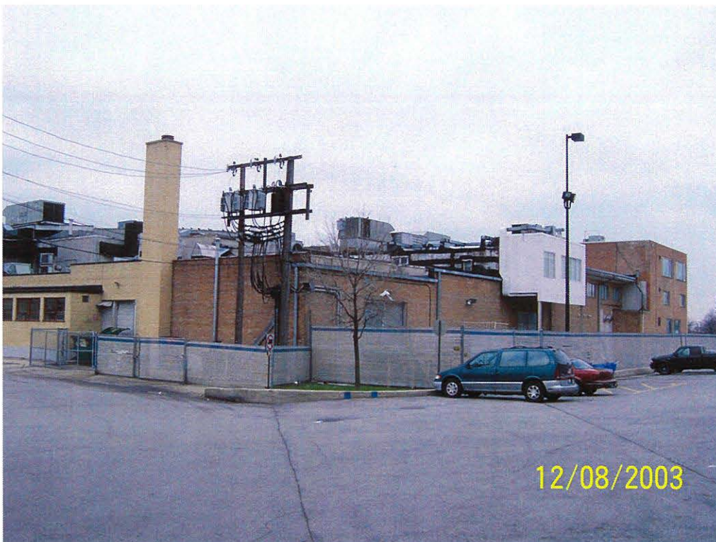
Figure 11. Brick back of original Drury Lane building. The view is to the southwest.
