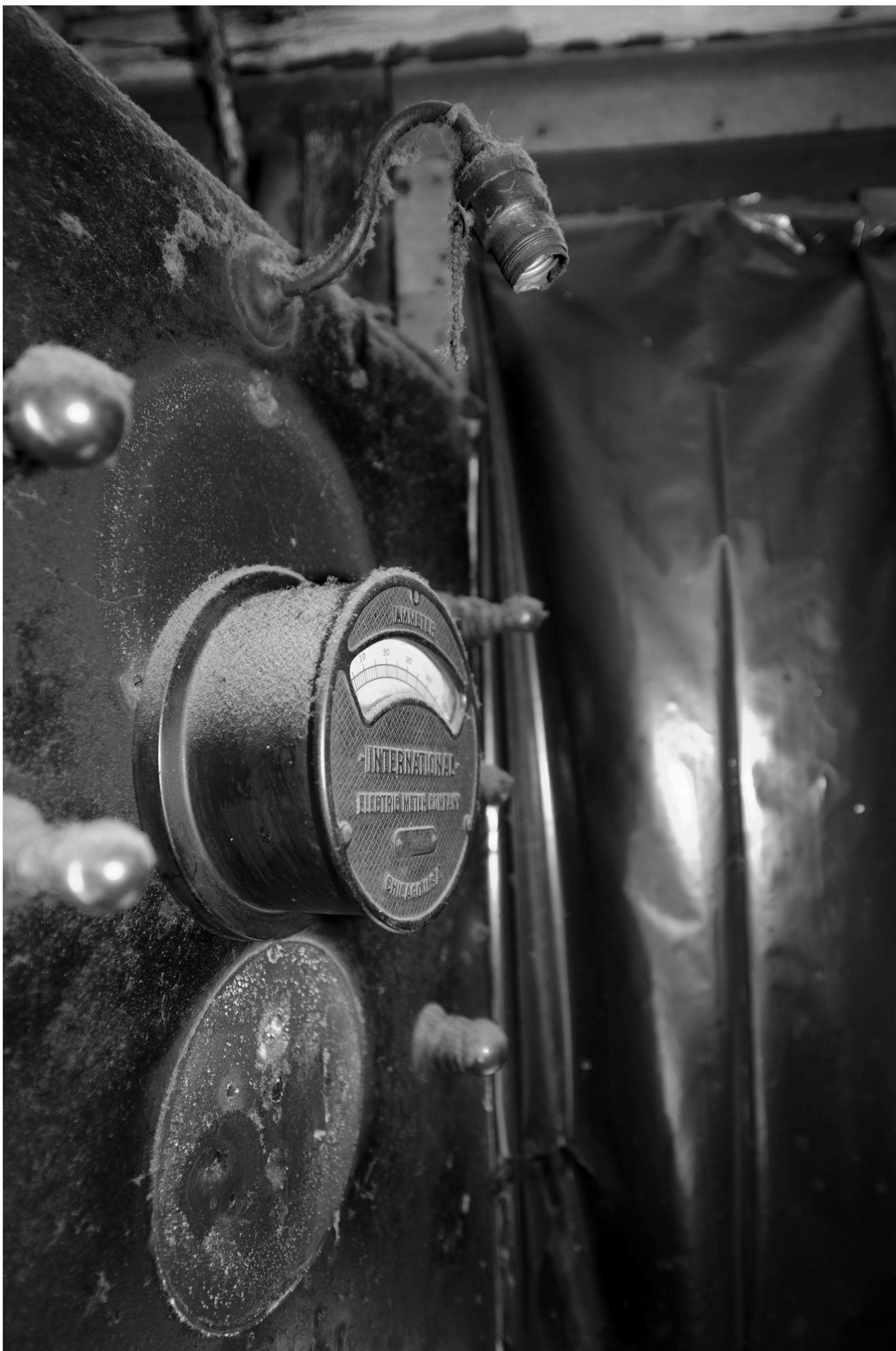
8 of 20 (IL_Cook_16thStreetTower_0008) Detail of power switch board, second floor, looking northeast.
