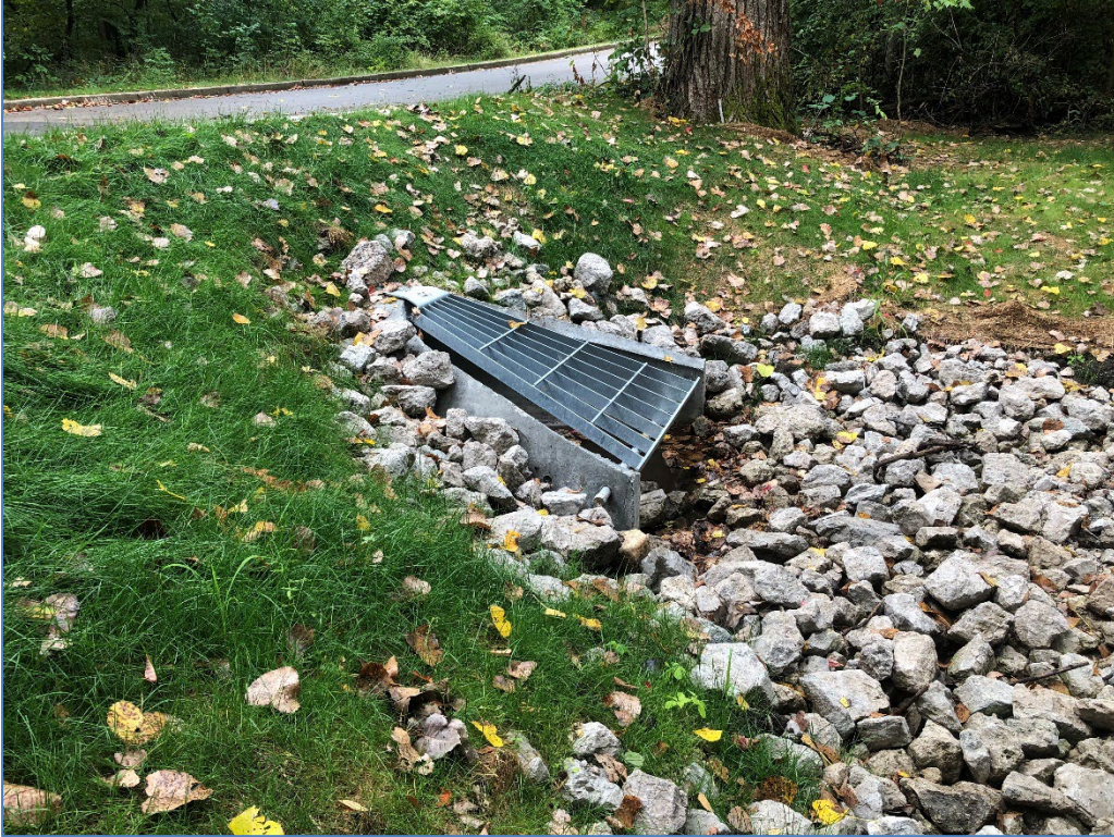
North Side Flared End Section
