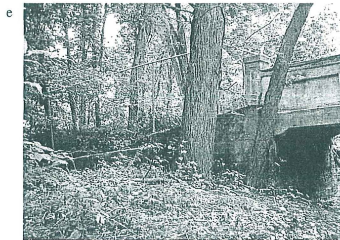
Figure 6. Photographs of bridge: c, view to the north; d, view to southeast; e, view to northeast.
