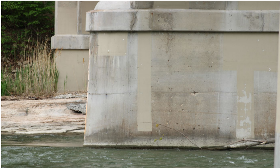
83. Looking North at Patching on S.N. 050-0096 South Profile of Pier #4
