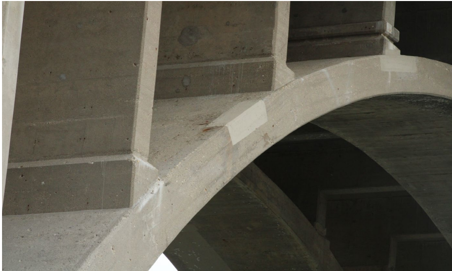
64. Looking South-East at Patching on S.N. 050-0096 West Span #5
