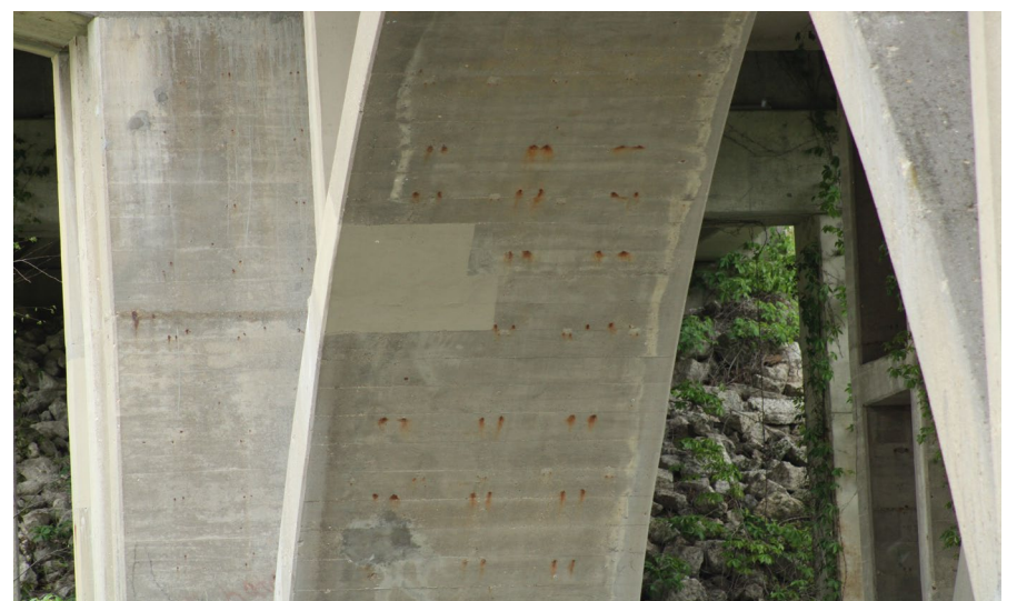
59. Looking South-West at Patching underneath S.N. 050-0096 East Span #6
