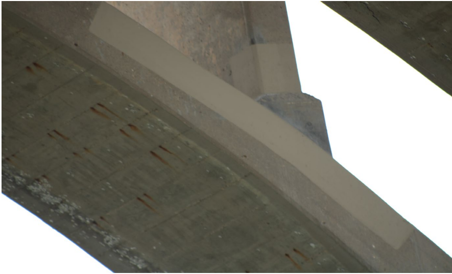
161. Looking North-West at Patching on the East Profile of S.N. 050-0096 West Span #6
