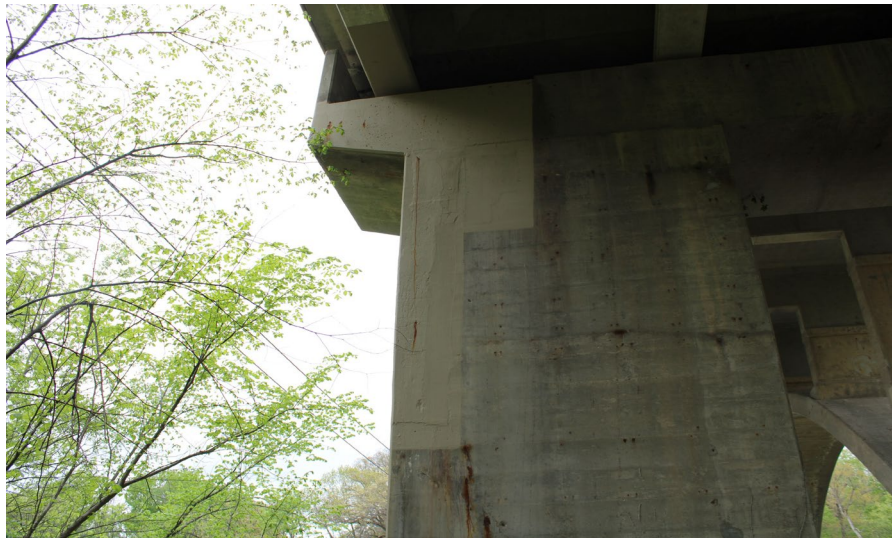
113. Looking North at Patching on S.N. 050-0096 South Profile of Pier #6
