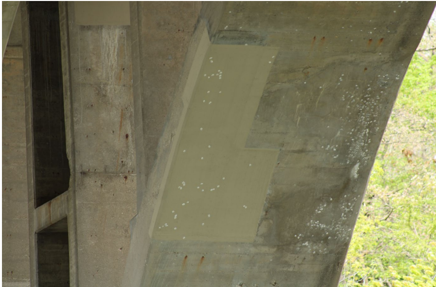
173. Looking North-East at Patching underneath S.N. 050-0096 East Span #5
