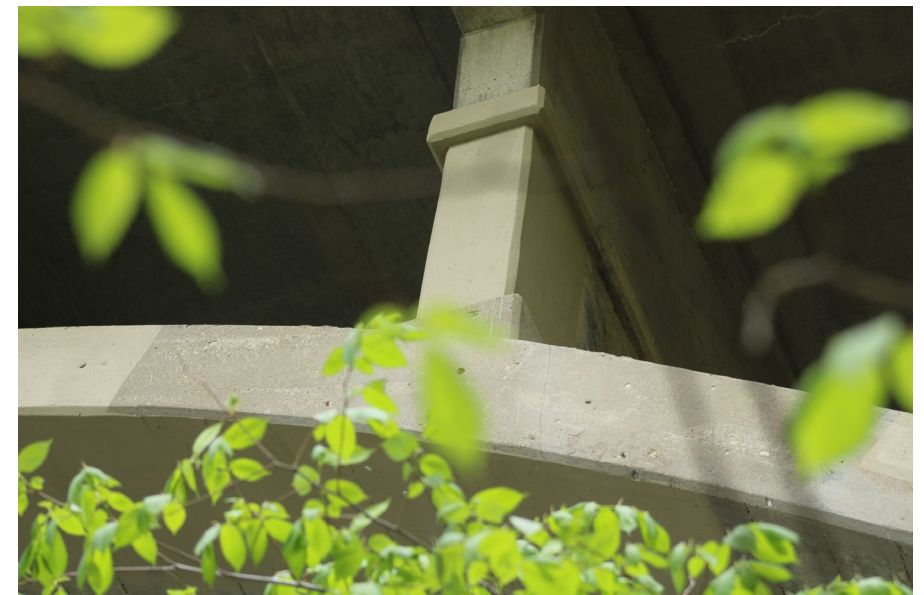
184. Looking East at Patching on S.N. 050-0096 West Profile of West Span #6
