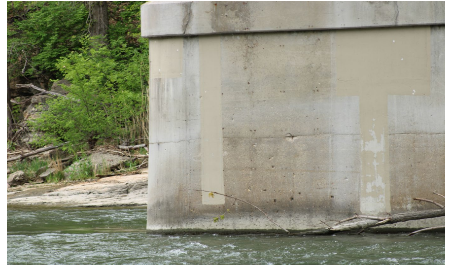
80. Looking North at Patching on S.N. 050-0096 South Profile of Pier #4
