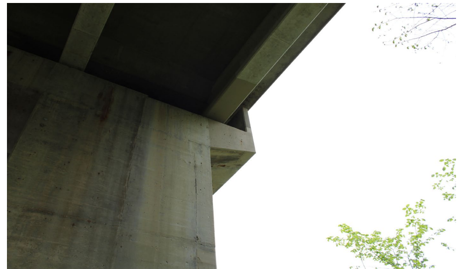
114. Looking North at Patching on S.N. 050-0096 South Profile of Pier #6
