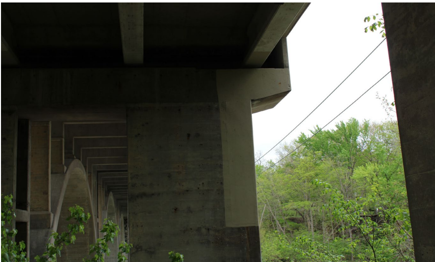
15. Looking South-West at Patching on the North Profile of S.N. 050-0096 West Pier #3
