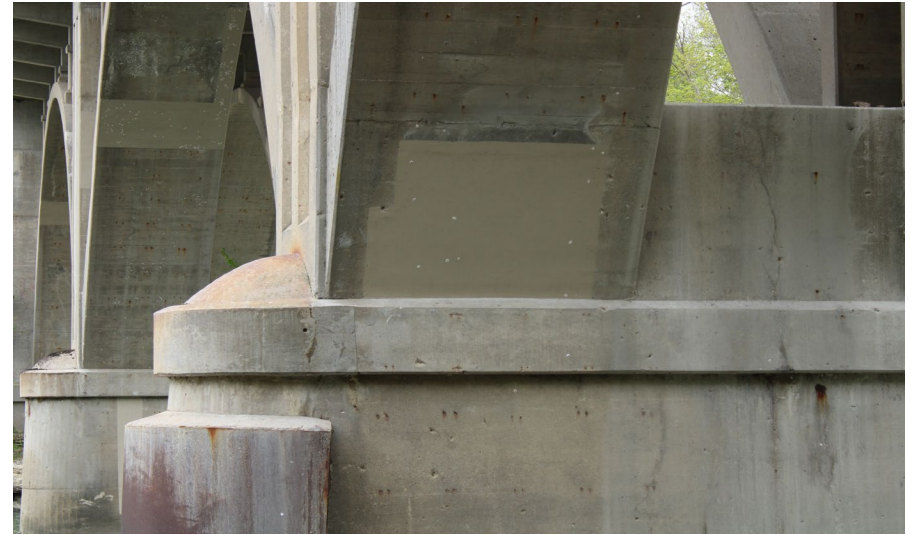
41. Looking South-West at Patching underneath S.N. 050-0096 East Span #4
