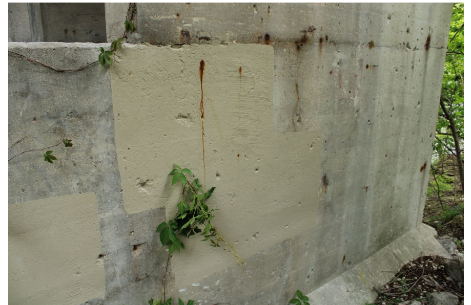
140. Looking North at Patching on S.N. 050-0096 South Profile of Pier #6
