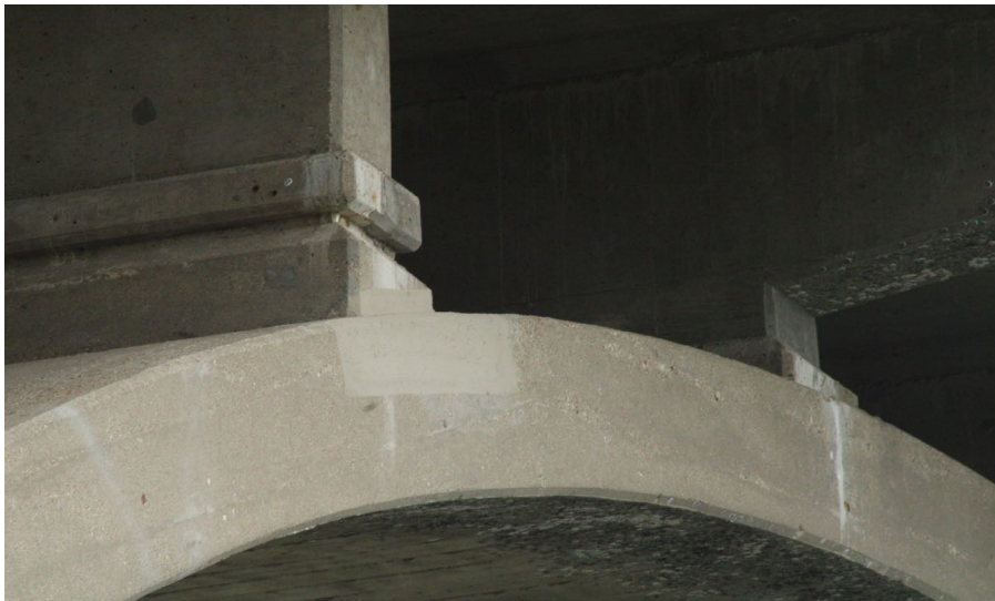
66. Looking South-East at Patching on S.N. 050-0096 West Span #5
