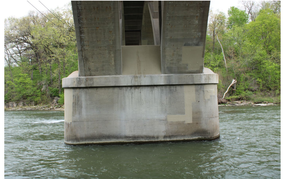
84. Looking North at Patching on S.N. 050-0096 South Profile of Pier #5
