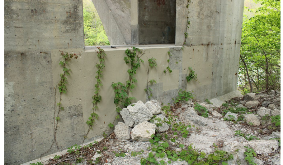
116. Looking North at Patching on S.N. 050-0096 South Profile of Pier #6
