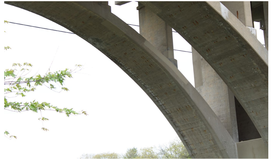
102. Looking West at Patching on S.N. 050-0096 underneath Span #6
