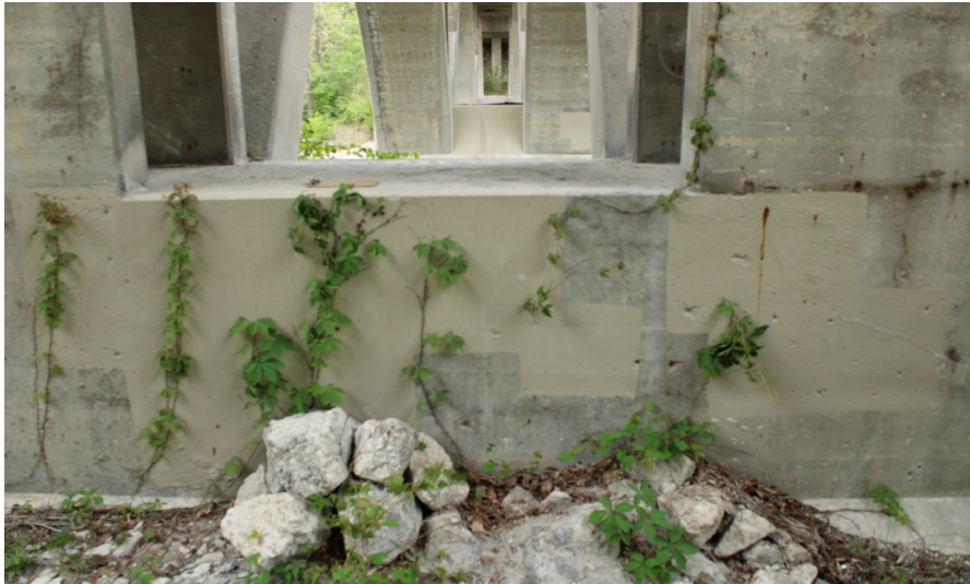
115. Looking North at Patching on S.N. 050-0096 South Profile of Pier #6
