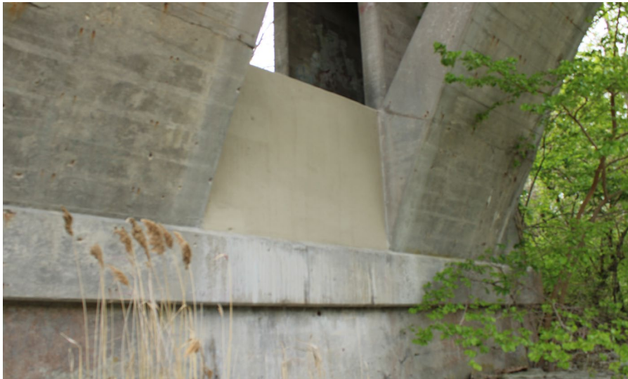
105. Looking South-West at Patching on S.N. 050-0096 North Profile of Pier #6
