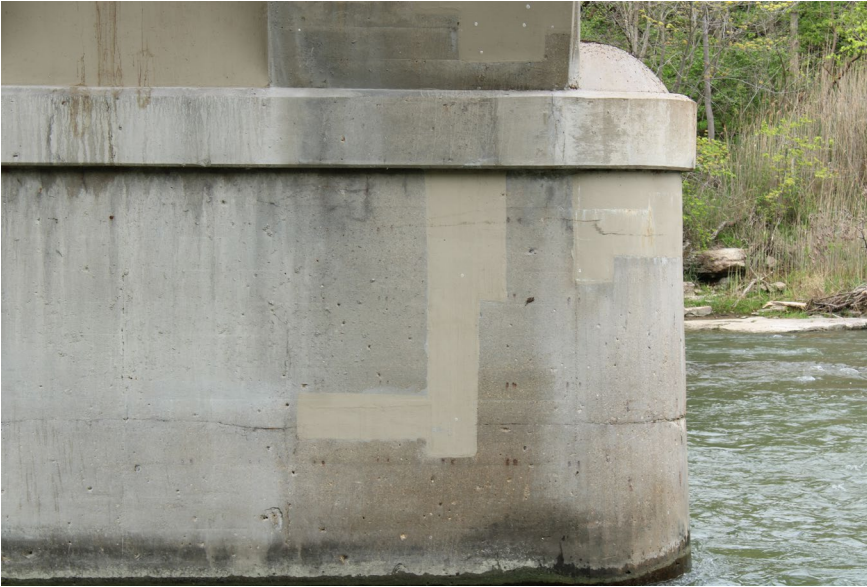
141. Looking North at Patching on S.N. 050-0096 South Profile of Pier #5
