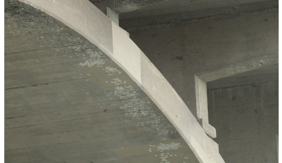
65. Looking South-East at Patching on S.N. 050-0096 West Span #5
