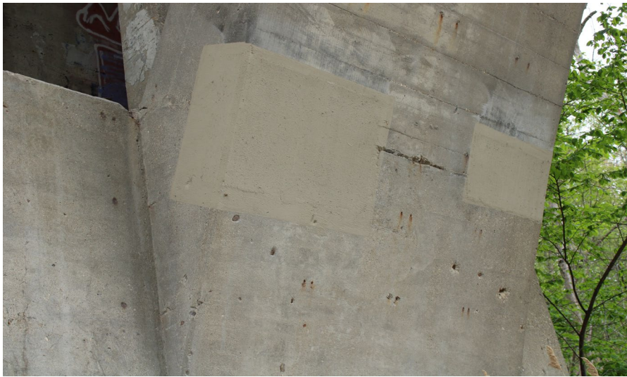
23. Looking North-East at Patching underneath S.N. 050-0096 East Span #4
