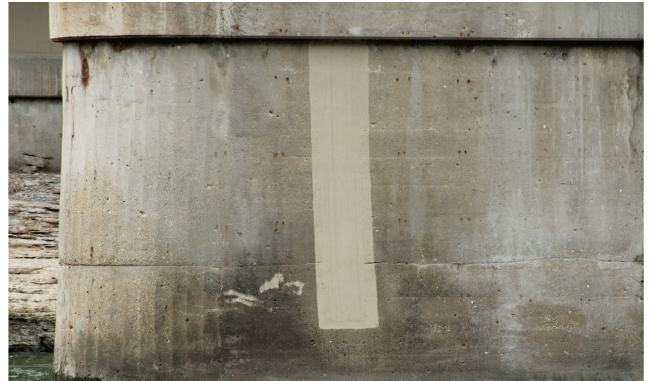
61. Looking South at Patching on S.N. 050-0096 Pier #5
