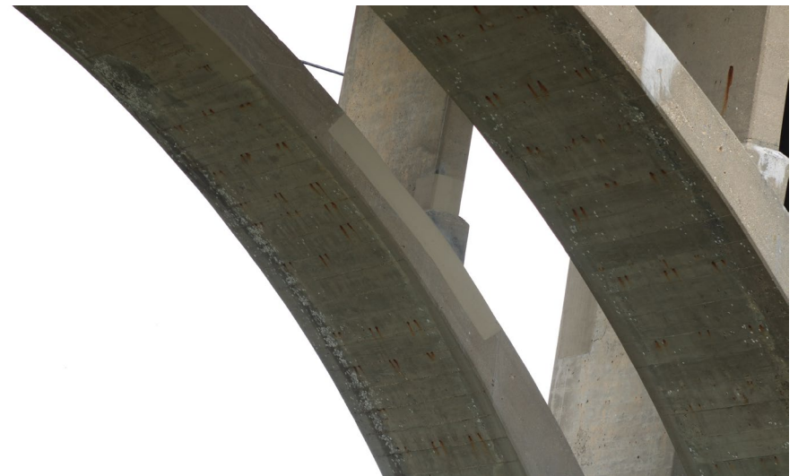
160. Looking North-West at Patching on the East Profile of S.N. 050-0095 West Span #6
