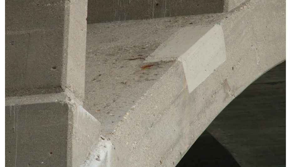
67. Looking South-East at Patching on S.N. 050-0096 West Span #5
