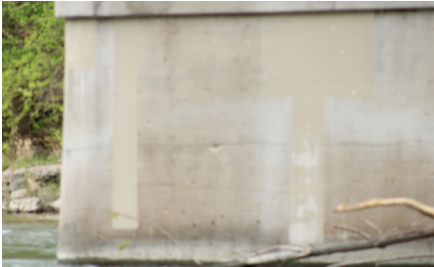
149. Looking North at Patching on S.N. 050-0096 South Profile of Pier #4
