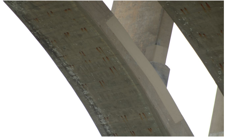
162. Looking North-West at Patching on the East Profile of S.N. 050-0096 West Span #6
