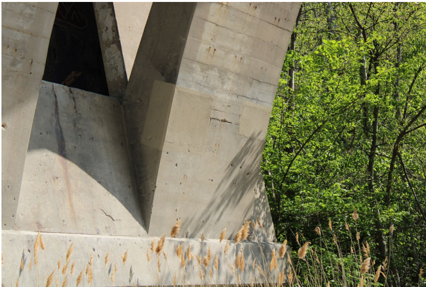
23. Looking North-East at Patching underneath S.N. 050-0096 East Span #4
