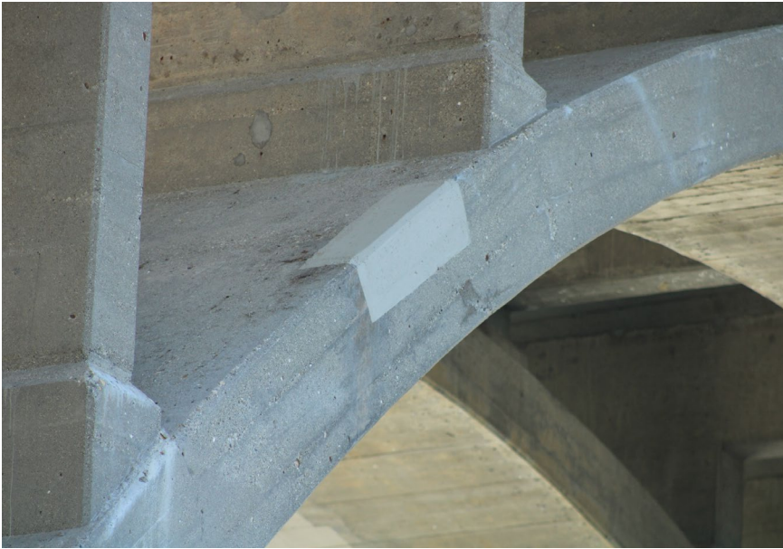
64. Looking South-East at Patching on S.N. 050-0096 West Span #5
