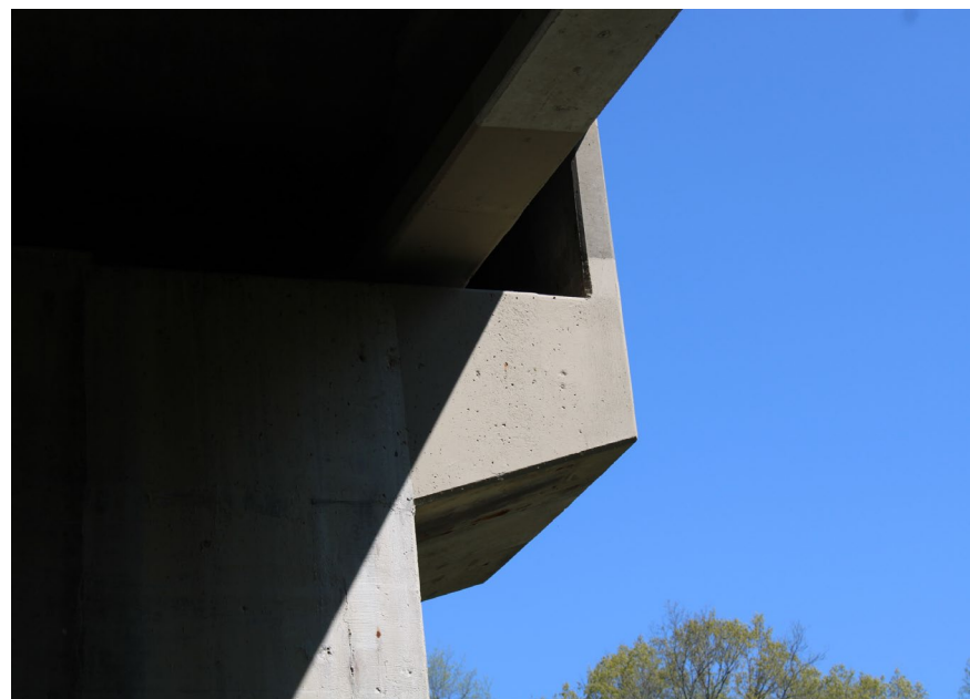
114. Looking North at Patching on S.N. 050-0096 South Profile of Pier #6
