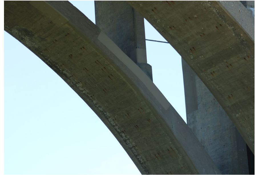
162. Looking North-West at Patching on the East Profile of S.N. 050-0096 West Span #6
