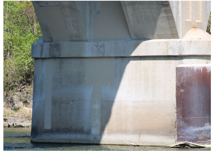
80. Looking North at Patching on S.N. 050-0096 South Profile of Pier #4
