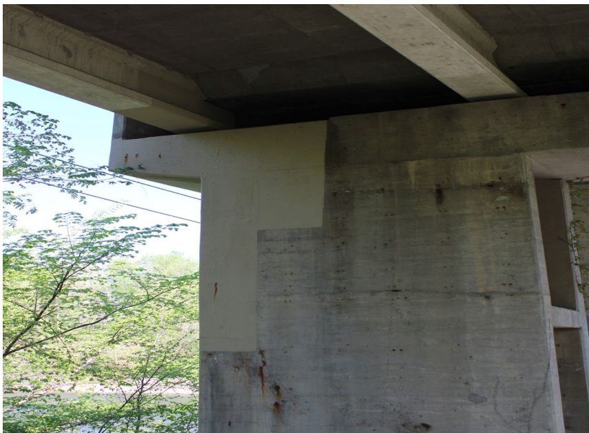
113. Looking North at Patching on S.N. 050-0096 South Profile of Pier #6
