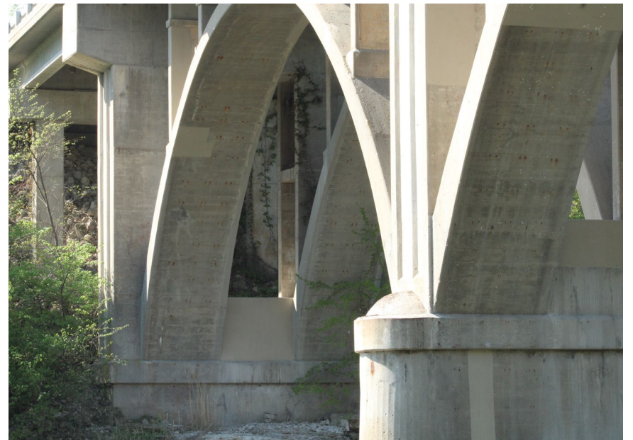
59. Looking South-West at Patching underneath S.N. 050-0096 East Span #6
