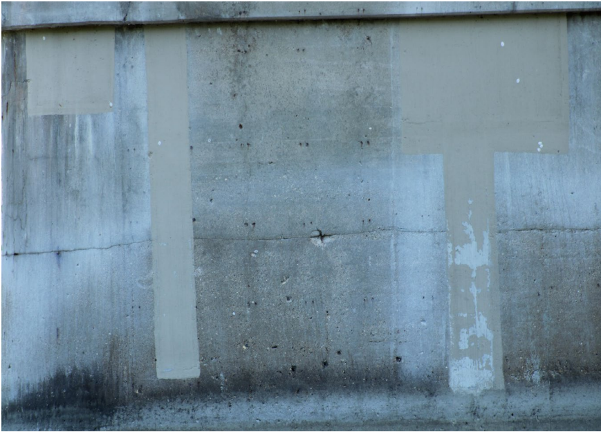
149. Looking North at Patching on S.N. 050-0096 South Profile of Pier #4
