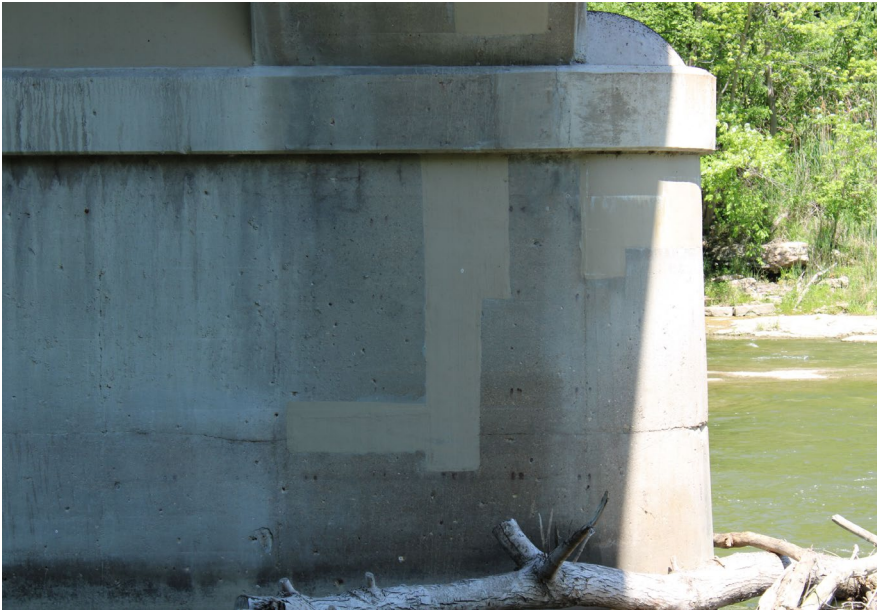
141. Looking North at Patching on S.N. 050-0096 South Profile of Pier #5
