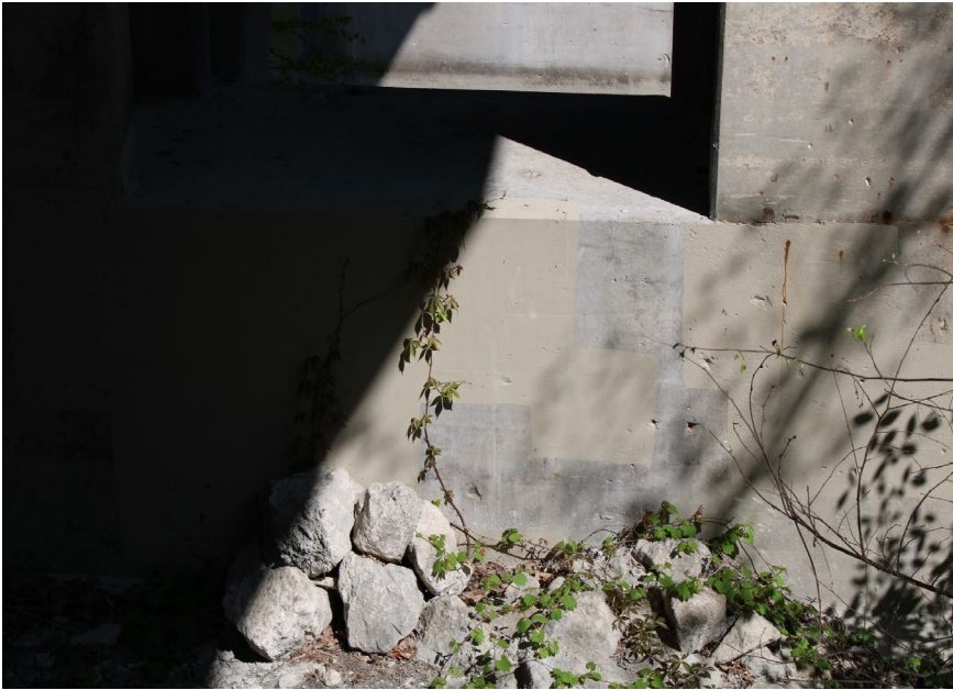
115. Looking North at Patching on S.N. 050-0096 South Profile of Pier #6
