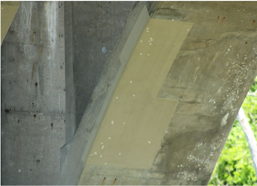
173. Looking North-East at Patching underneath S.N. 050-0096 East Span #5
