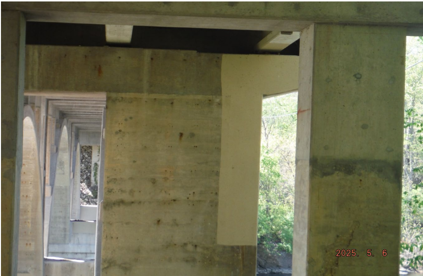
17. Looking South-West at Patching on the North Profile of S.N. 050-0096 West Pier #3
