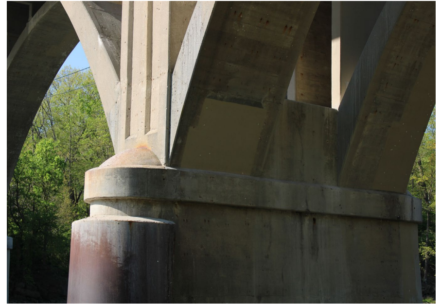
41. Looking South-West at Patching underneath S.N. 050-0096 East Span #4
