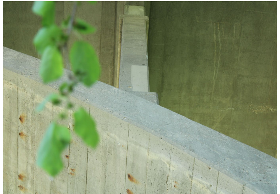
184. Looking East at Patching on S.N. 050-0096 West Profile of West Span #6
