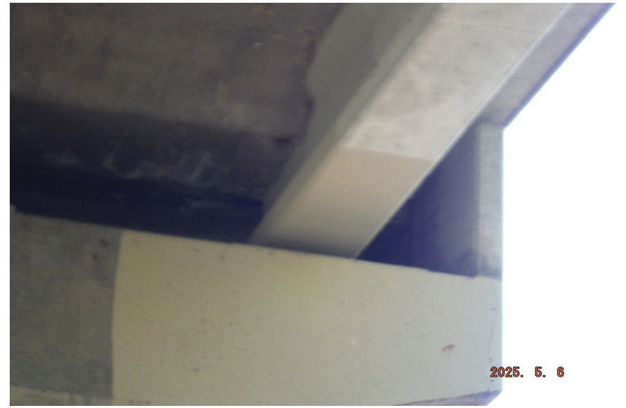
16. Looking South-West at Patching along the beams on the North Profile of S.N. 050-0096 West Pier #3
