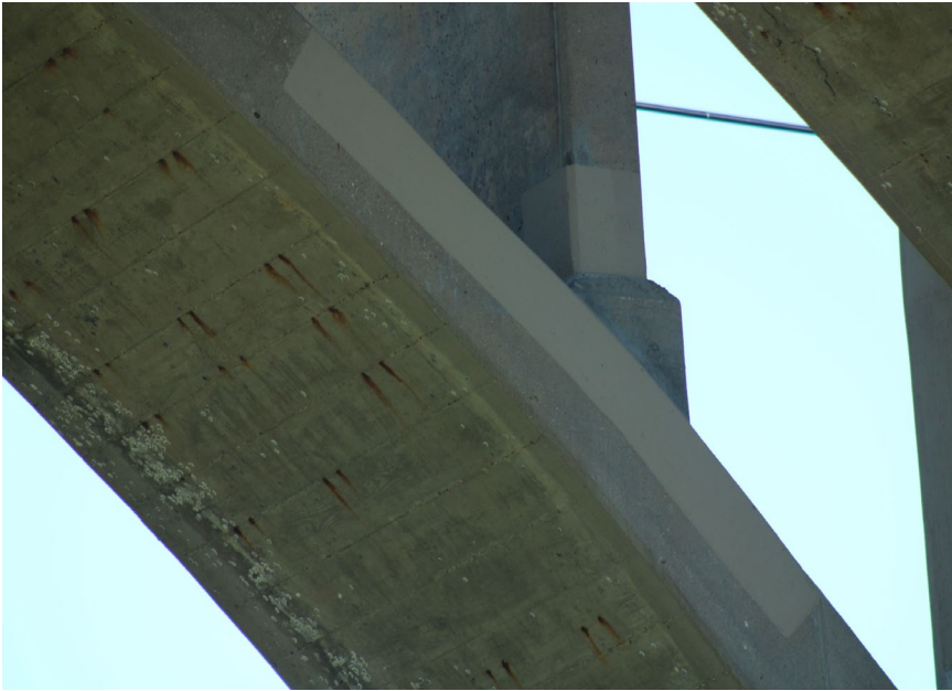
161. Looking North-West at Patching on the East Profile of S.N. 050-0096 West Span #6
