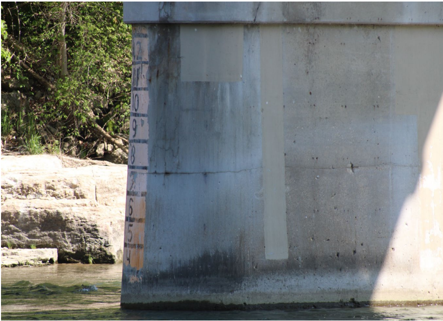
83. Looking North at Patching on S.N. 050-0096 South Profile of Pier #4
