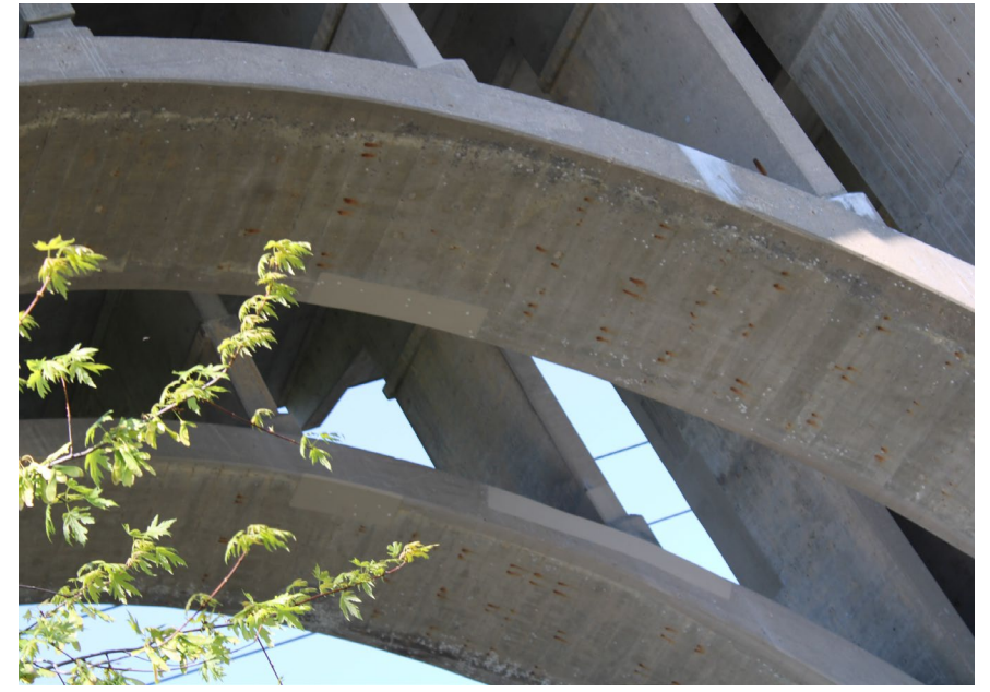
102. Looking West at Patching on S.N. 050-0096 underneath Span #6
