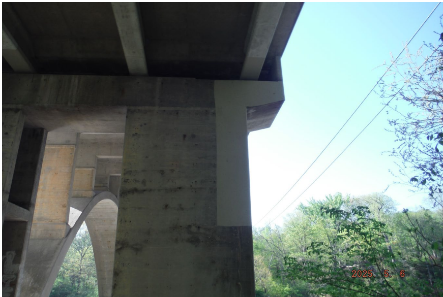
15. Looking South-West at Patching on the North Profile of S.N. 050-0096 West Pier #3
