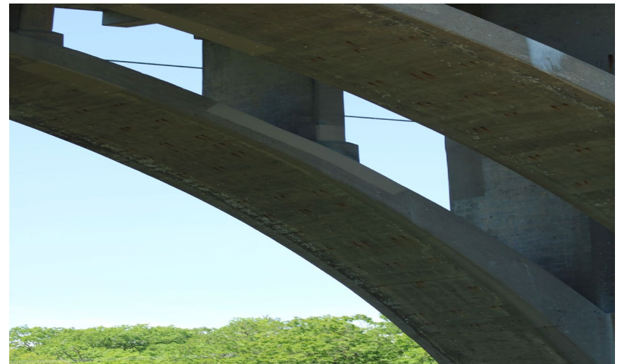
160. Looking North-West at Patching on the East Profile of S.N. 050-0095 West Span #6
