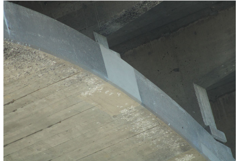
65. Looking South-East at Patching on S.N. 050-0096 West Span #5
