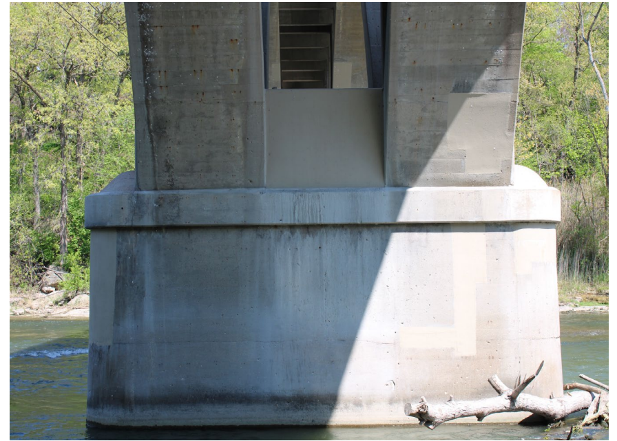
84. Looking North at Patching on S.N. 050-0096 South Profile of Pier #5
