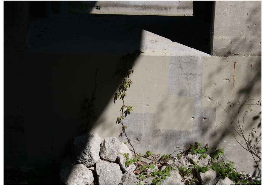
116. Looking North at Patching on S.N. 050-0096 South Profile of Pier #6
