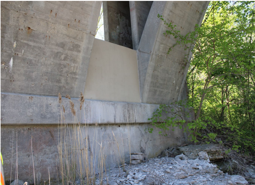
105. Looking South-West at Patching on S.N. 050-0096 North Profile of Pier #6
