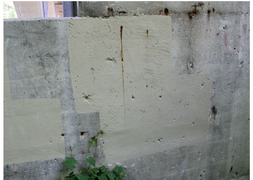
140. Looking North at Patching on S.N. 050-0096 South Profile of Pier #6
