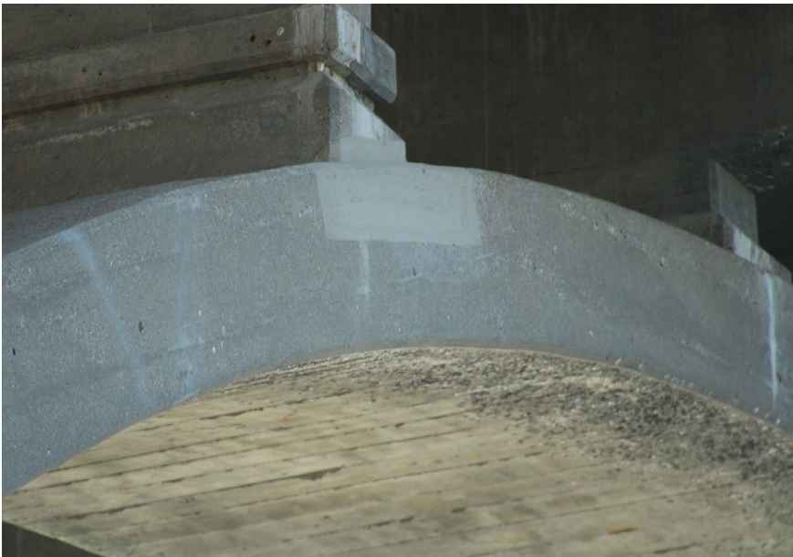
66. Looking South-East at Patching on S.N. 050-0096 West Span #5
