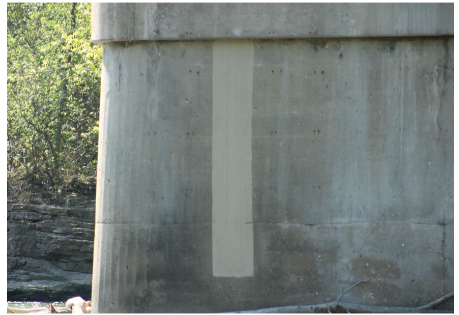
61. Looking South at Patching on S.N. 050-0096 Pier #5
