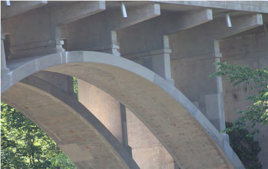
177. Looking East at Patching on the West Profile of S.N. 050-0096 West Span #6
