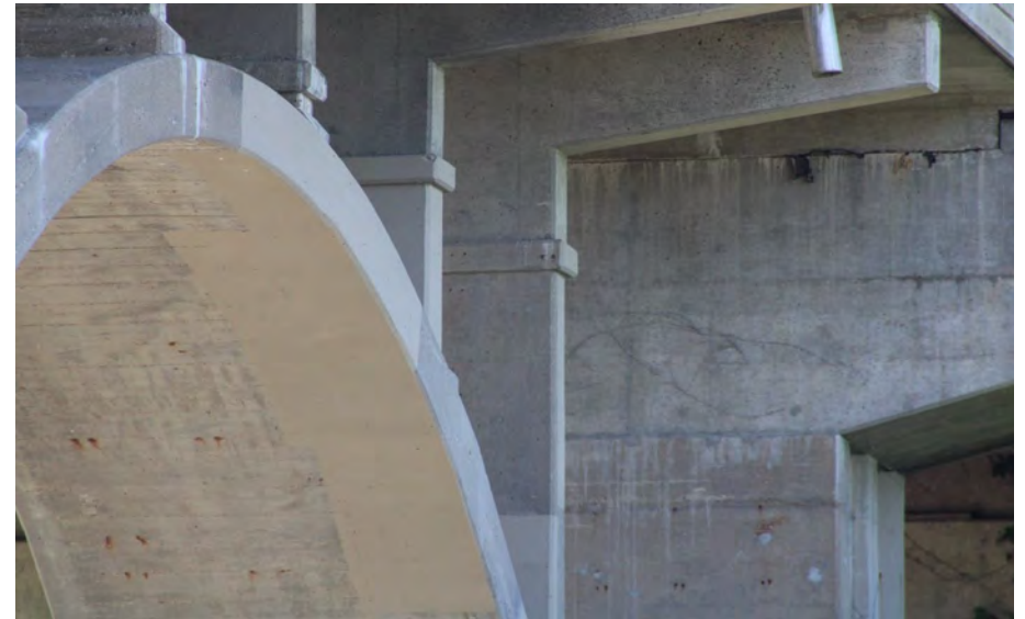
174. Looking South-East at Patching on the West Profile of S.N. 050-0096 West Span #6
