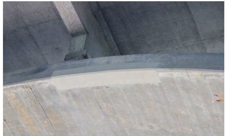
180. Looking Directly Up at Patching on S.N. 050-0096 East Span #6
