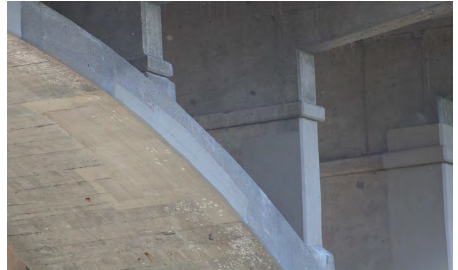
110. Looking South-East at Patching on the West Profile of S.N. 050-0096 West Span #5
