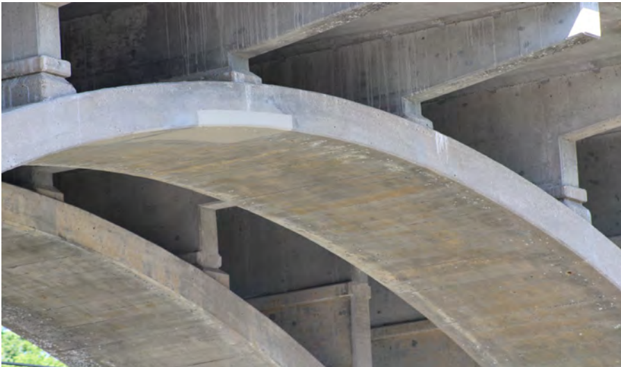
199. Looking North-West at Patching on the West Profile of S.N. 050-0096 East Span #6
