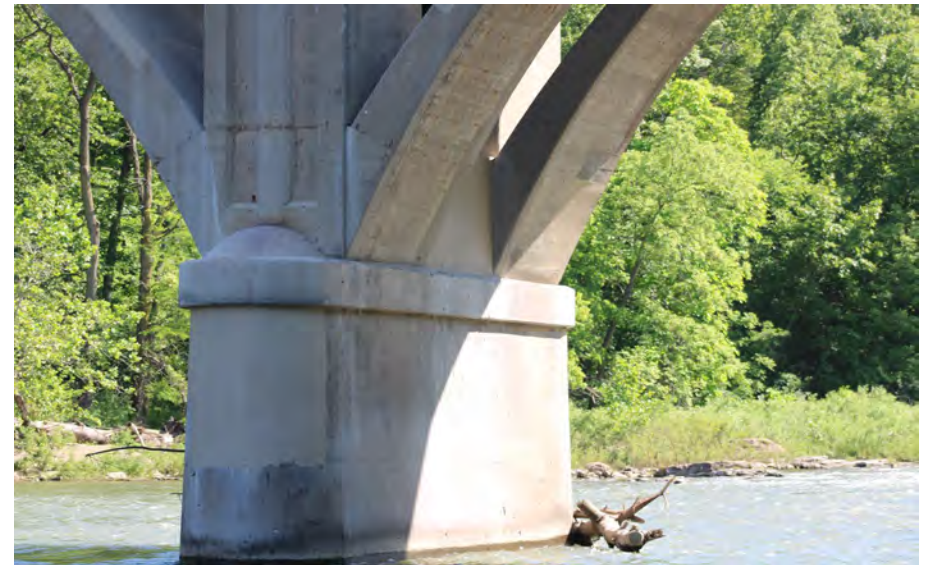
144. Looking East at Patching on the West Profile of S.N. 050-0096 Pier #5
