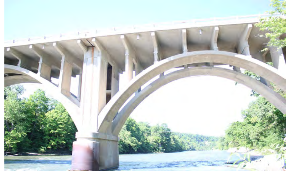
6. Looking West at Patching on the East Profile of S.N. 050-0096
