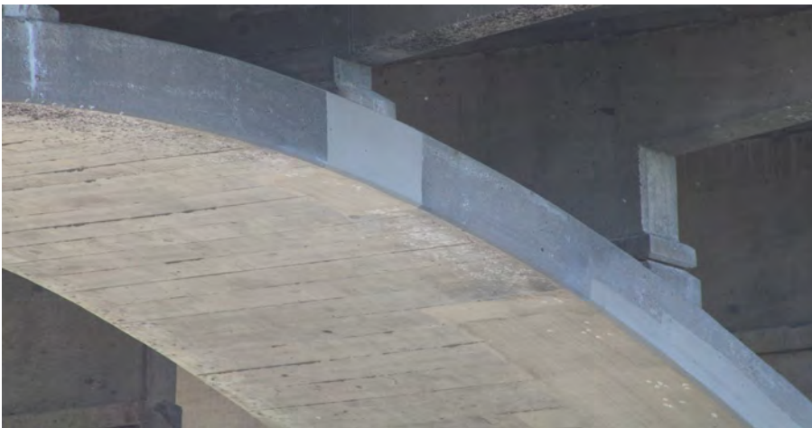
119. Looking South-East at Patching on the West Profile of S.N. 050-0096 West Span #5
