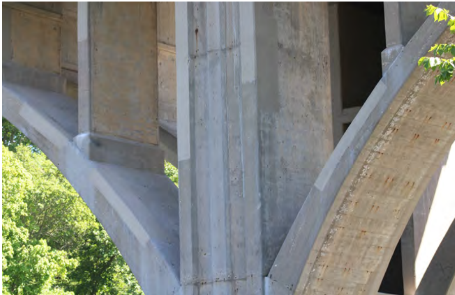
147. Looking East at Patching on the West Profile of S.N. 050-0096 Pier #5
