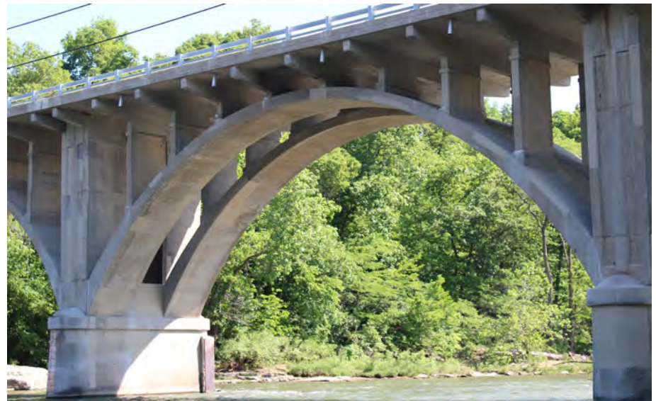
100. Looking North-East at Patching on the West Profile of S.N. 050-0096 Span #5
