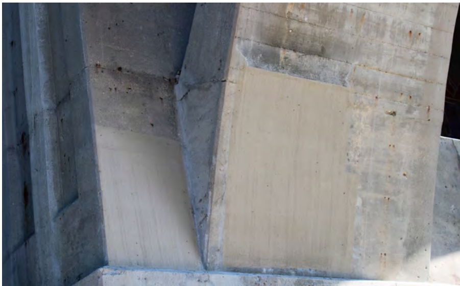
31. Looking North-East at Patching on the South Profile of S.N. 050-0096 West Pier #3
