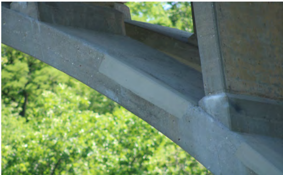
115. Looking North-East at Patching on the West Profile of S.N. 050-0096 West Span #5
