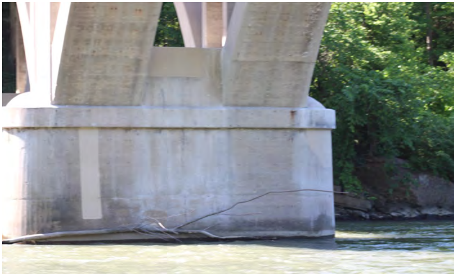
127. Looking South-West at Patching on the North Profile of S.N. 050-0096 Pier #5
