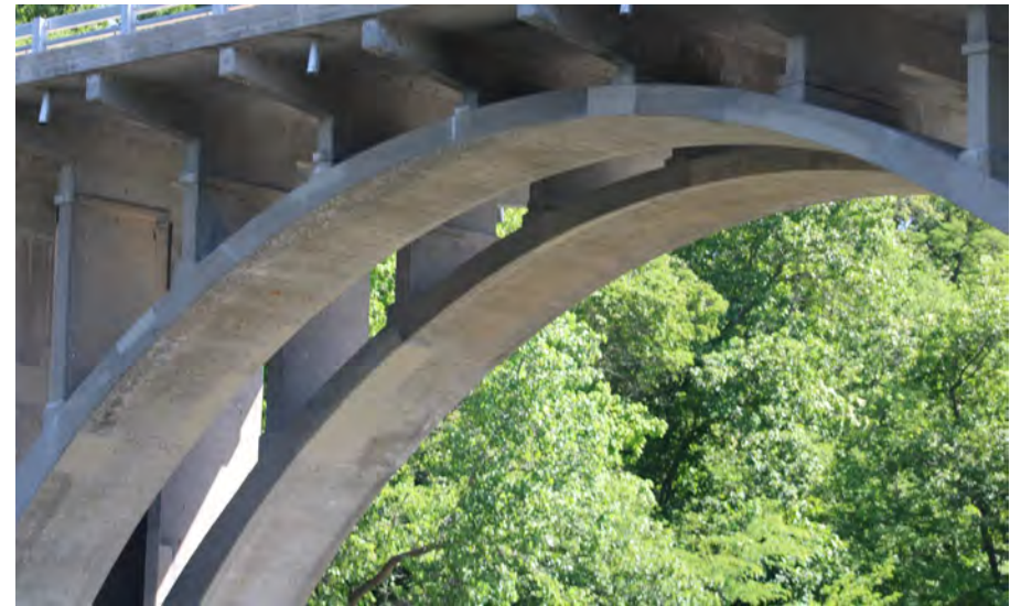
98. Looking North-East at Patching on the West Profile of S.N. 050-0096 Span #5
