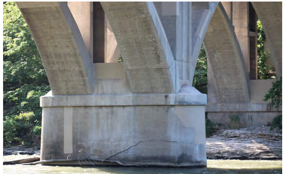
152. Looking South-East at Patching on the North Profile of S.N. 050-0096 Pier #5
