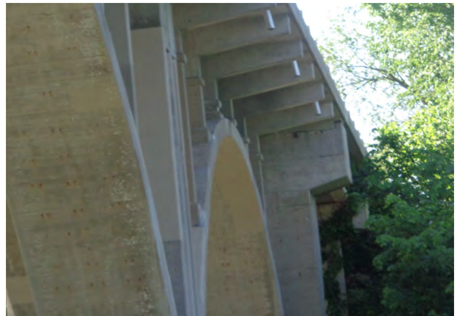
148. Looking South at Patching on the West Profile of S.N. 050-0096 Pier #5
