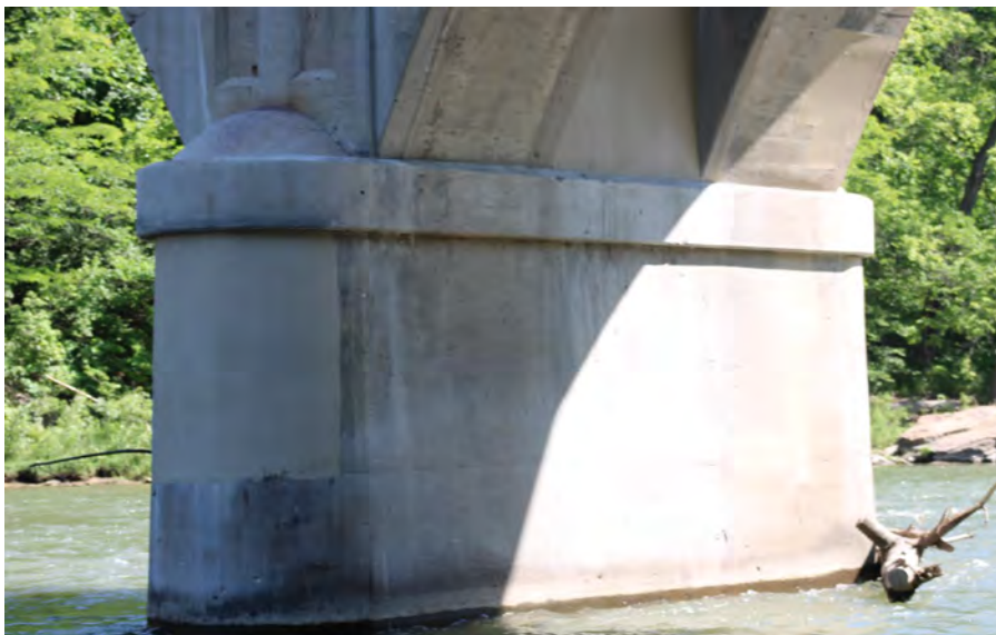
151. Looking East at Patching on the West Profile of S.N. 050-0096 Pier #5
