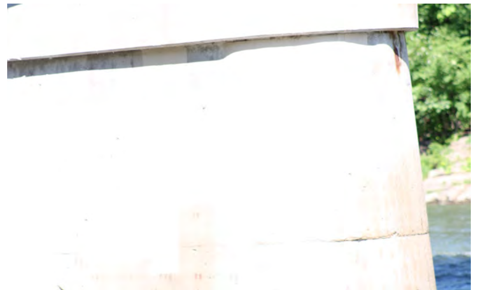
140. Looking North-West at Patching on the East Profile of S.N. 050-0096 Pier #5
