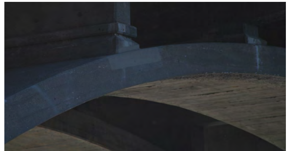
116. Looking South-East at Patching on the West Profile of S.N. 050-0096 West Span #5
