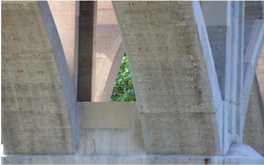
157. Looking South-East at Patching on the North Profile of S.N. 050-0096 Pier #5
