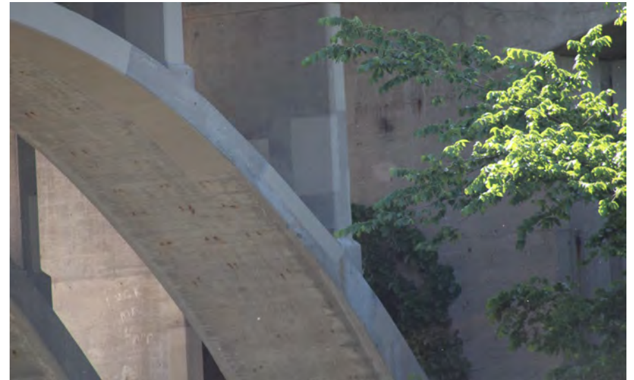
178. Looking South-East at Patching on the West Profile of S.N. 050-0096 West Span #6
