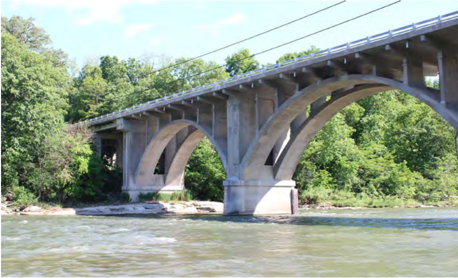
9. Looking North-East at Patching on the West Profile of S.N. 050-0096
