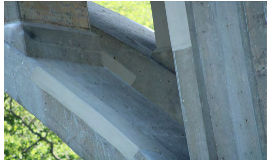
112. Looking North-East at Patching on the West Profile of S.N. 050-0096 West Span #5
