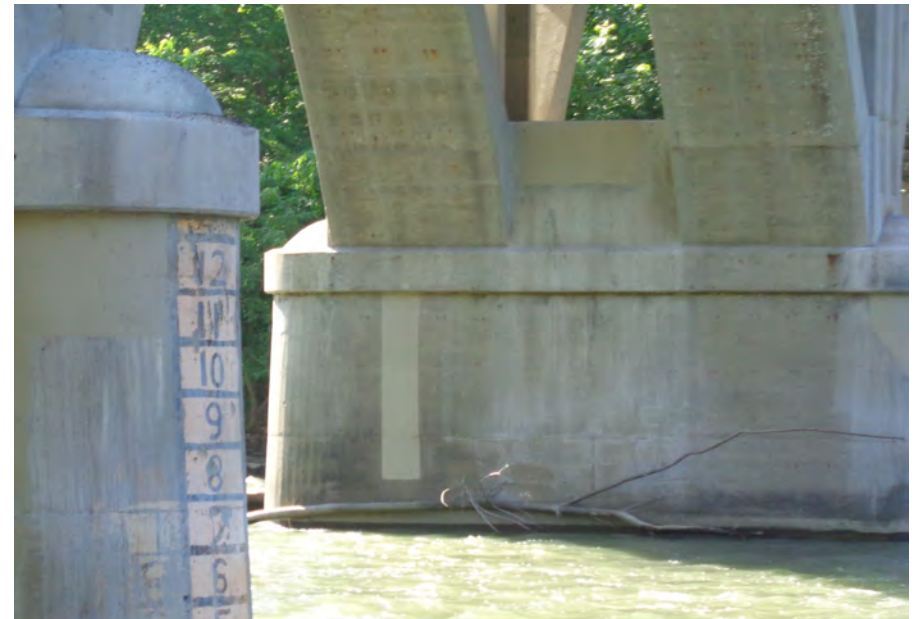
128. Looking South-East at Patching on the North Profile of S.N. 050-0096 Pier #5
