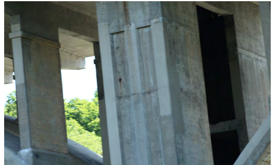
146. Looking East at Patching on the West Profile of S.N. 050-0096 Pier #5
