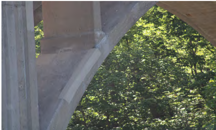
179. Looking South-East at Patching on the West Profile of S.N. 050-0096 West Span #6
