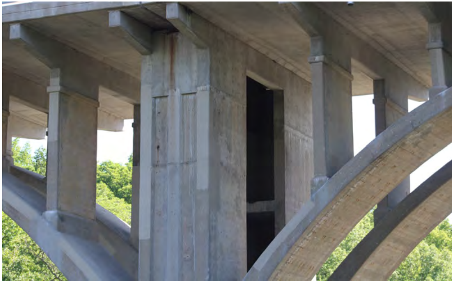
145. Looking East at Patching on the West Profile of S.N. 050-0096 Pier #5
