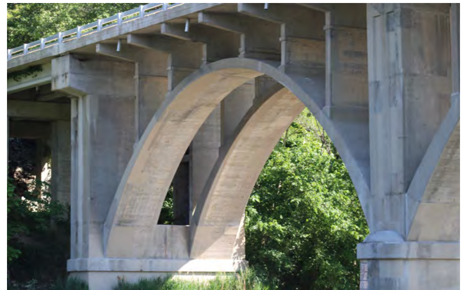
76. Looking North-East at Patching on & under S.N. 050-0096 Span #4
