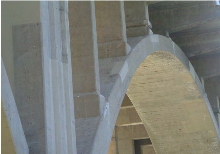
109. Looking South at Patching on the West Profile of S.N. 050-0096 West Span #5
