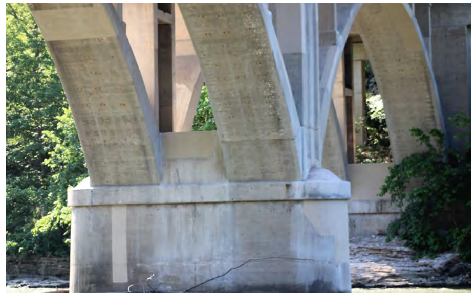
156. Looking South-East at Patching on the North Profile of S.N. 050-0096 Pier #5
