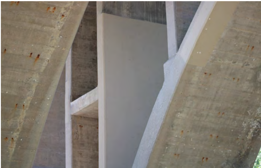
79. Looking South-West at Patching on the North Profile of S.N. 050-0096 Pier #4
