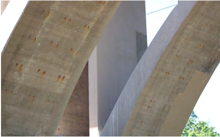
89. Looking South-West at Patching on the North Profile of S.N. 050-0096 Pier #4
