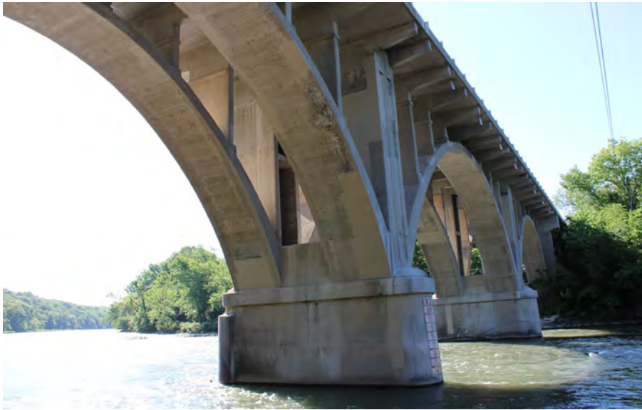
77. Looking South-East at Patching on the North Profile of S.N. 050-0096 Pier #4
