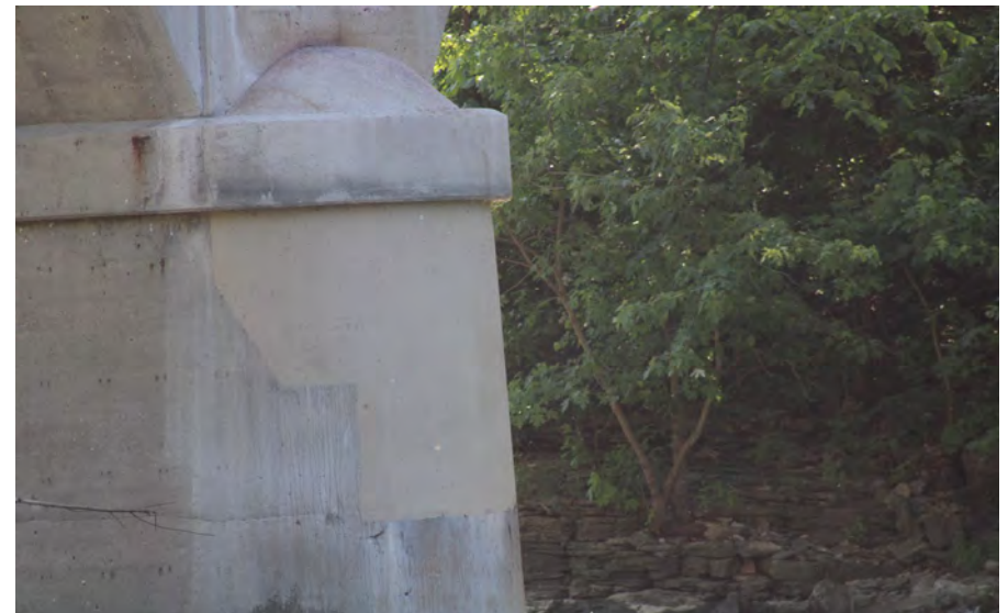
132. Looking South at Patching on the West Profile of S.N. 050-0096 Pier #5
