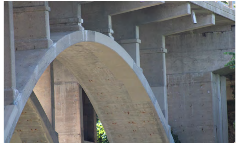
176. Looking South-East at Patching on the West Profile of S.N. 050-0096 West Span #6
