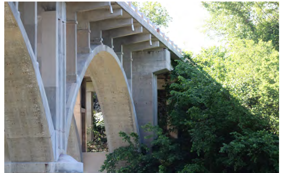
168. Looking South at Patching on the West Profile of S.N. 050-0096 West Span #6
