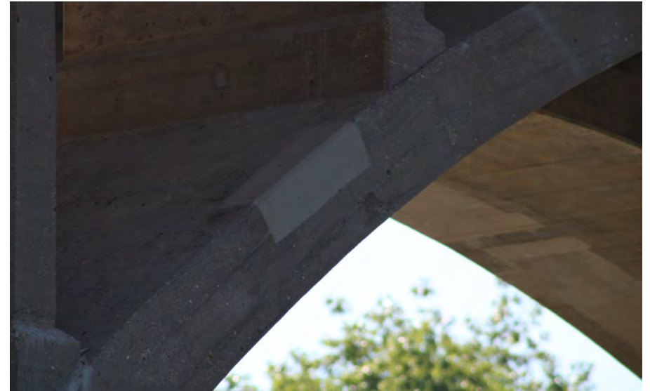
118. Looking South-East at Patching on the West Profile of S.N. 050-0096 West Span #5
