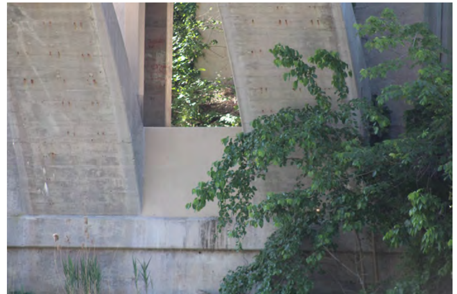
204. Looking South-East at Patching on the North Profile of S.N. 050-0096 Pier #6
