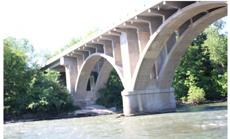
134. Looking South-West at Patching on the East Profile of S.N. 050-0096 Pier #5
