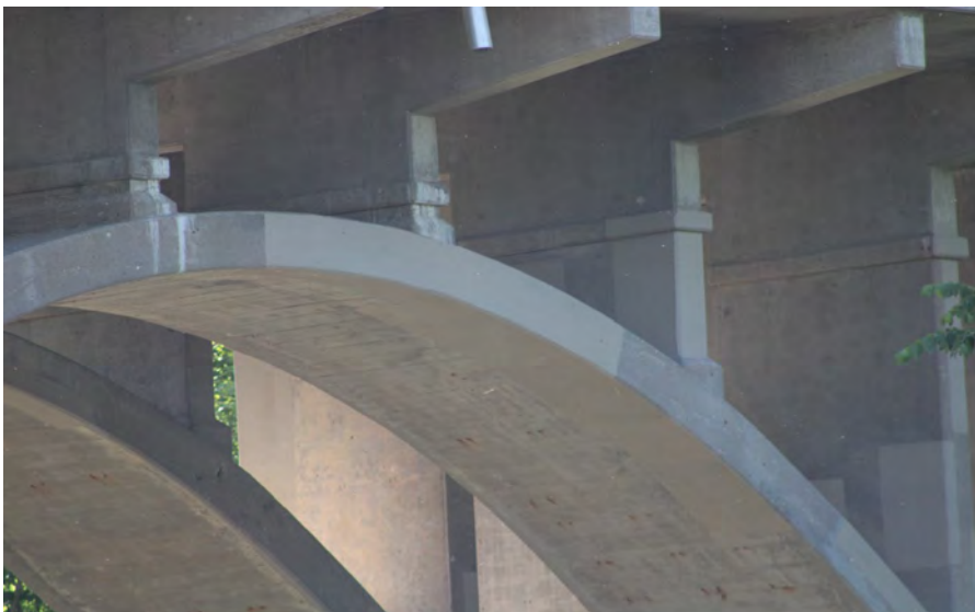
175. Looking East at Patching on the West Profile of S.N. 050-0096 West Span #6
