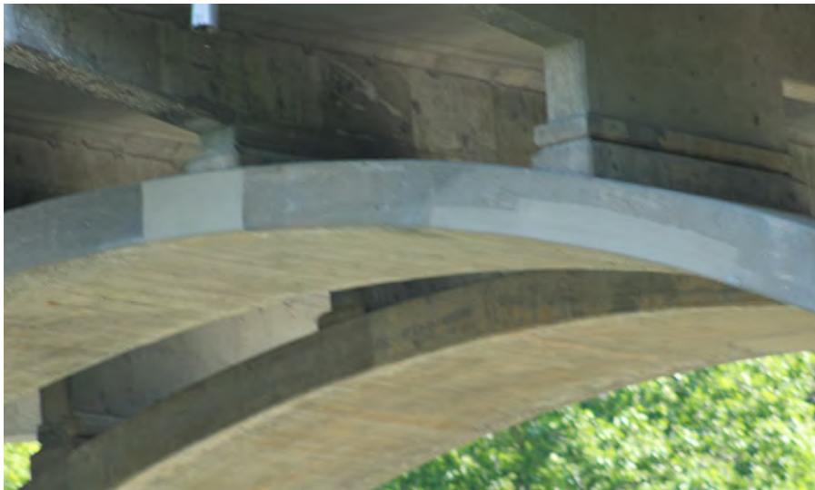
111. Looking North-East at Patching on the West Profile of S.N. 050-0096 West Span #5
