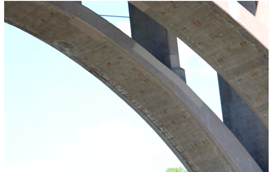
190. Looking North-West at Patching on the East Profile of S.N. 050-0096 West Span #6
