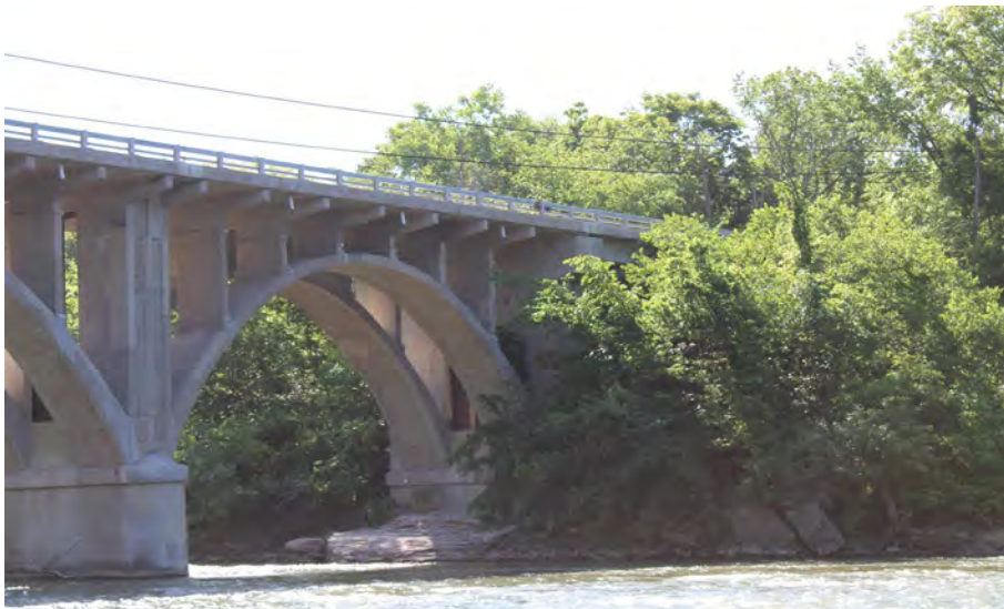
171. Looking South-East at Patching on the West Profile of S.N. 050-0096 West Span #6
