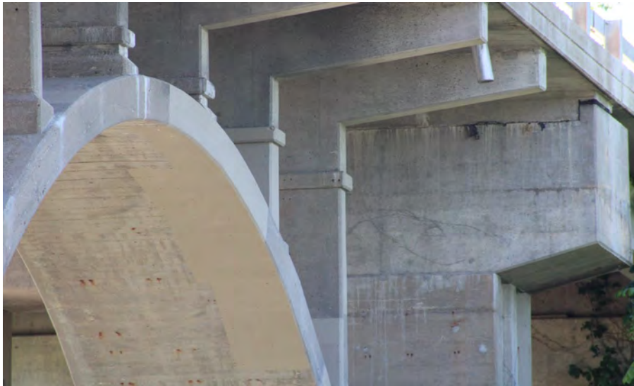
173. Looking South-East at Patching on the West Profile of S.N. 050-0096 West Span #6
