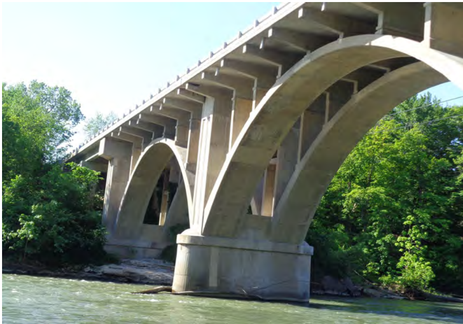
133. Looking South-West at Patching on the East Profile of S.N. 050-0096 Pier #5
