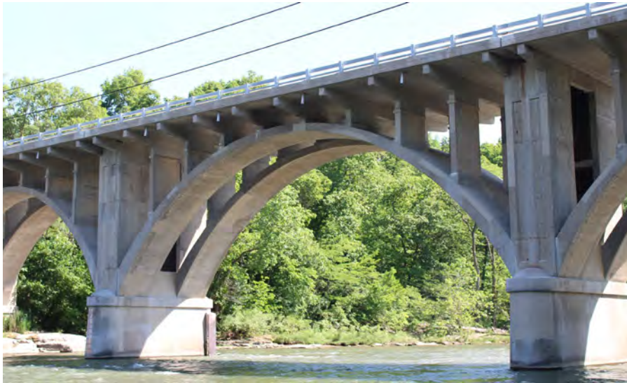
97. Looking North-East at Patching on the West Profile of S.N. 050-0096 Span #5
