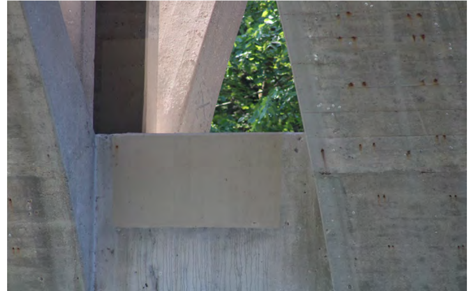
158. Looking South-East at Patching on the North Profile of S.N. 050-0096 Pier #5
