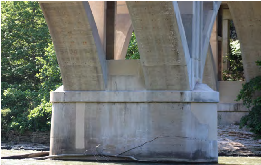
153. Looking South-East at Patching on the North Profile of S.N. 050-0096 Pier #5
