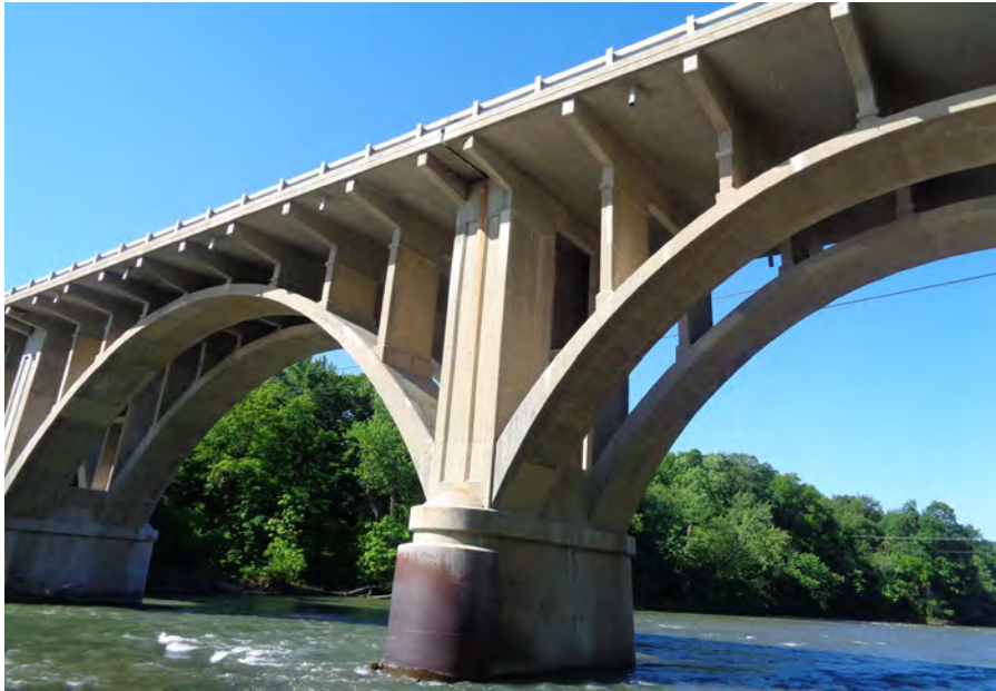
85. Looking South-West at Patching on the East Profile of S.N. 050-0096 Pier #4
