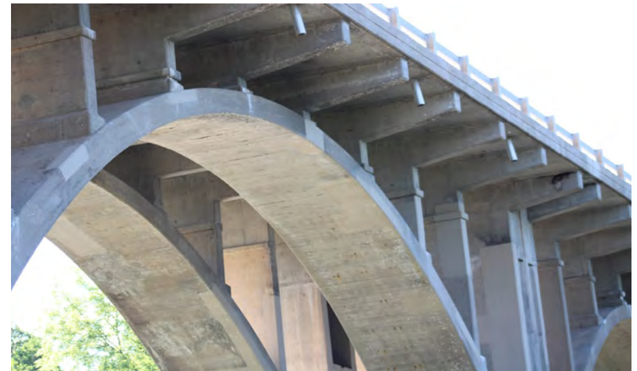
120. Looking South-East at Patching on the West Profile of S.N. 050-0096 West Span #5
