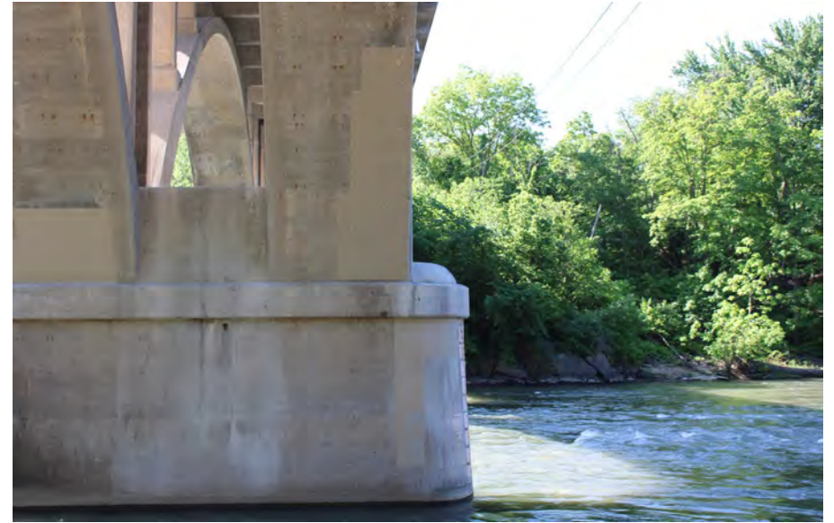
78. Looking South-West at Patching on the North Profile of S.N. 050-0096 Pier #4
