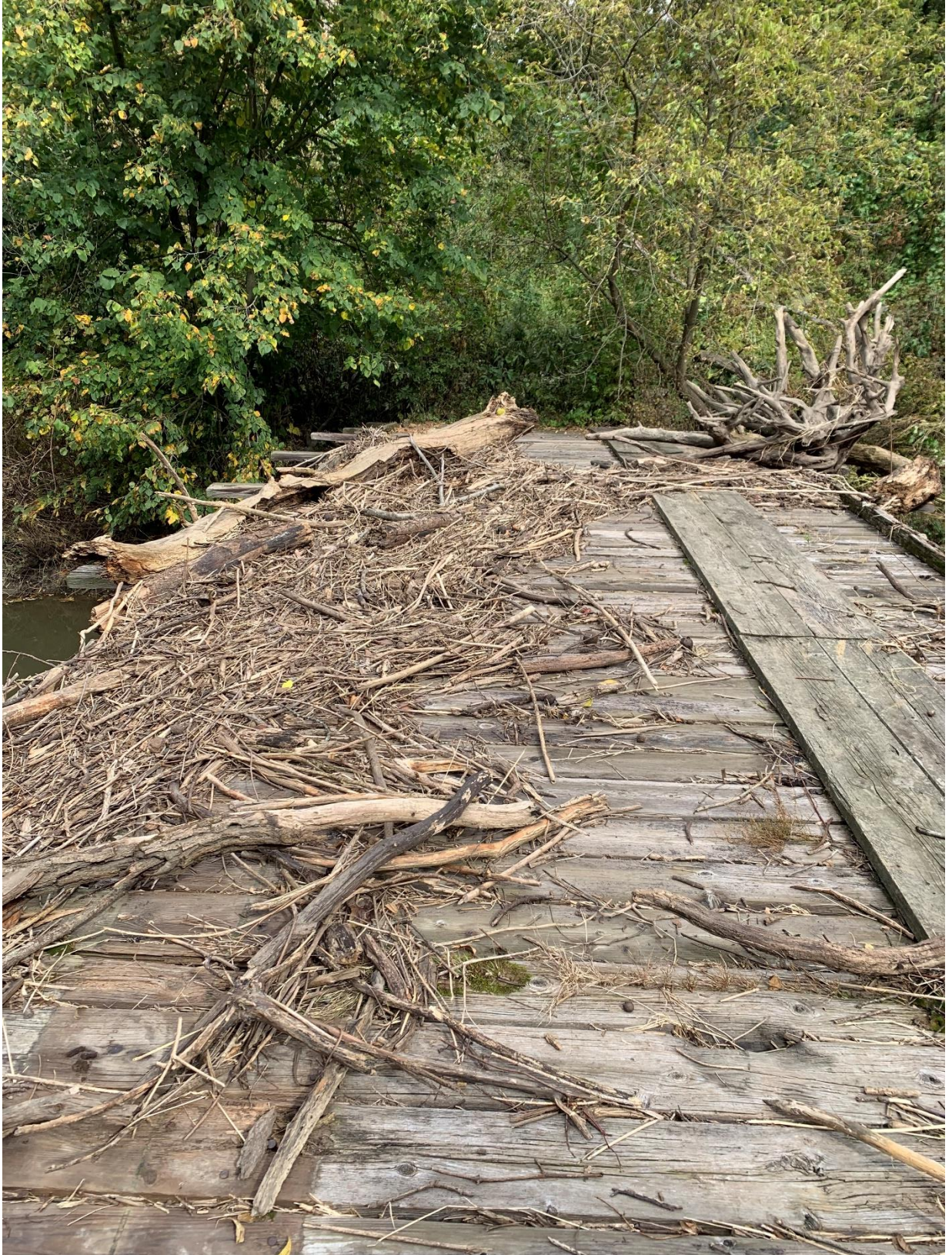
Flood debris on bridge
