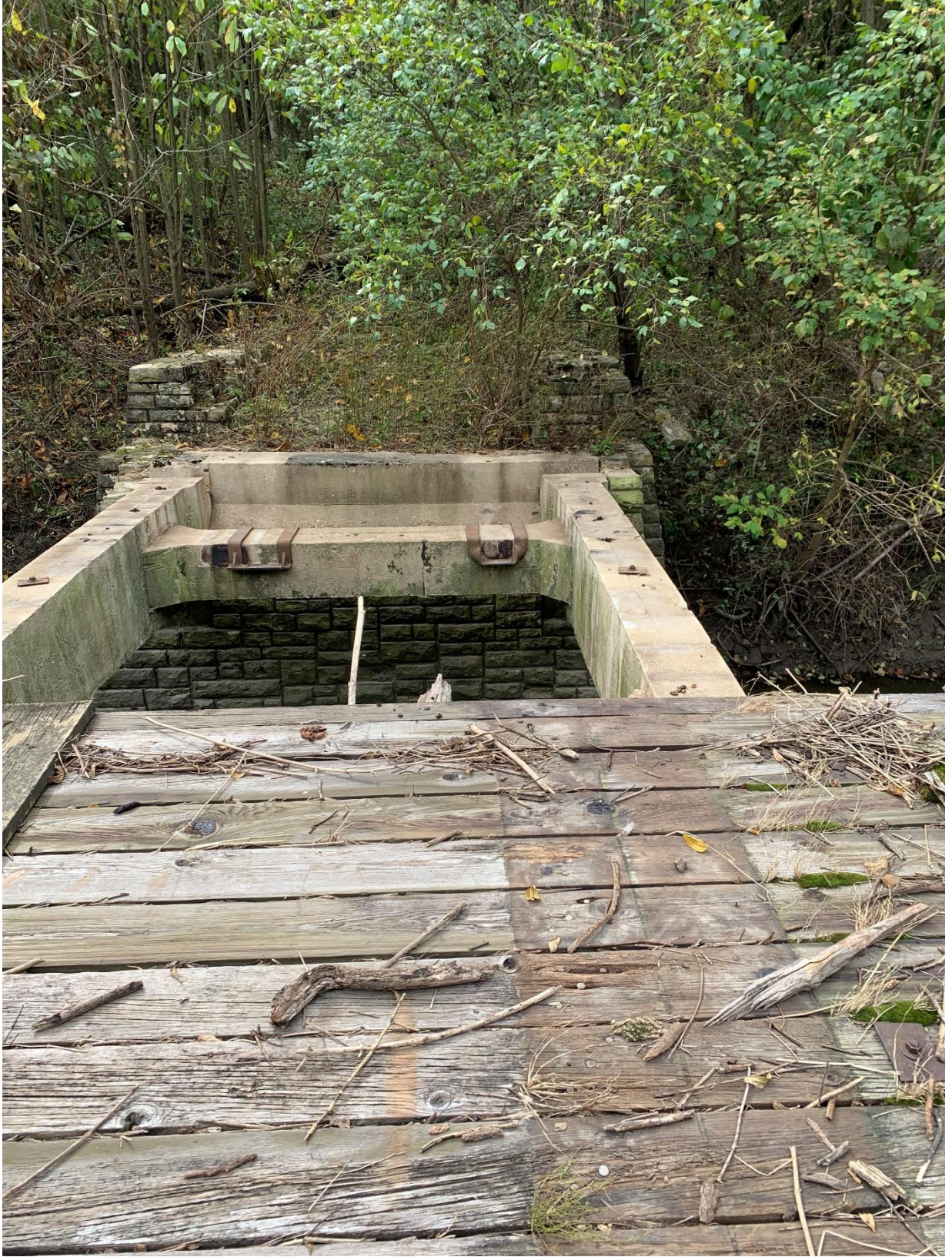
Lost planks due to flood damage.
