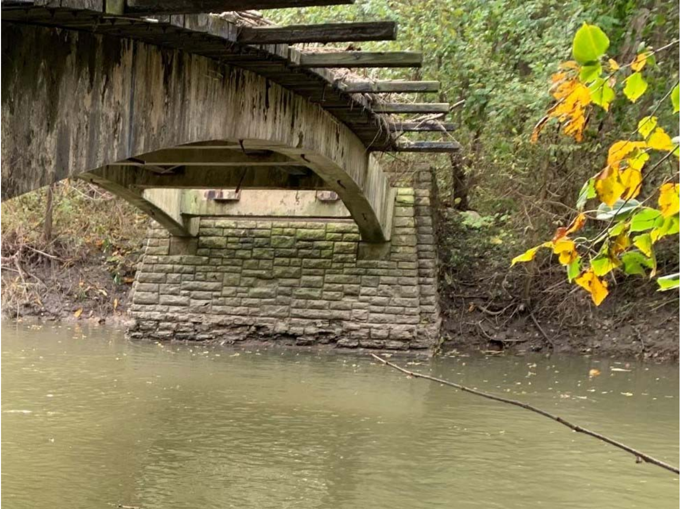
Abutment showing concrete foundation and bank erosion.
