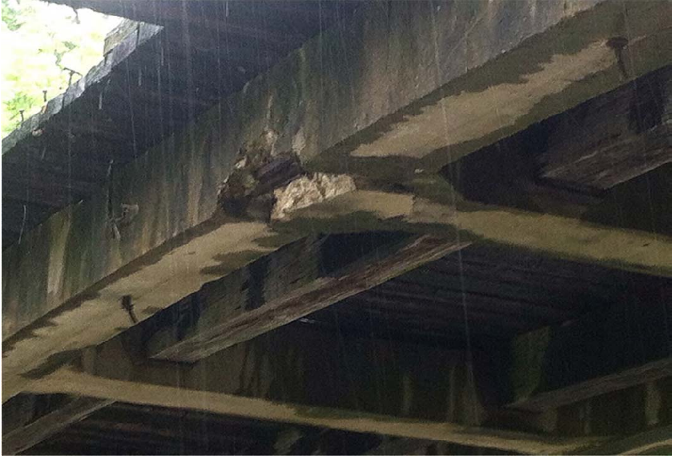
Details of exposed reinforcing bar on face of arch crown
