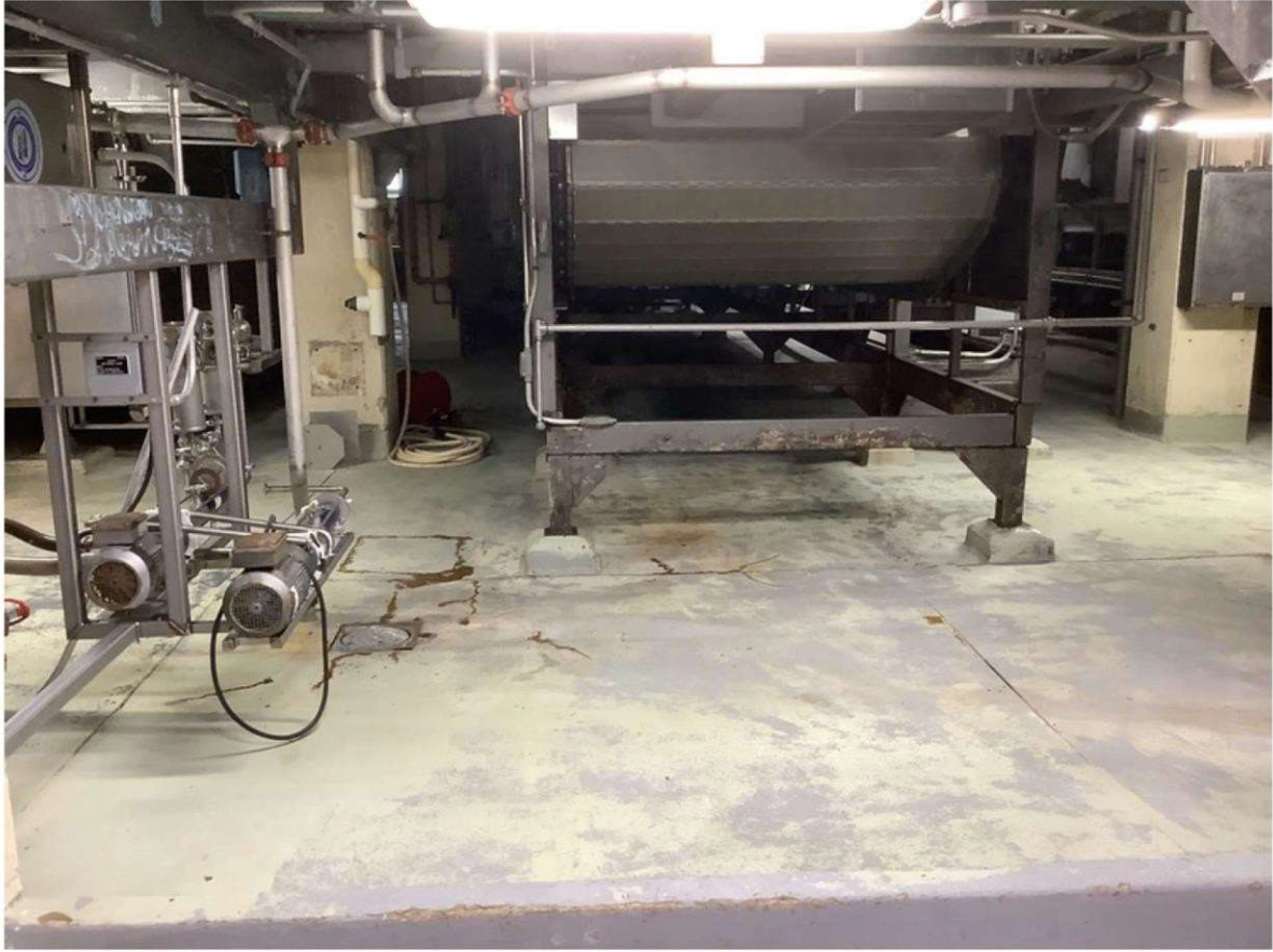
Food processing equipment on the fourth floor
