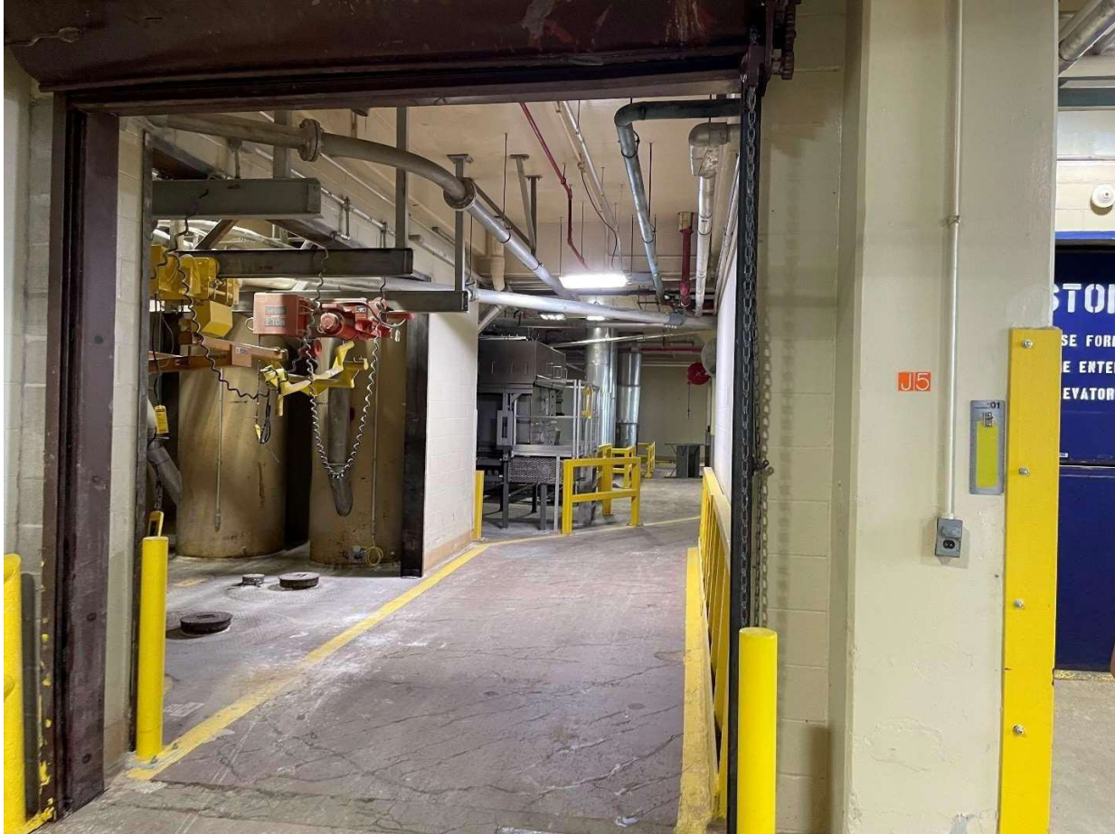
Storage tanks 6 th floor.
