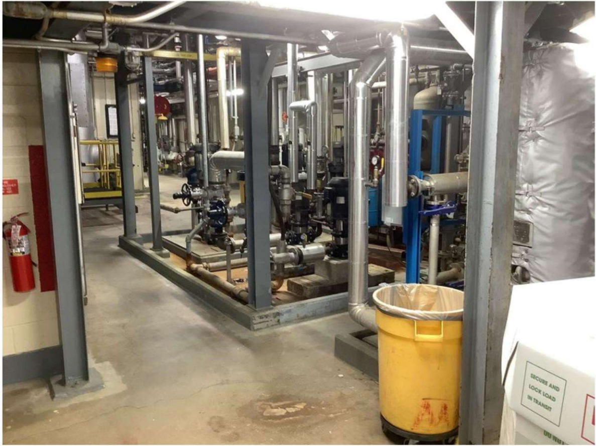
Overview of the boiler room
