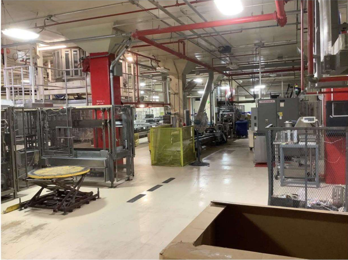
Food manufacturing equipment on the second floor
