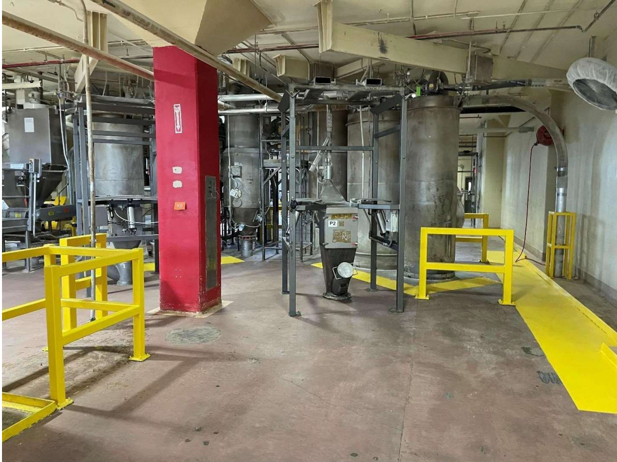
Granola processing storage tanks 6th floor.
