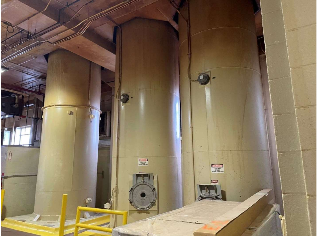
Storage tanks 5 th floor.
