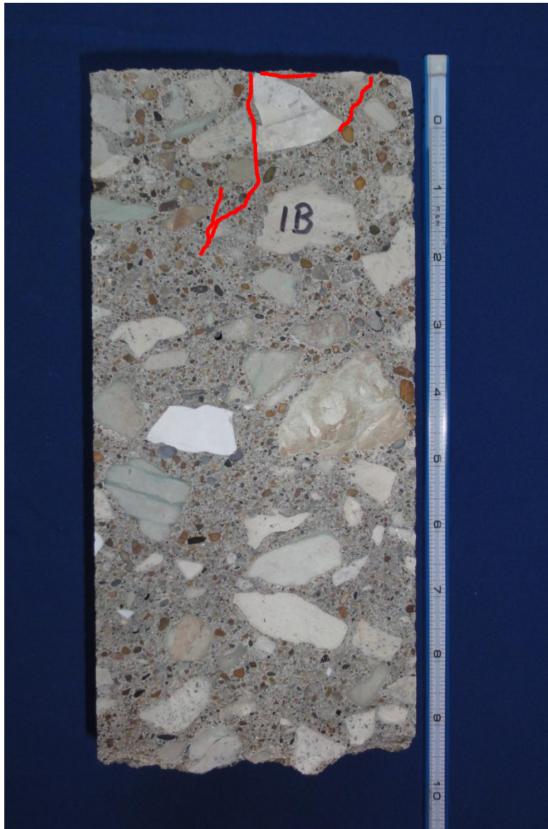
Figure 11. Lapped section of Core 1B. Crack locations are marked in red.
