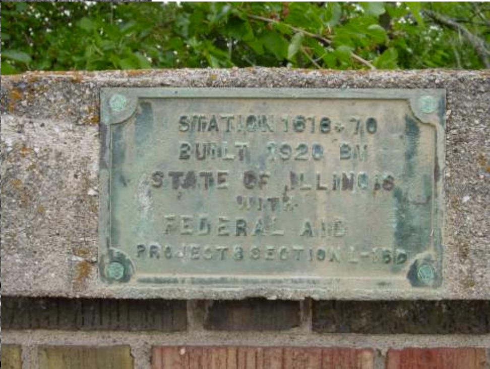
FIG. 73 Girard, IL. Bridge marked Station 1616-70 on Cambridge Rd. Concrete still visible under blacktop. Camera facing west. Photograph by Travis Ratermann, 24 June 2008.
