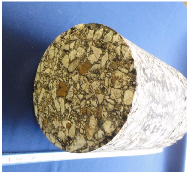
Figure 8. Top surface of the asphaltic core
